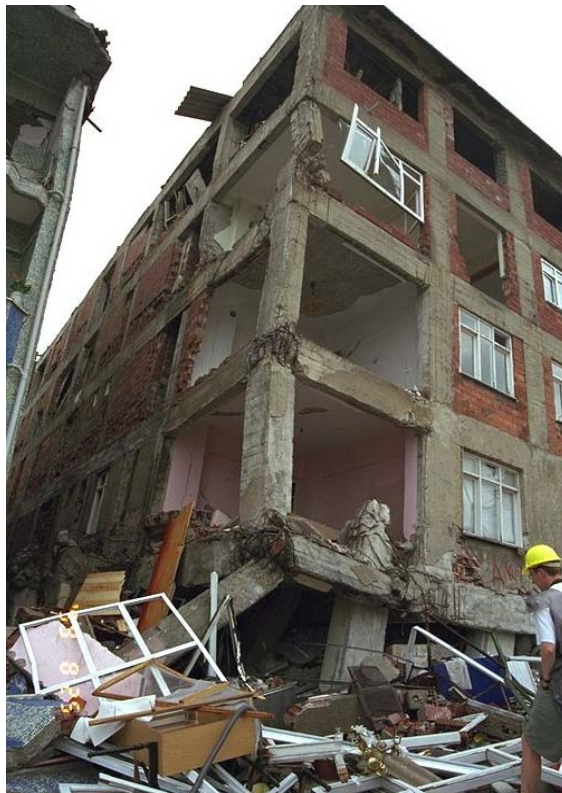
Figure 4-3 Beam-column joint failures in the 1999 Koceali (Turkey) Earthquake (Courtesy of NISEE Earthquake Engineering Online Archive).
