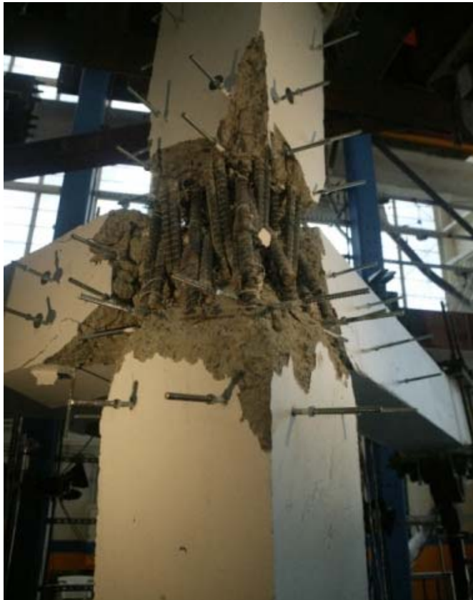
Figure 3-7 Beam-column joint specimen ID 5 tested to failure (Courtesy of NEES Grand Challenge).
