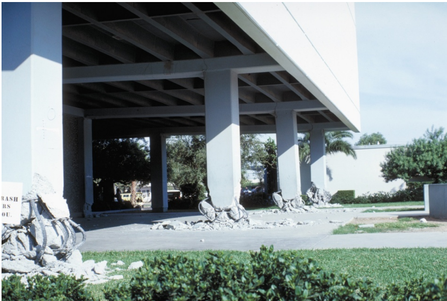
Figure 4-8 Column crushing due to discontinuous wall system, 1979 Imperial Valley Earthquake (Courtesy of NISEE Earthquake Engineering Online Archive).
