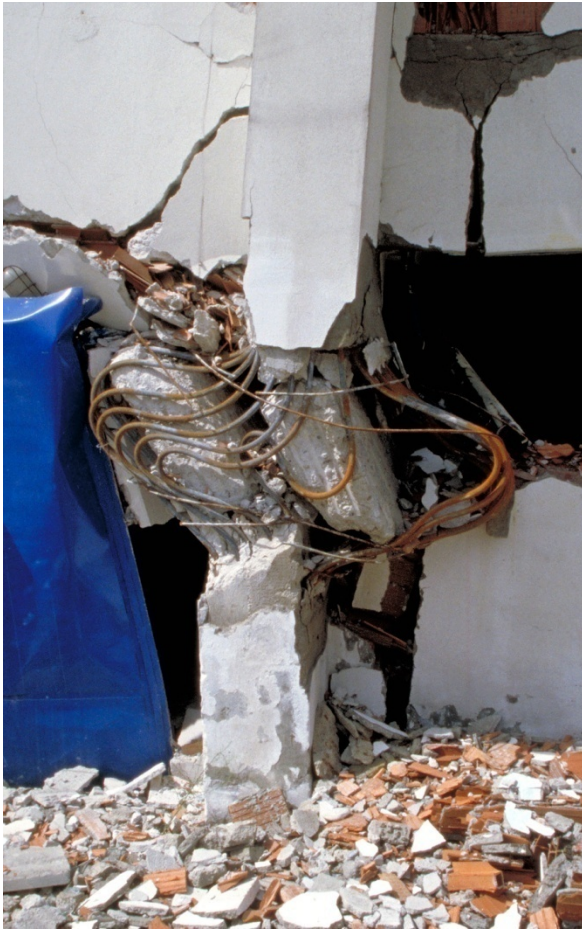
Figure 4-2 Column shear and axial failure in the 1999 Koceali (Turkey) Earthquake (Courtesy of NISEE Earthquake Engineering Online Archive).
