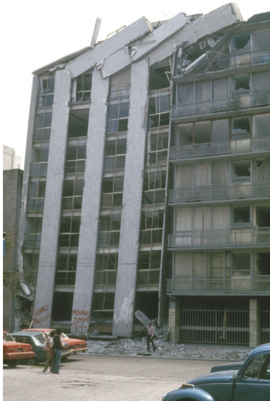
Figure 4-11 Collapse of upper stories due to building pounding in the 1985 Michoacán (Mexico) Earthquake (Courtesy of Jack Moehle).
