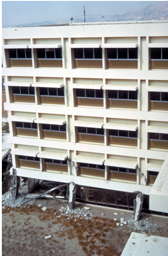
Figure 4-6 Weak-story mechanism, Olive View Hospital, 1971 San Fernando Earthquake (Courtesy of NISEE Earthquake Engineering Online Archive).
