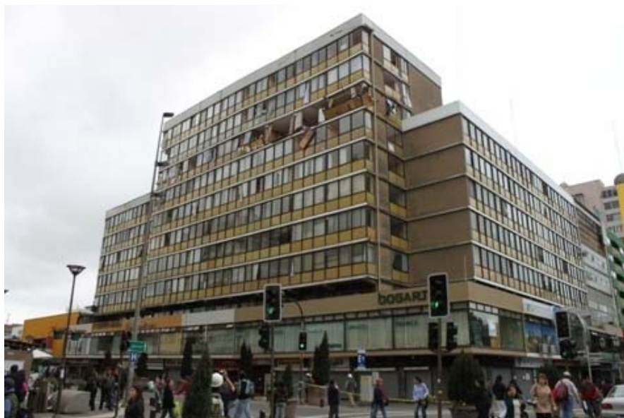
Figure 4-10 Story damage due to vertical irregularity, 2010 Maule (Chile) Earthquake (Courtesy of Jack Moehle).
