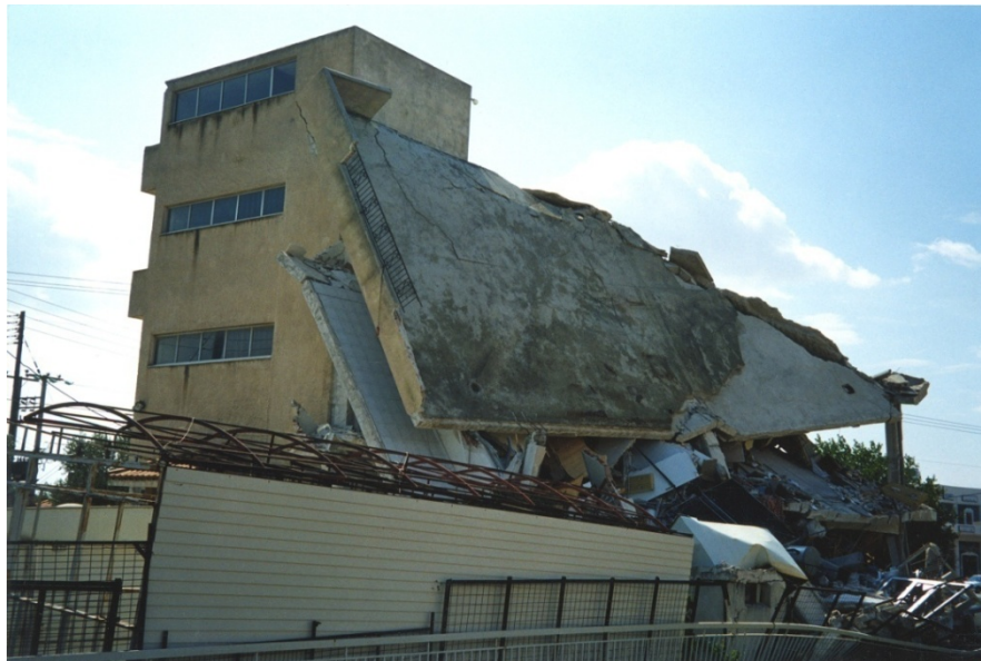
Figure 4-9 Collapse due to torsional drift demands in the 1999 Athens (Greece) Earthquake (Courtesy of NISEE Earthquake Engineering Online Archive).
