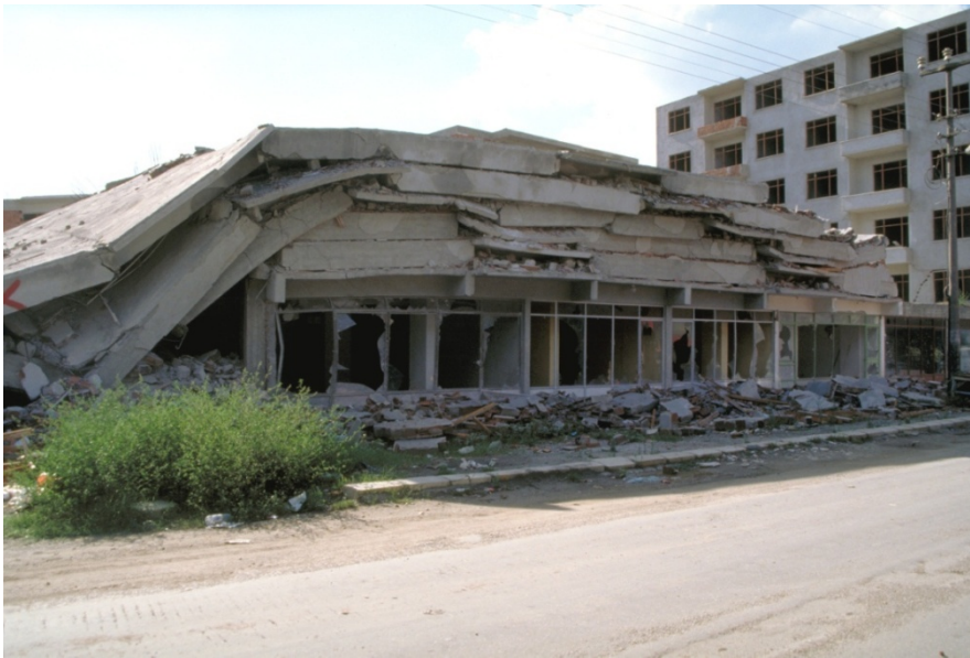
Figure 4-7 Weak frame building collapse in the 1999 Kocaeli (Turkey) Earthquake (Courtesy of NISEE Earthquake Engineering Online Archive).
