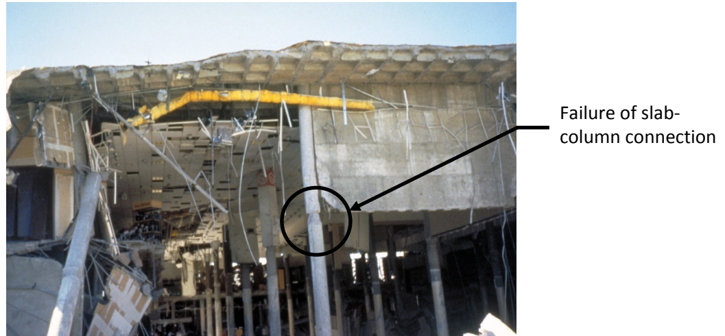
Figure 4-4 Slab-column connection failure in the 1994 Northridge Earthquake (Courtesy of NISEE Earthquake Engineering Online Archive).
