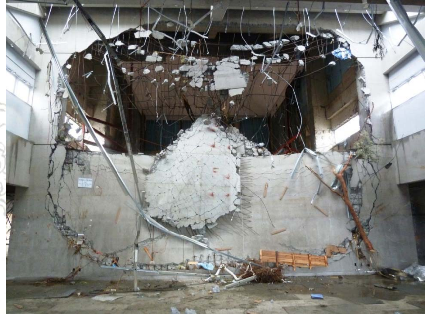
Rikuzentakata Takada Matsubara Building Shear Wall Blowout
