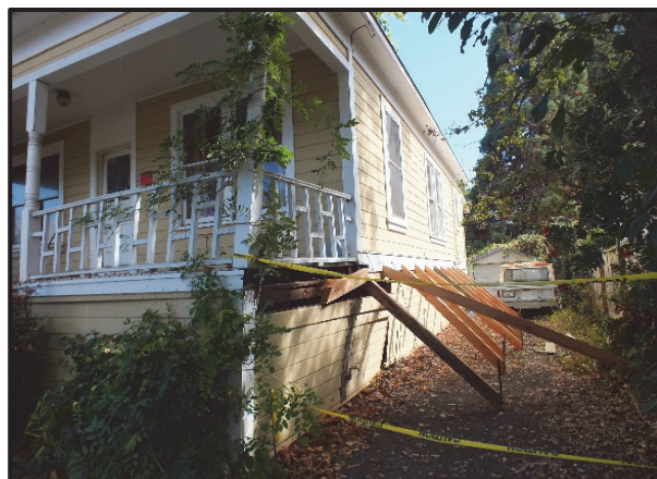
Figure 1: House with cripple walls damaged in the South Napa earthquake. Temporary bracing has been installed to provide stability and prevent collapse. Photo credit: Estructure.
