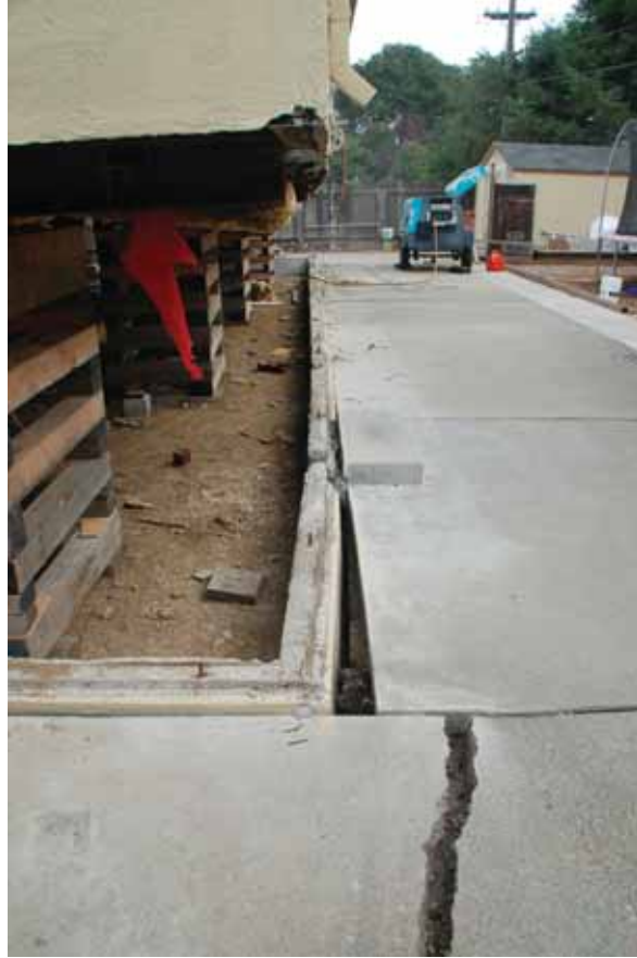
Figure 7-10 Photo showing demolished perimeter foundation and cracks in pavement.
