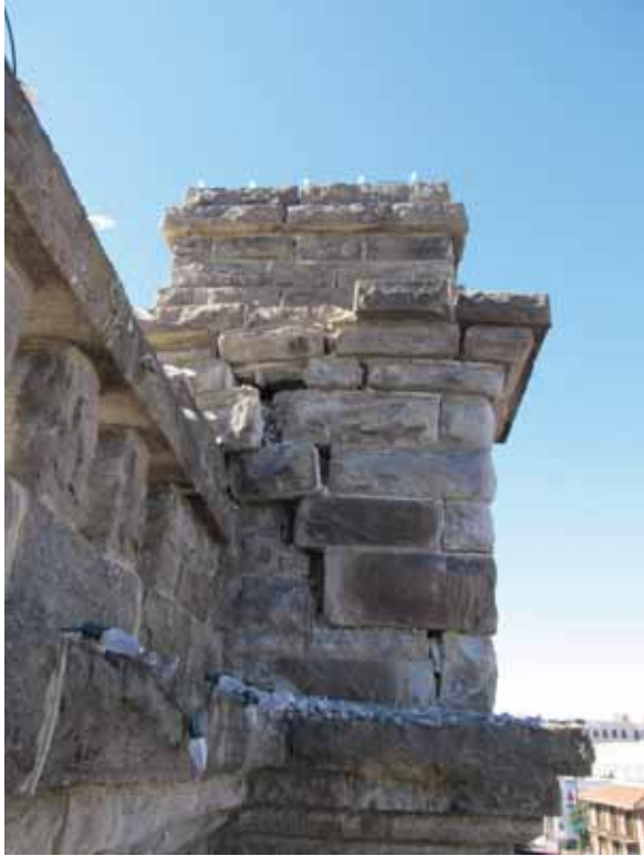
Figure 4-60 Cracking on east side of the tower feature.
