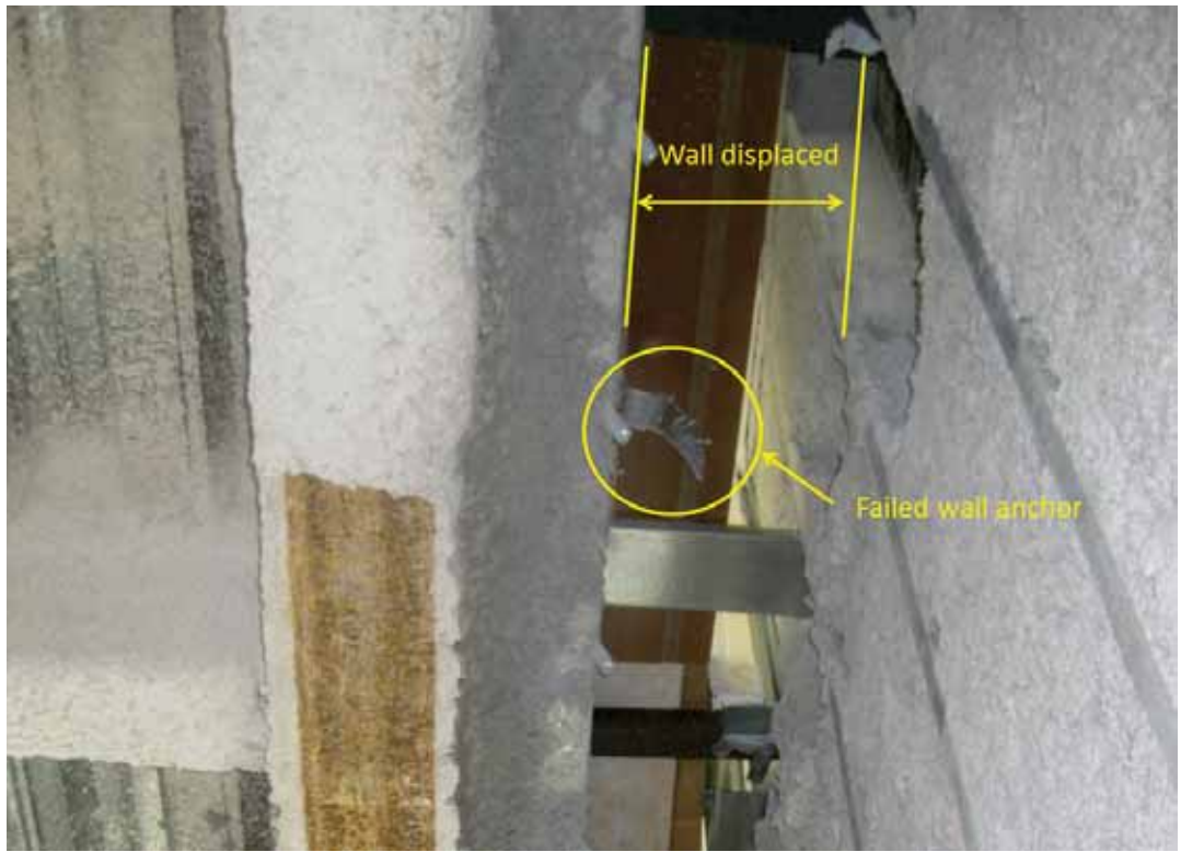
Figure 4-10 Failed wall anchor at bowed wall.
