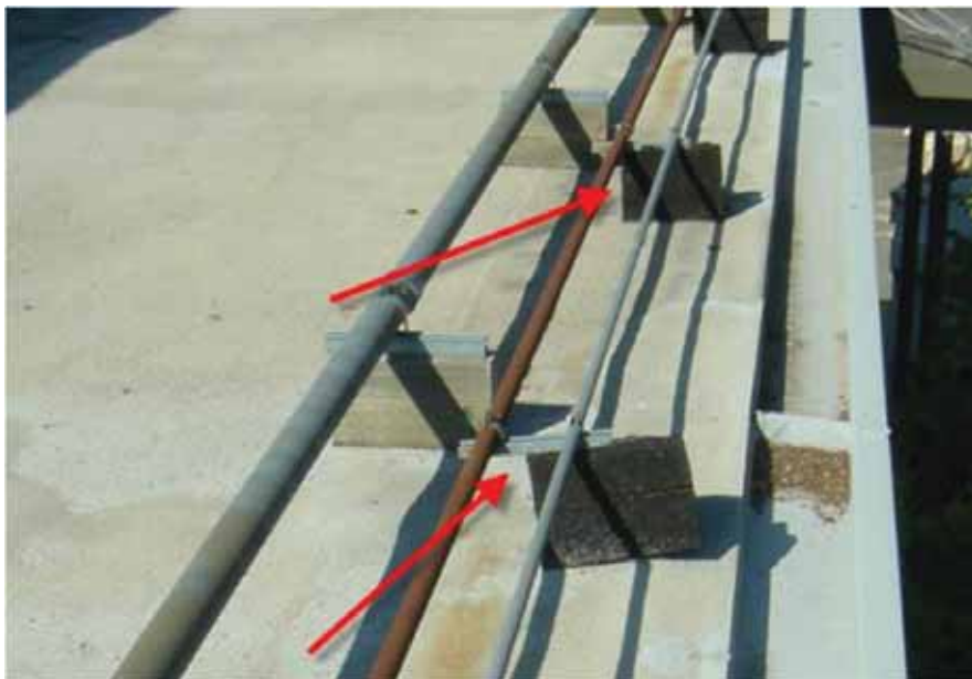
Figure 6-29 Shifted rooftop pipe supports at Silverado Middle School (photo by Quattrocchi Kwok Architects).
