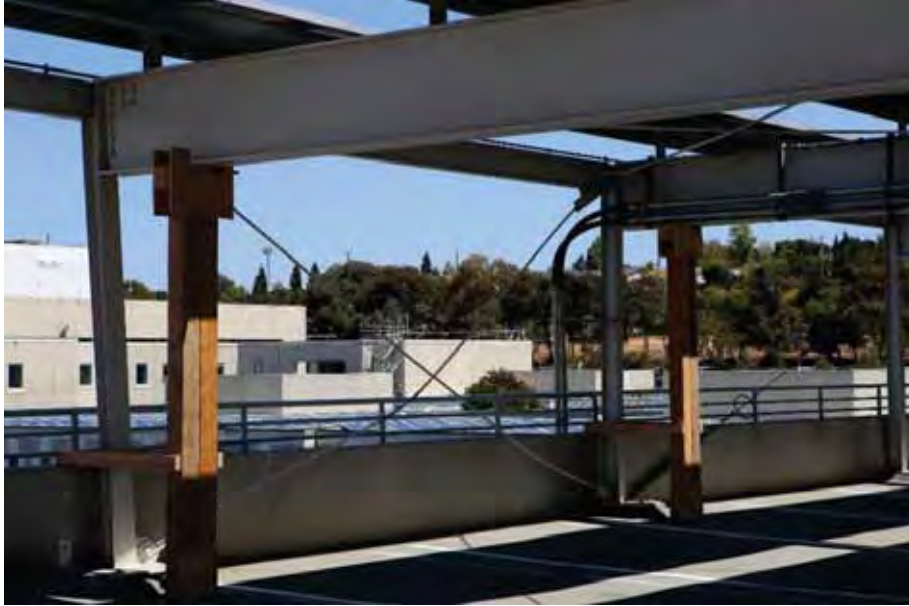
Figure 10-36 Elongated steel X-bracing rods. Note residual drift in the shored column to the left (photo by Jiun-Wei Lai).
