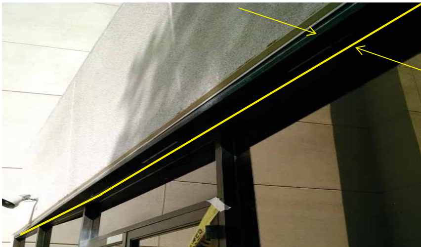
Figure 5-11 South Nursing Wing storefront glazing damage leading to RESTRICTED USE posting at BLD-01656. Yellow line indicates amount of movement in the top track.
