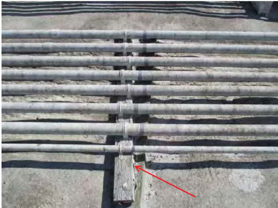
Figure 6-31 Shifted conduit at sleeper support, Harvest Middle School (photo by Quattrocchi Kwok Architects).
