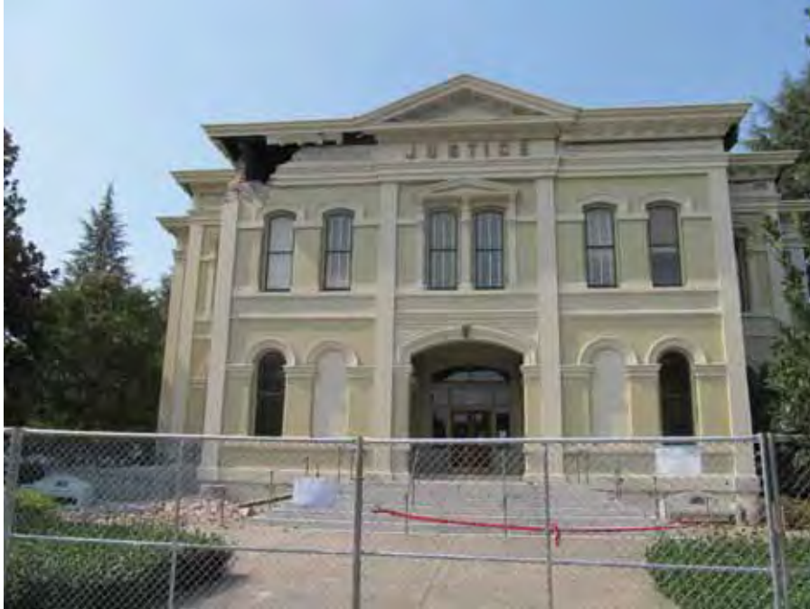
Figure 4-47 East façade of historic URM courthouse. Note fallen bricks below the damaged portion at the top of the wall.
