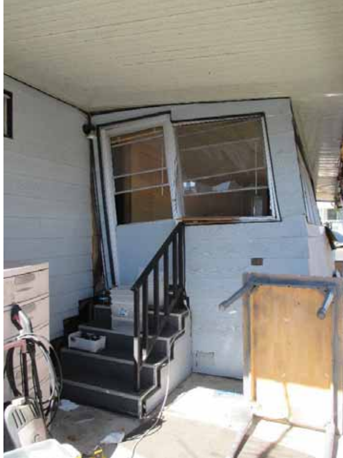
Figure 8-16 Add-on porch structure severely damaged by the earthquake.
