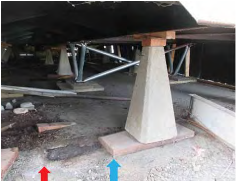
Figure 8-22 Extent of home sliding. Red arrow is initial wood board position, blue arrow is final position. ERBS can be observed in the background.
