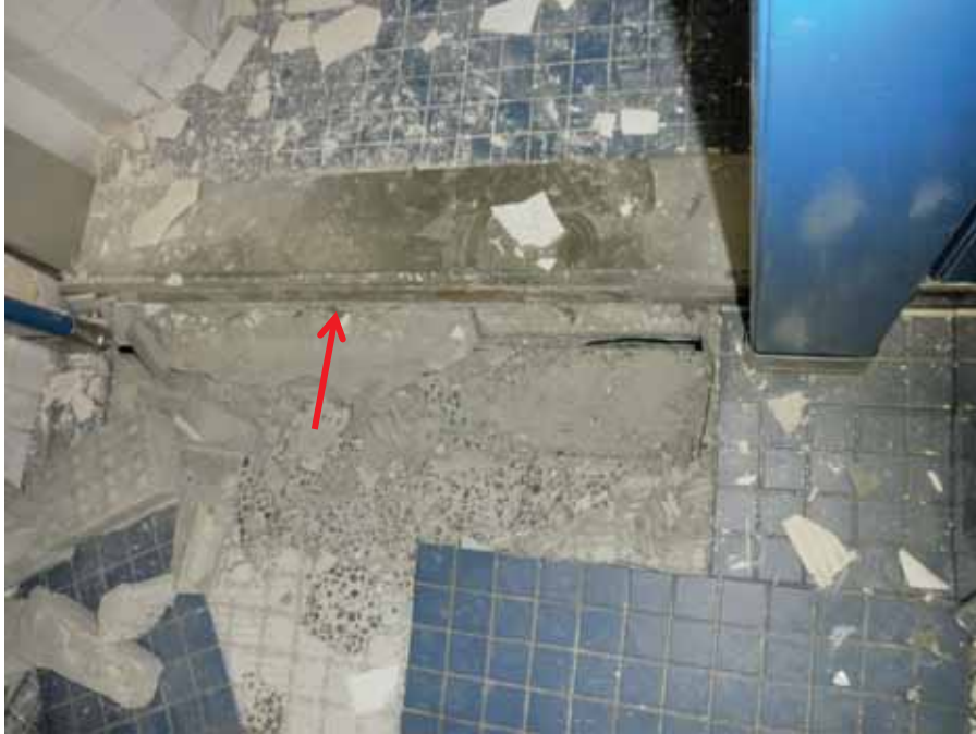
Figure 4-39 Floor finish damage due to pounding at the seismic joint indicated by the arrow.
