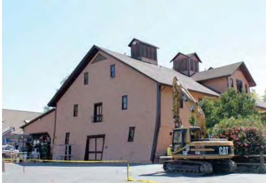
Figure 9-3 Historic timber-framed winery building with large residual drift at the ground floor.
