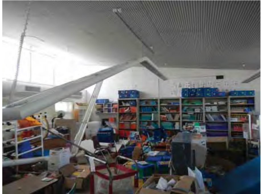
Figure 6-2 Damaged light fixtures in classroom at Pueblo Vista Elementary School (photo by Quattrocchi Kwok Architects).
