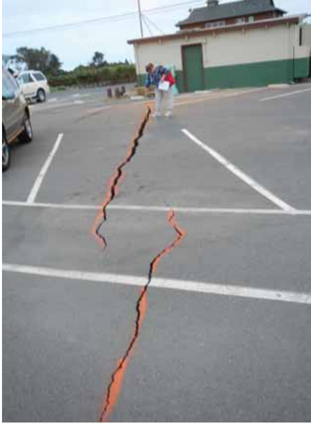
Figure 6-36 Cracks in asphalt parking lot at Stone Bridge School (photo by Quattrocchi Kwok Architects).
