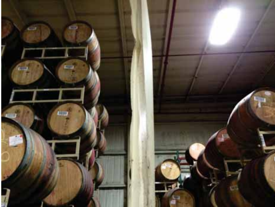
Figure 9-4 Steel columns damaged by impact of barrels.
