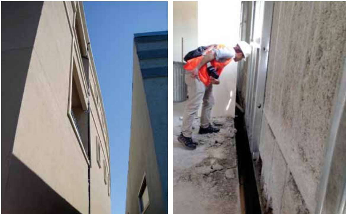
Figure 4-8 Bowed wall separated from floor (photo on right from Lauren Biscombe).
