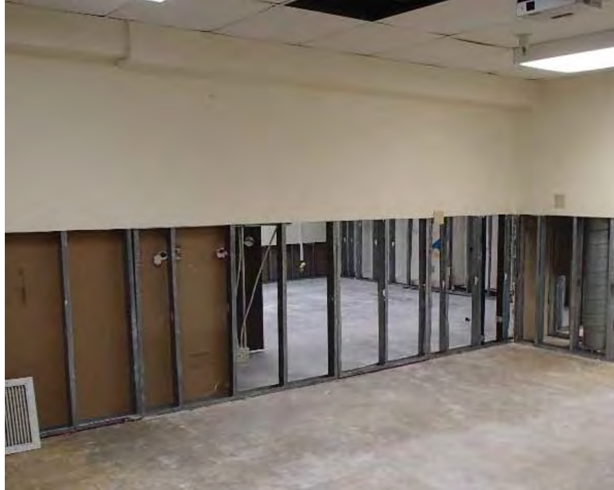
Figure 10-7 Gypsum wallboard was removed from partition walls where water damage from a broken sprinkler head occurred.
