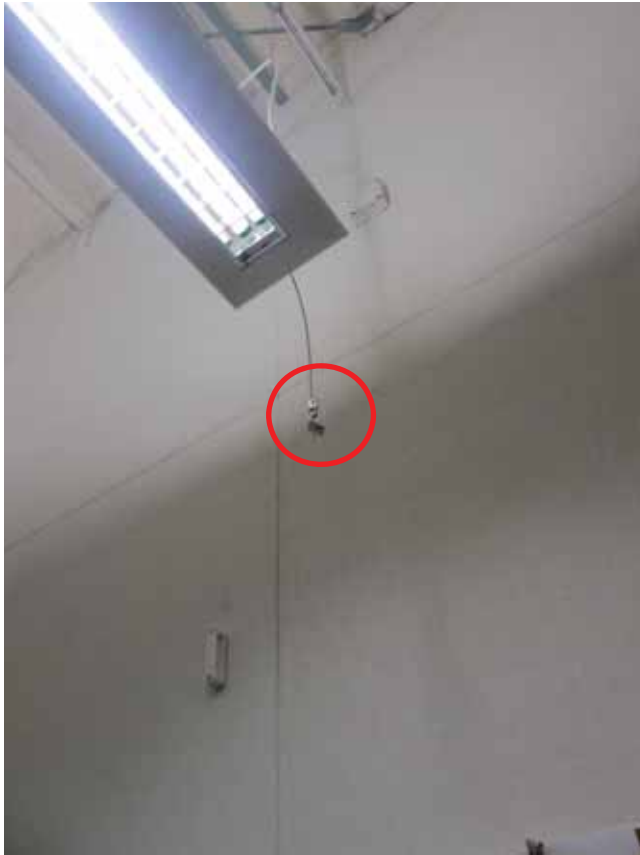
Figure 6-8 Bracing wire pulled out of wall at Harvest Middle School (photo by Quattrocchi Kwok Architects).
