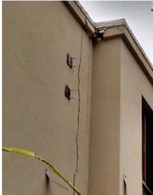
Figure 5-26 Cracking along the separation joint between BLD-01666 and BLD-01667 at the roof penthouse.
