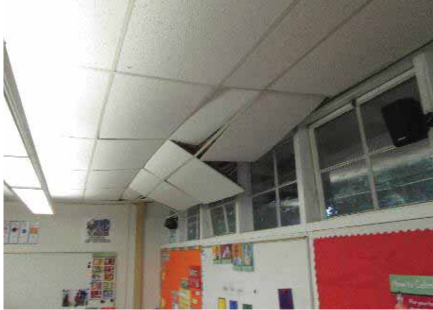
Figure 6-19 Damage to suspended acoustic tile ceiling in Napa Junction Elementary School (photo by Quattrocchi Kwok Architects).
