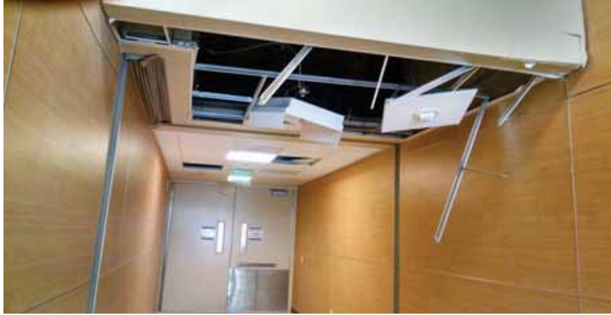
Figure 5-7 Third floor ceiling damage in BLD-05323 corridor link.
