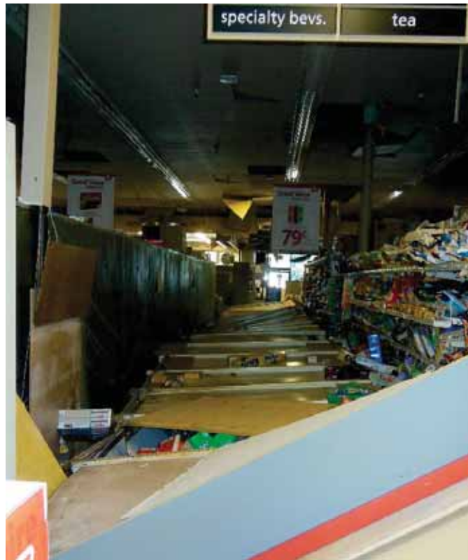
Figure 10-29 Unanchored fixtures overturned in aisle.
