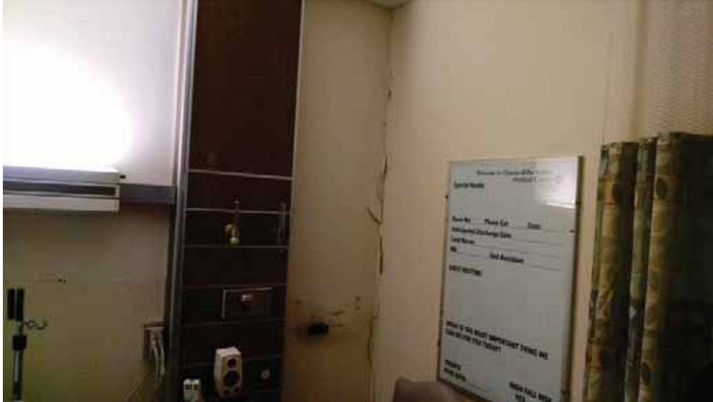
Figure 10-9 Damage to gypsum wallboard at corner (photo from OSHPD).
