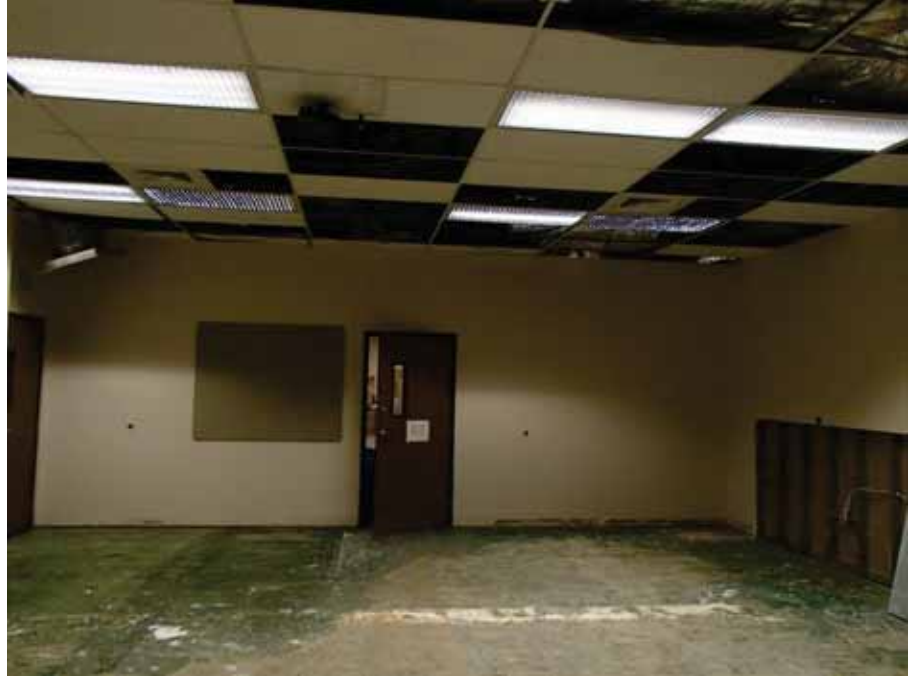
Figure 10-14 Acoustic ceiling where tiles fell in an office building.
