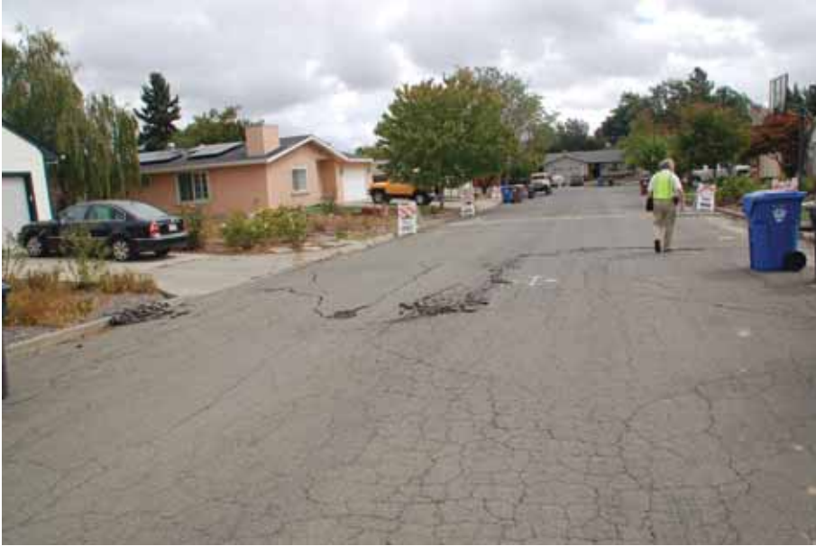
Figure 7-9 Surface rupture observed on street.
