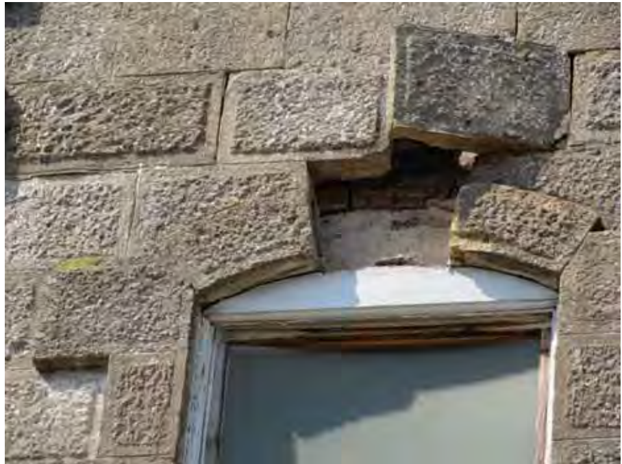
Figure 4-78 Loose stone cladding over window at front façade.
