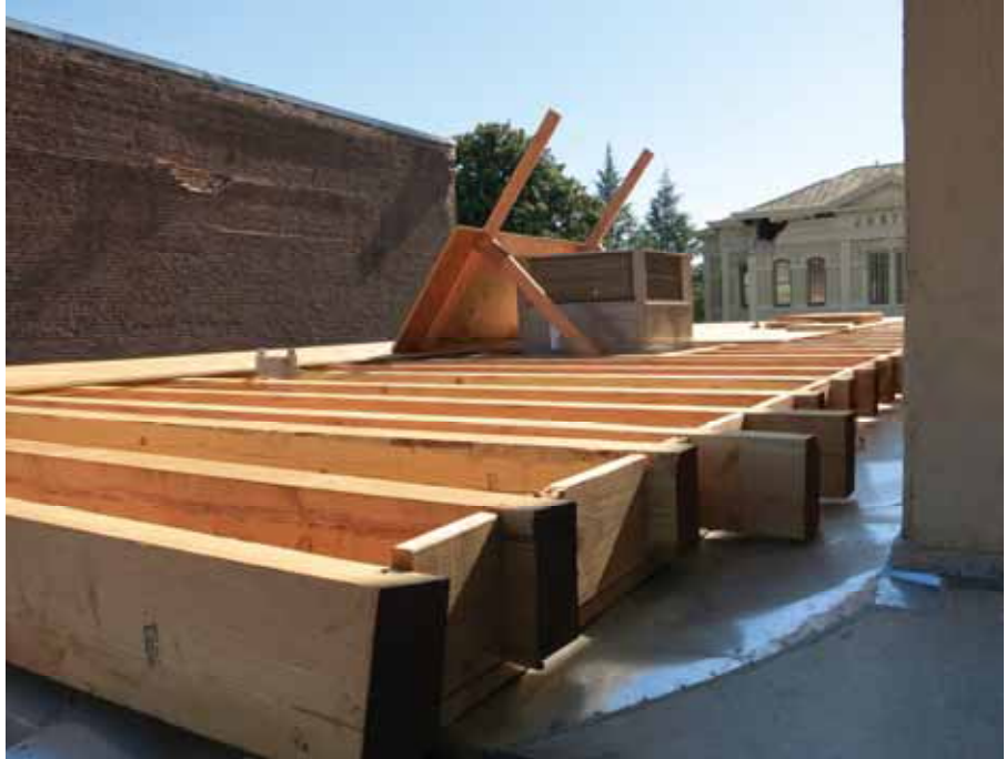
Figure 4-50 Wooden barrier constructed on the roof a building neighboring a masonry wall at risk of collapse.
