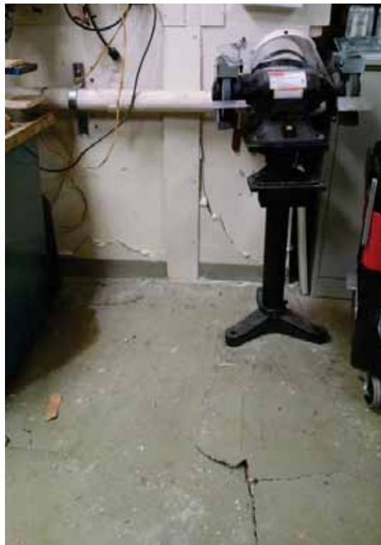
Figure 5-27 Cracking of the 1/2 inch to 1 inch thick topping slab over original roof slab inside the roof penthouse along the separation joint.
