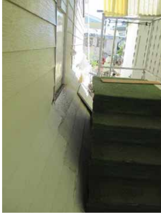
Figure 8-26 Entry stairs at Napa Valley MHP home that displaced significantly to the east.
