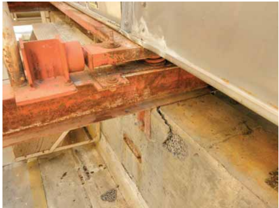
Figure 4-41 Anchor failure, rooftop cooling tower 1974 wing.
