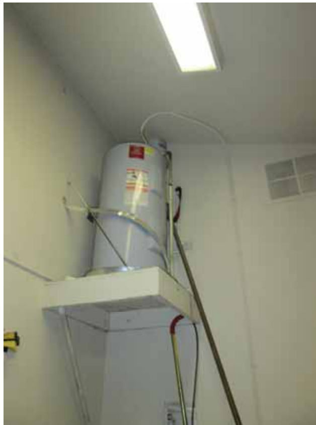
Figure 6-23 Failed earthquake restraining strap on water heater (photo by Quattrocchi Kwok Architects).
