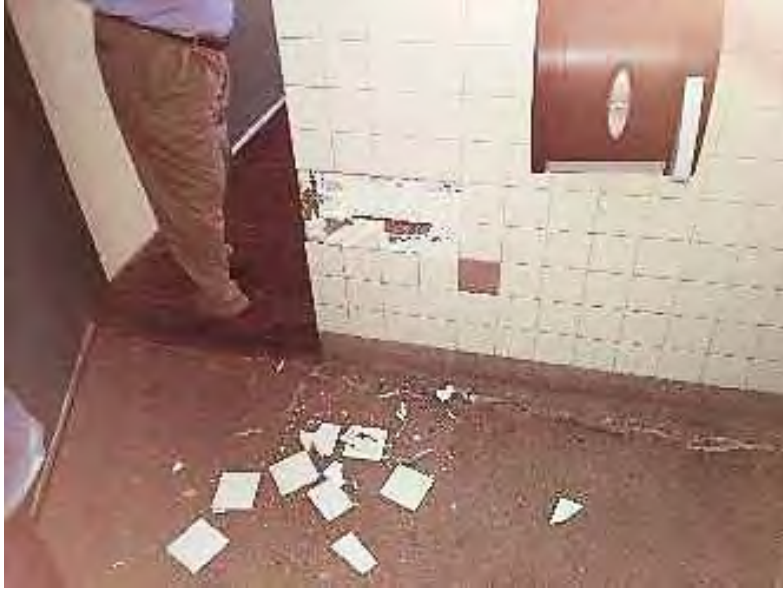
Figure 6-21 Dislodged adhered tile in Harvest Middle School (photo by Quattrocchi Kwok Architects).
