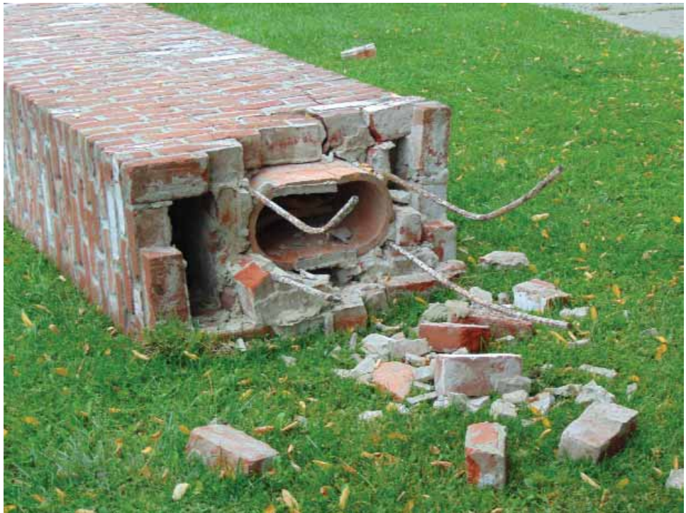
Figure 7-24 Photo of chimney laying on front yard of home (photo from Janiele Maffei).
