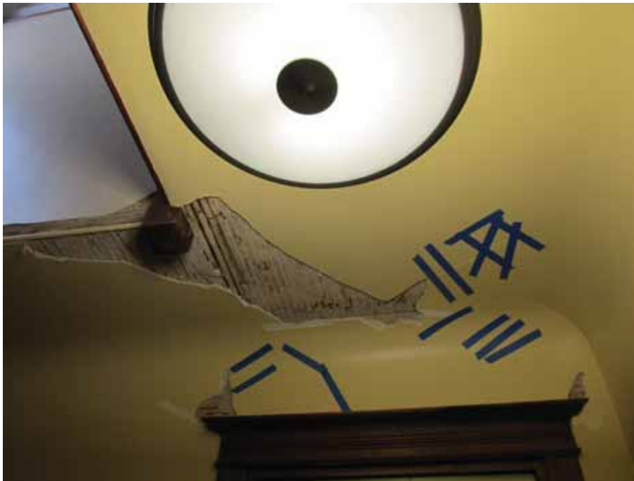
Figure 4-63 Lath and plaster ceiling damage and temporary taping at cracks and spalls.
