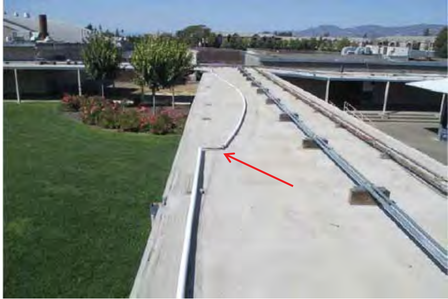
Figure 6-34 Broken PVC conduit at Redwood Middle School (photo by Quattrocchi Kwok Architects).
