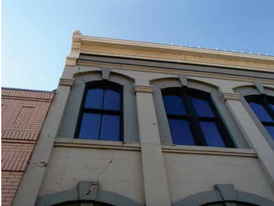
Figure 4-65 Cracking in URM on south façade.
