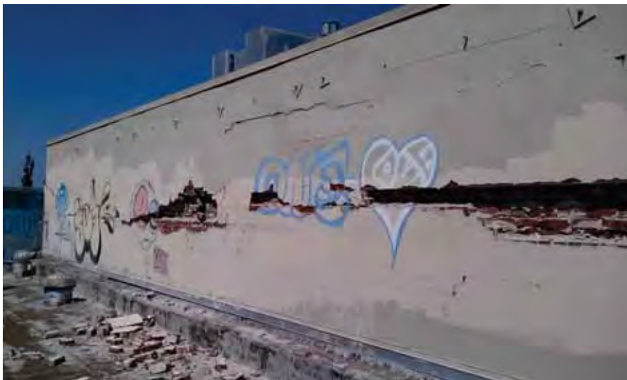
Figure 4-66 URM damage, west elevation (photo from Chris Jonas, ZFA Structural Engineers).
