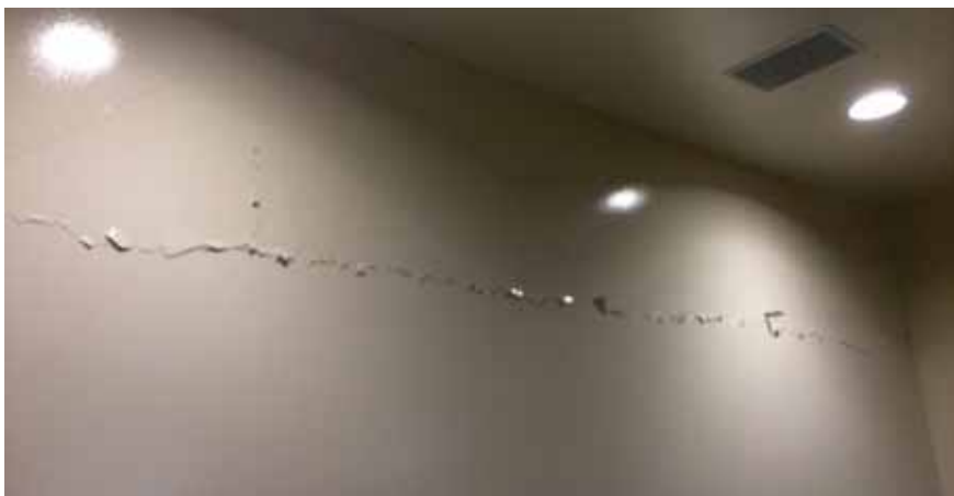
Figure 5-6 Cracked gypsum board wall in BLD-05309.
