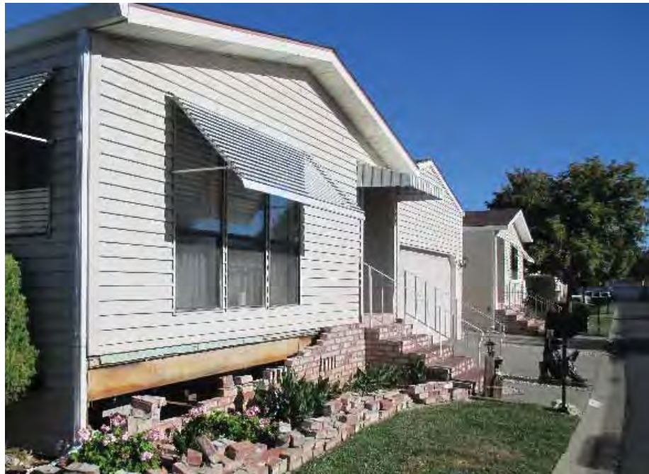
Figure 8-19 Damage to brick masonry skirt wall.
