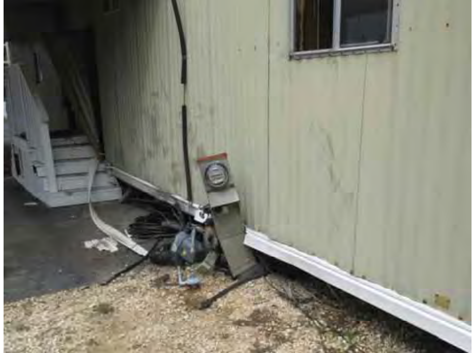
Figure 8-23 Manufactured home that slid and fell onto its utility hookup.
