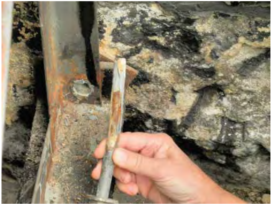
Figure 4-87 Failed wall anchor, north elevation.
