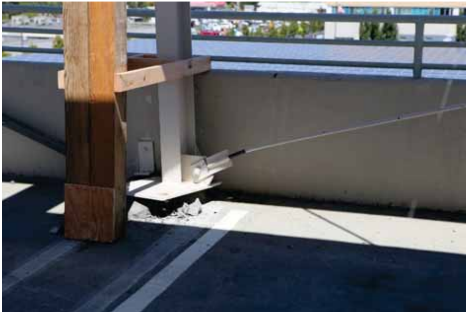
Figure 10-37 Possible plastic strain of steel rod X-bracing adjacent to gusset plate. Column has twisted due to eccentric configuration of rod bracing and anchor bolts. Anchor bolt breakout or grout crushing occurred beneath column baseplate (photo by Jiun-Wei Lai).
