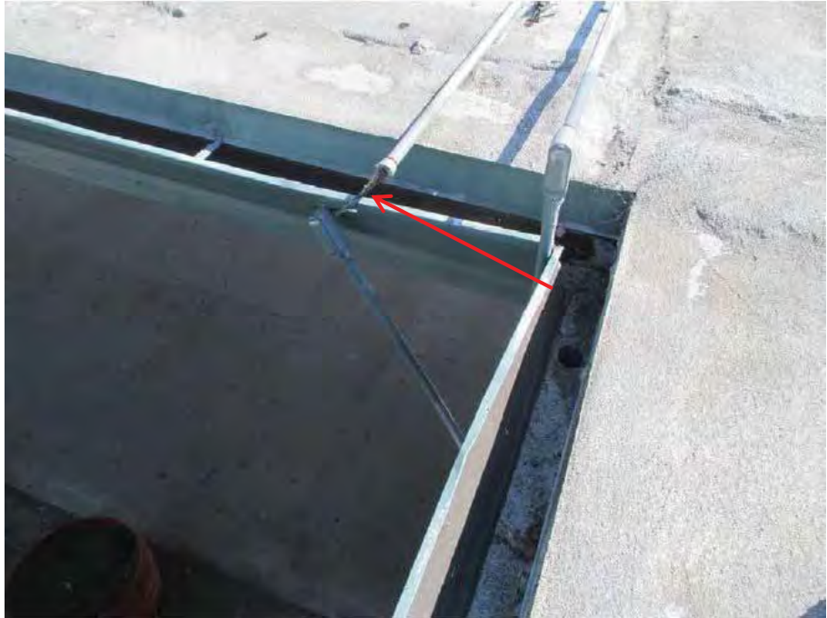
Figure 6-30 Exposed wires at failed conduit fitting, Harvest Middle School (photo by Quattrocchi Kwok Architects).
