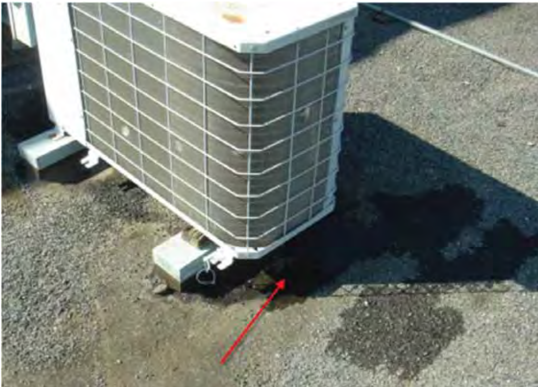
Figure 6-25 Shifted rooftop condensate unit at Redwood Middle School (photo by Quattrocchi Kwok Architects).
