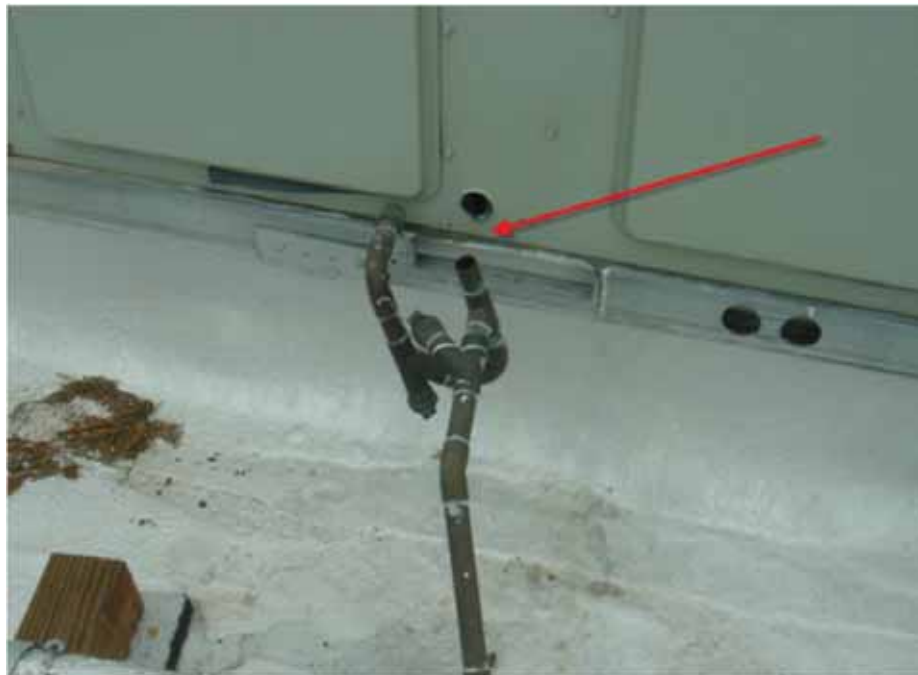
Figure 6-27 Broken condensate connection at air conditioning unit, Redwood Middle School (photo by Quattrocchi Kwok Architects).
