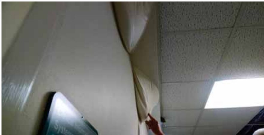
Figure 5-9 Evidence of water leak in corridor of BLD-01650 (paint stretched to contain water).
