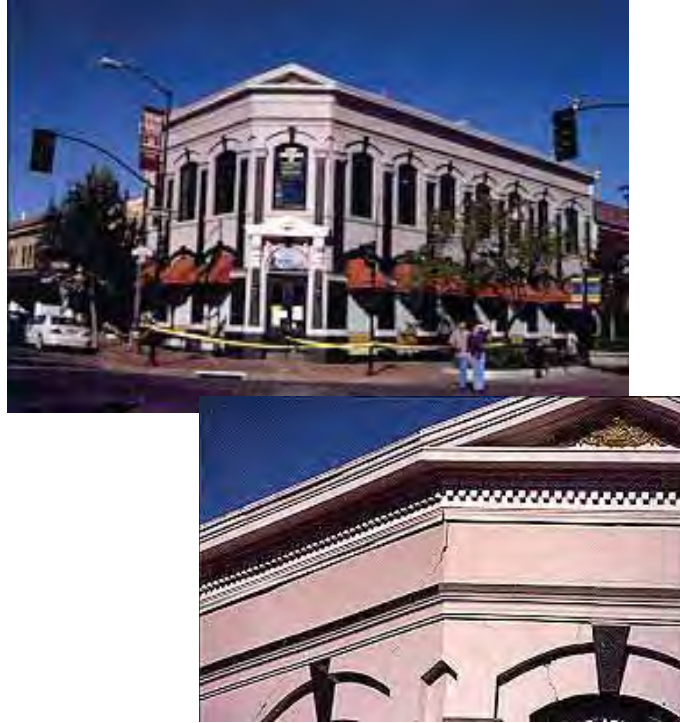
Figure 4-67 Photo of Building J4 and detail of damage after the 2000 Yountville earthquake (PEER, 2000).
