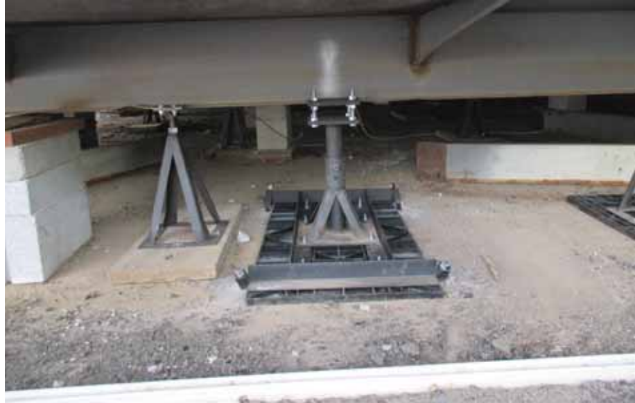
Figure 8-7 Steel pier system with anchor rods to the ground.
