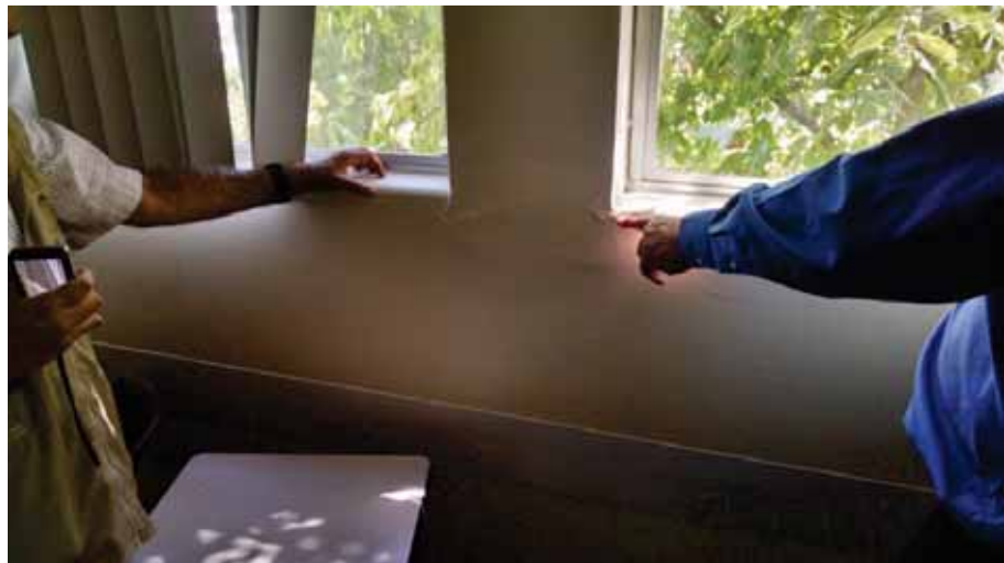
Figure 5-4 Cracked concrete wall piers in BLD-01650.
