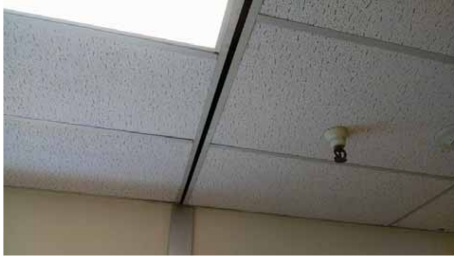
Figure 5-12 Movement at seismic joint between BLD-01652 and BLD-01650 Main Hospital.
