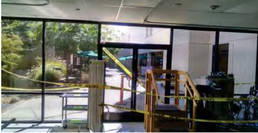
Figure 5-10 South Nursing Wing storefront glazing damage leading to entrance posted RESTRICTED USE at BLD-01656.
