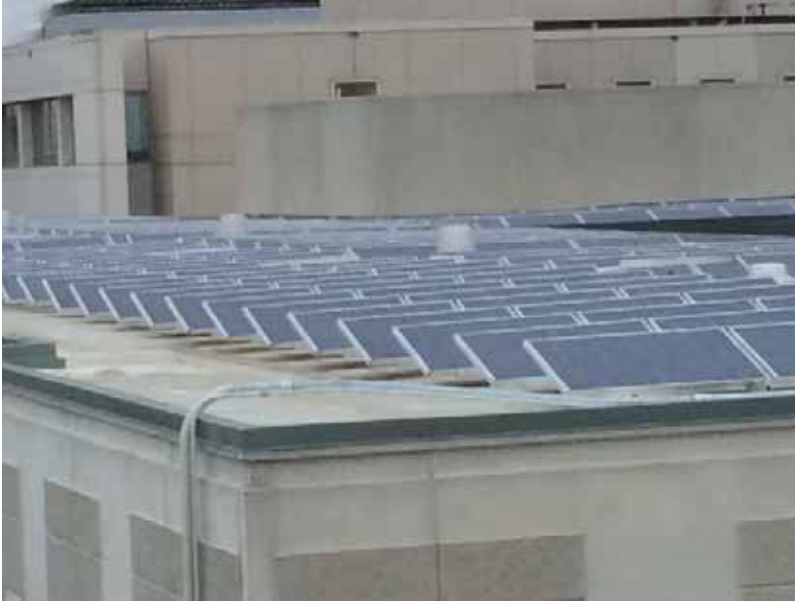
Figure 10-39 Low-profile unattached (ballast-only) solar array on roof of medical office building (photo from Kaiser Permanente). No damage was reported.
