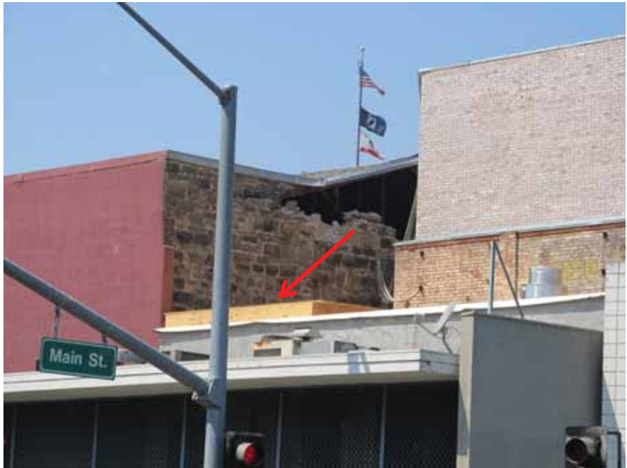
Figure 4-51 Failure of stone masonry east wall. Red arrow indicates wood barrier protecting adjacent property from falling stones.
