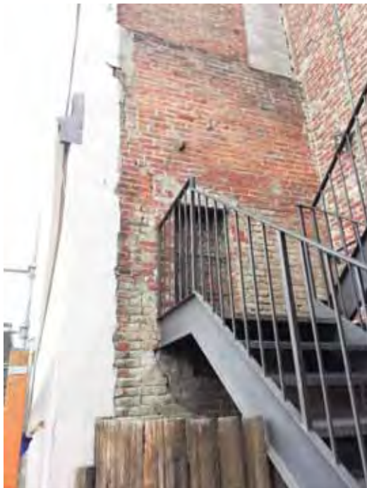
Figure 4-83 Southeast corner, damage to URM wall due to interaction with steel stair.
