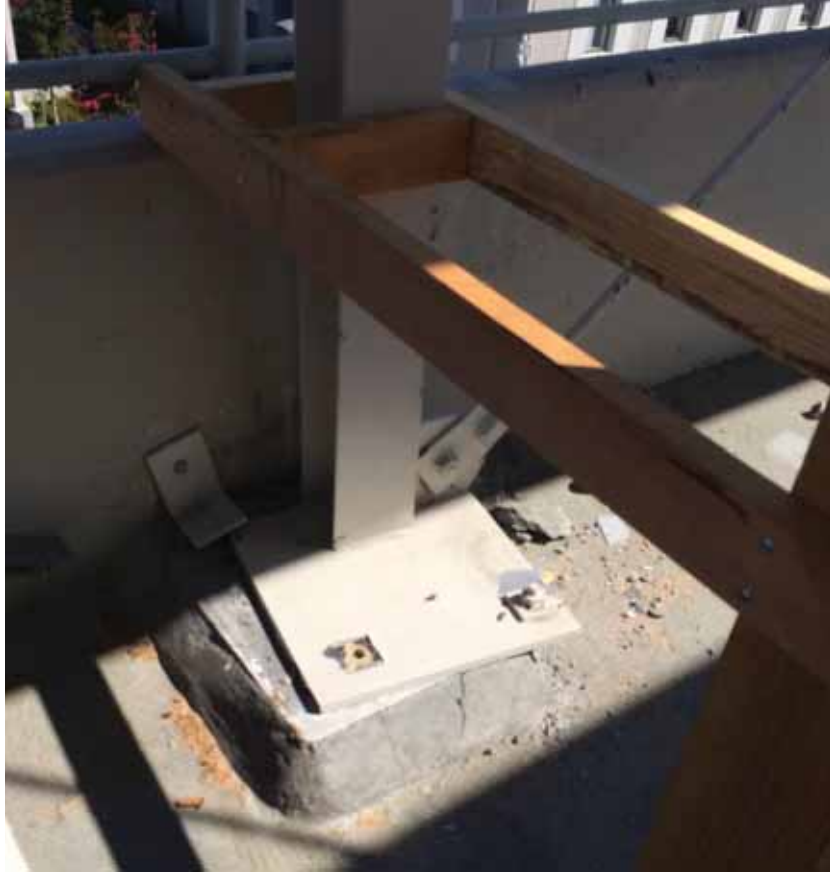
Figure 10-38 Clip angle is anchored to the concrete wall but not attached to column baseplate. Note eccentricity between the X-bracing rod and the column anchor bolts (photo by John Silva).
