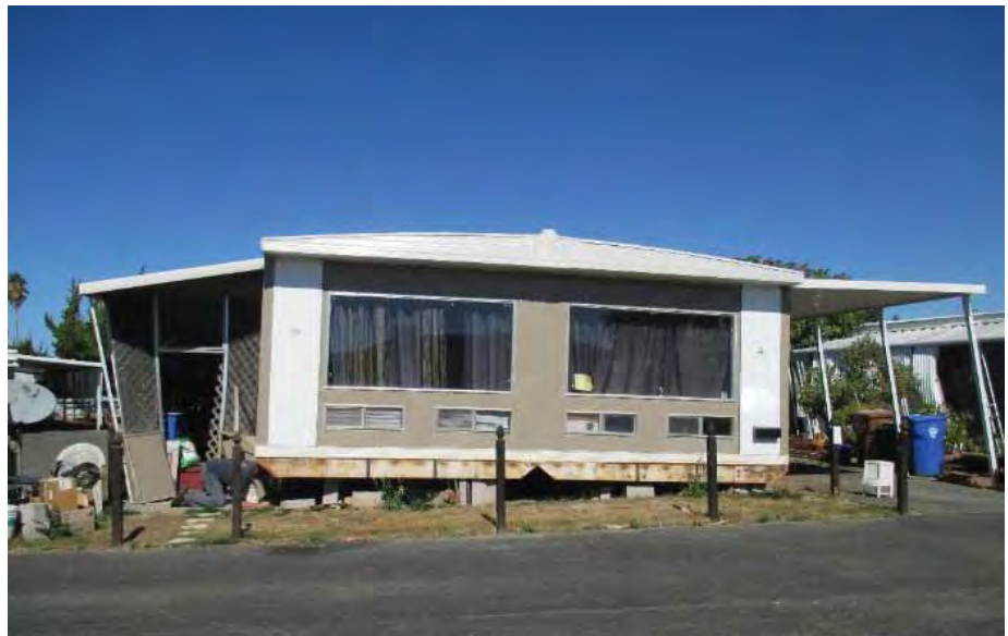
Figure 8-13 Home dropped from masonry gravity pier supports.
