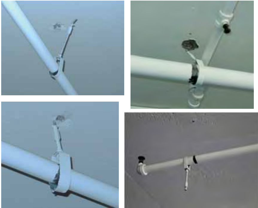
Figure 10-25 Failures of powder driven fasteners. Bottom right photo is from PEER (2014).
