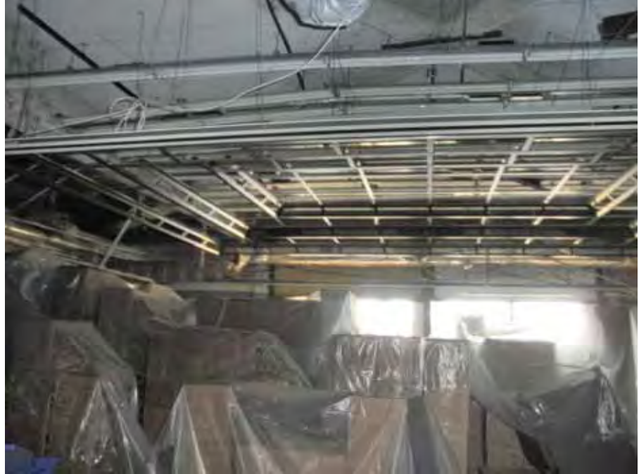
Figure 4-34 Ceiling removed due to water damage, third floor.
