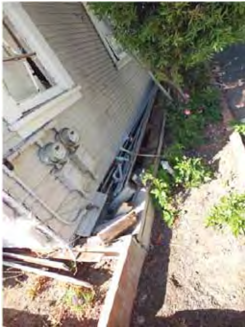
Figure 7-17 Collapsed cripple wall.
