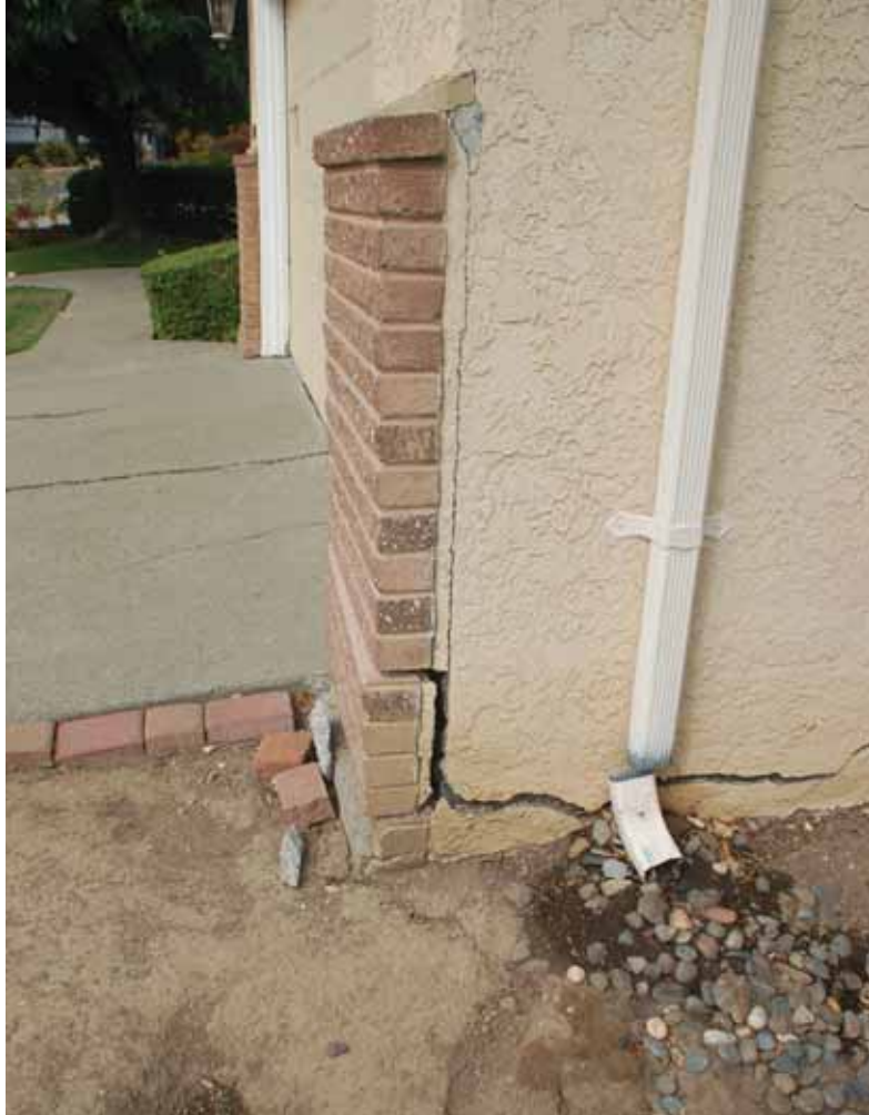
Figure 7-4 Crack continuing around the base of structure.
