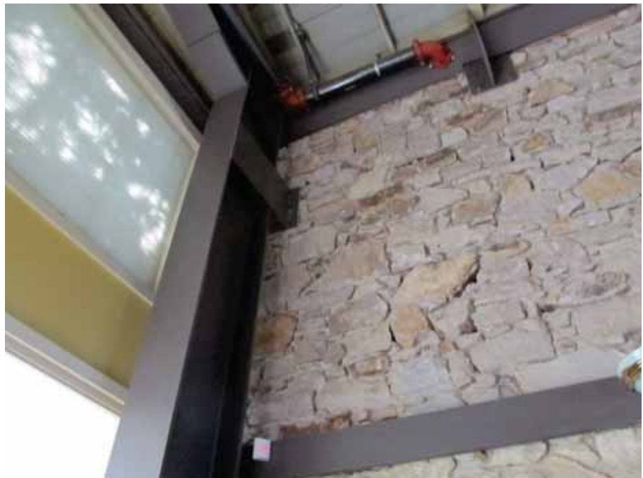
Figure 4-73 Diagonal cracks in stone wall.
