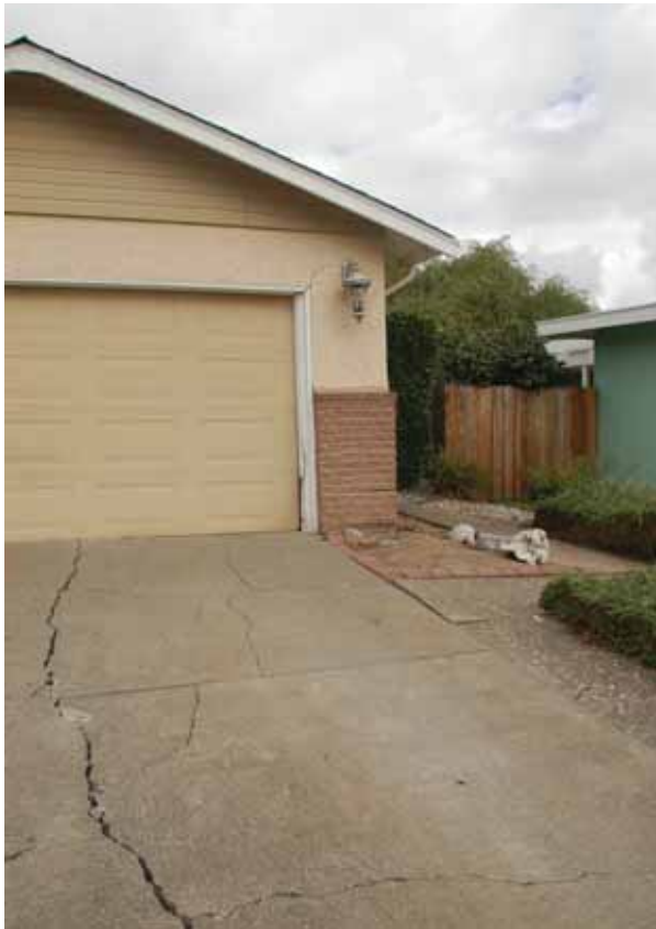
Figure 7-3 Crack running through the street and up the driveway.
