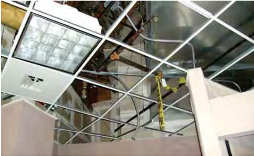
Figure 10-22 Sprinkler piping in close proximity to HVAC components.
