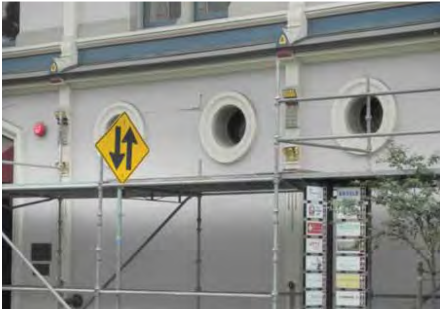
Figure 4-82 Minor cracking in URM wall, north elevation.
