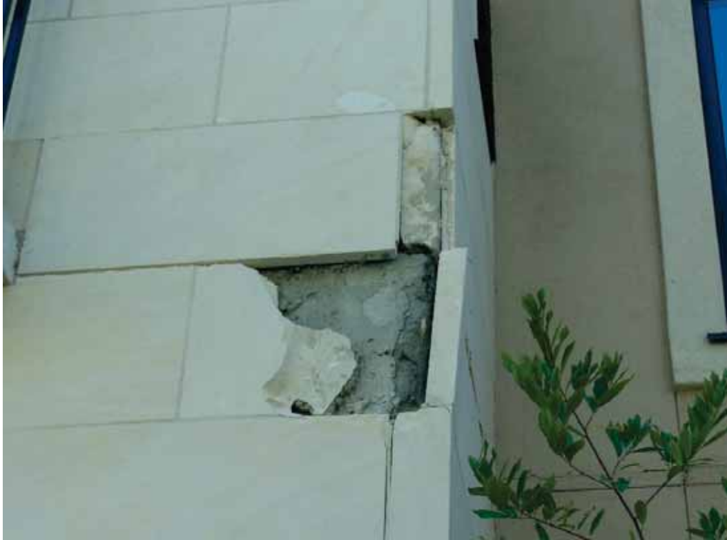
Figure 4-15 Adhered veneer damaged during the earthquake.
