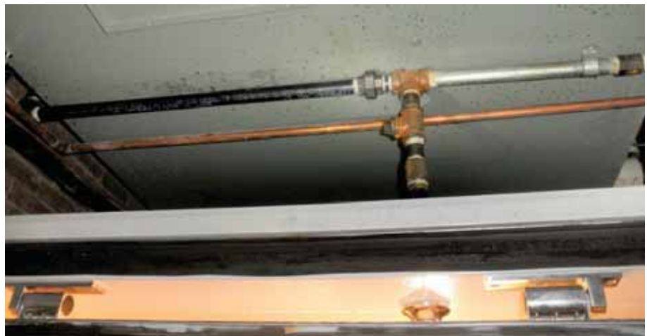
Figure 10-21 Repaired condition of a failed pipe at threaded connection that resulted in flooding of the first floor restaurant.
