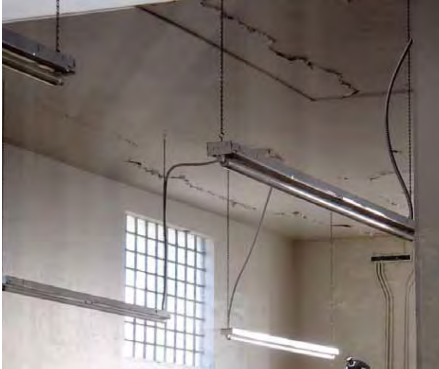
Figure 10-13 Cracking and spalling of a plaster ceiling in an older reinforced concrete building in downtown Napa.
