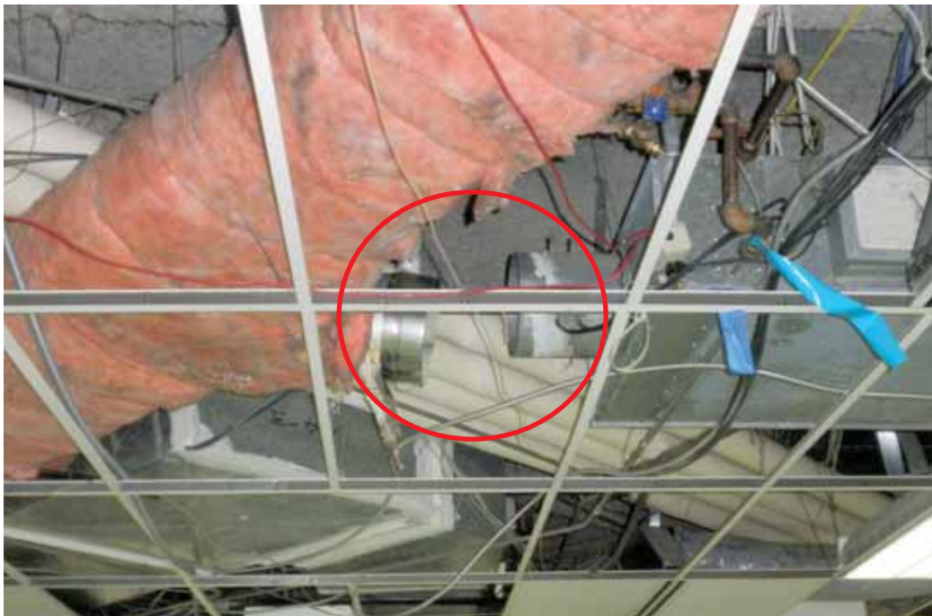
Figure 4-33 Ceiling and duct damage. The duct separated from the in-line HVAC unit to the right.
