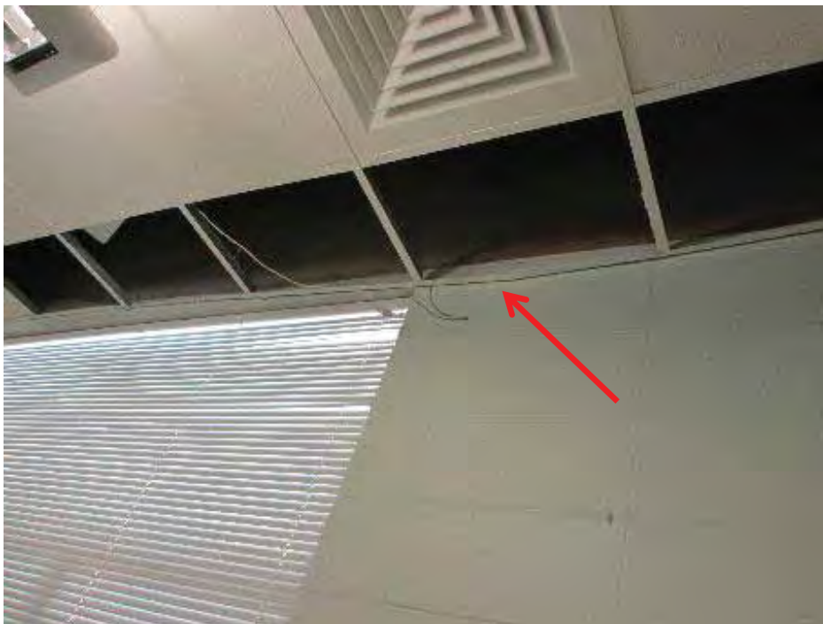
Figure 6-18 Dislodged tiles and bent edge angle in a Silverado Middle School classroom (photo by Quattrocchi Kwok Architects).
