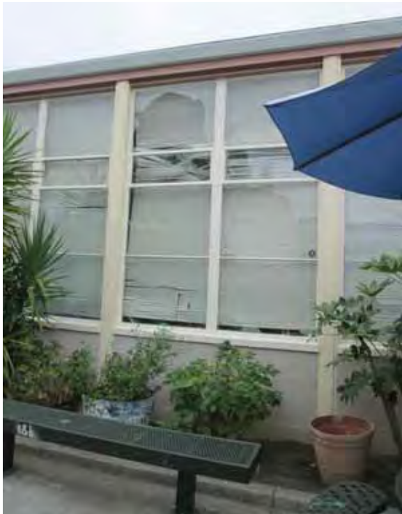
Figure 6-22 Broken window at Harvest Middle School (photo by Quattrocchi Kwok Architects).
