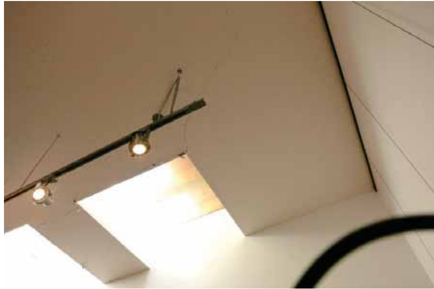
Figure 10-11 Cracking of gypsum wallboard ceiling.
