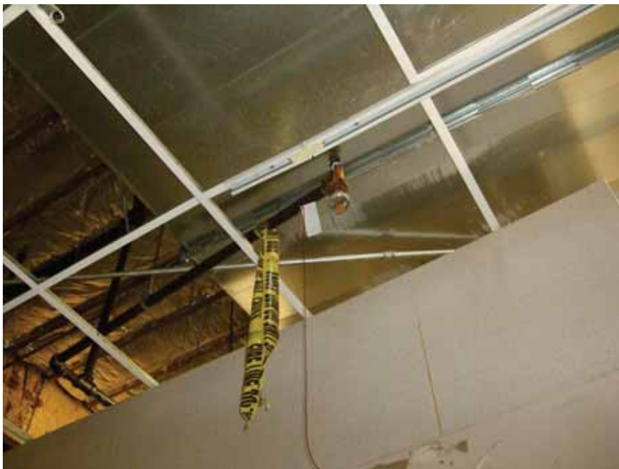
Figure 10-23 Sprinkler armover in close proximity to HVAC components.
