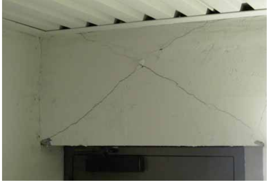
Figure 4-14 Cracking in spandrel in concrete stair core.
