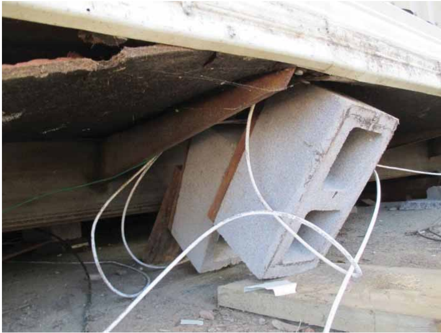
Figure 8-14 Close-up of toppled masonry gravity pier.
