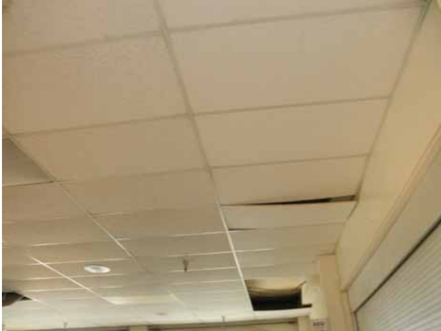
Figure 4-21 Minor damage to suspended ceilings.
