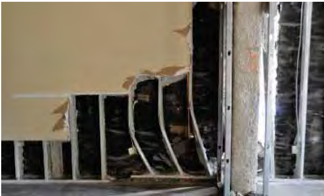
Figure 4-7 Damaged studs in exterior wall.
