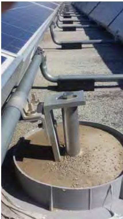
Figure 10-43 Mechanical attachment of solar array on the roof of an office/warehouse building two miles east of earthquake epicenter (photo from PanelClaw, Inc.). Array includes ballast and mechanical attachments to the building roof at selected locations. Mechanical attachments are evenly distributed throughout the array and typically showed similar evidence of possible movement.
