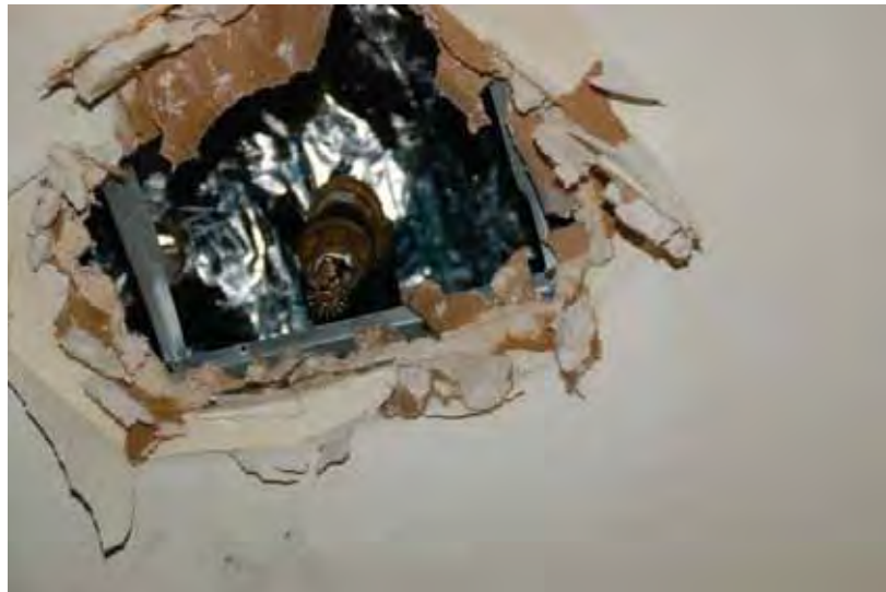
Figure 4-18 Sprinkler impacted HVAC components and discharged.
