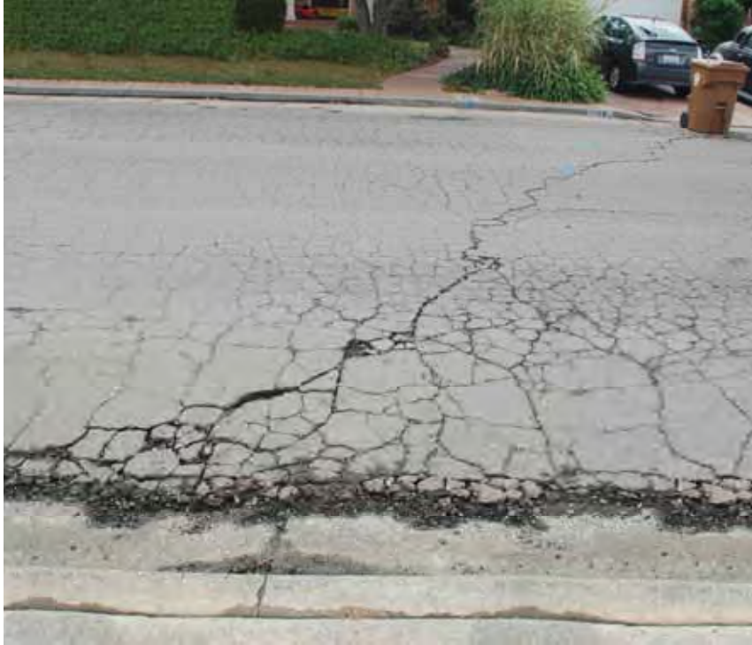
Figure 7-2 Surface feature of fault rupture observed on street.
