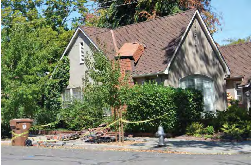
Figure 7-23 Photo of damaged chimney (photo from Janiele Maffei)
