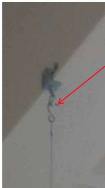
Figure 10-18 “S” hook opened during earthquake and caused fixtures to drop.
