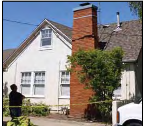
Figure 1: Chimney damaged in the South Napa Earthquake. Photo Credit: Exponent.
