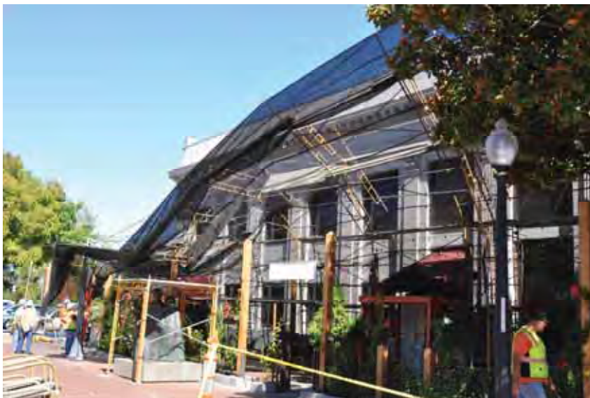
Figure 12-5 Scaffolding used as a barricade damaged in a windstorm (photo by Fred Turner).
