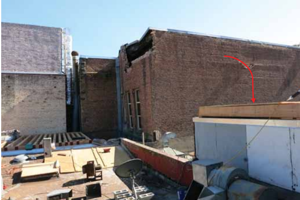
Figure 12-7 Protective barrier constructed over the rooftops of buildings to protect from falling brick.
