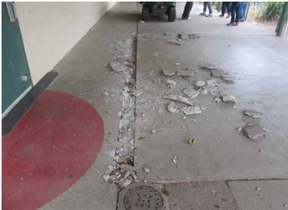
Figure 6-35 Cracking at slab joint in walkway at Harvest Middle School (photo by Quattrocchi Kwok Architects).
