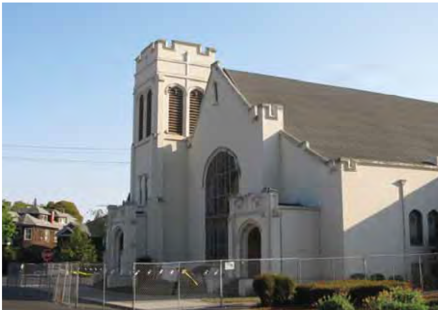
Figure 12-2 Church with damaged gable façade where the fence setback was less than a 1.5H:1V set back distance.
