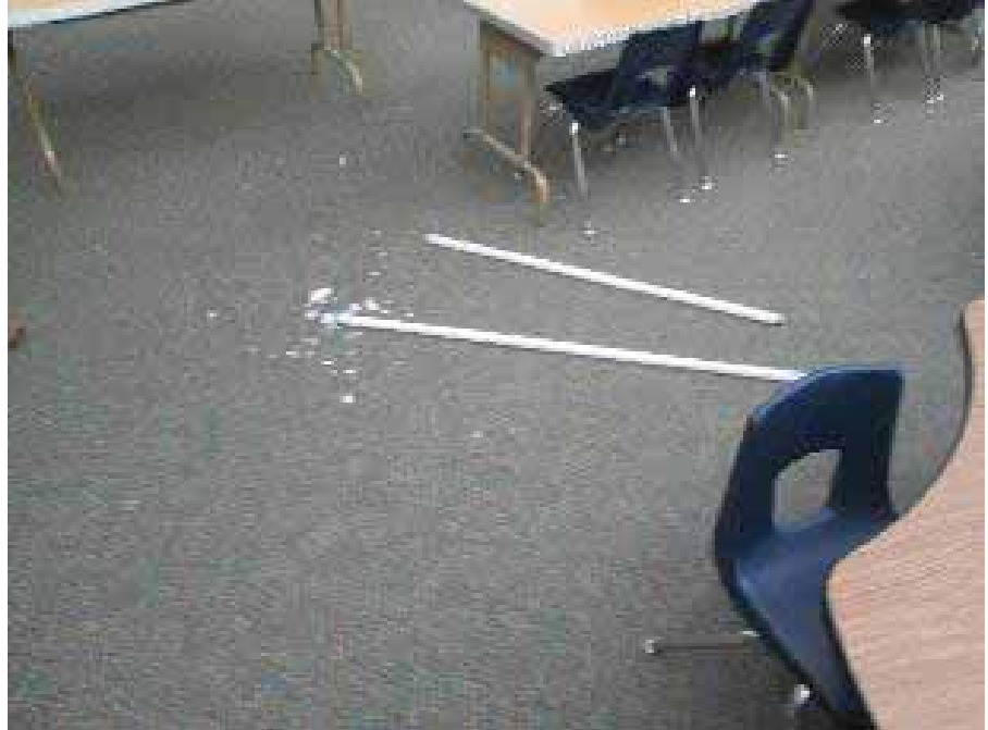
Figure 6-10 Dislodged fluorescent bulbs at Shearer Elementary School (photo by Quattrocchi Kwok Architects).
