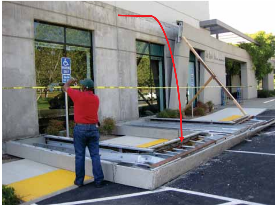
Figure 10-5 Metal stud and stucco framed cladding dislodged from concrete wall.
