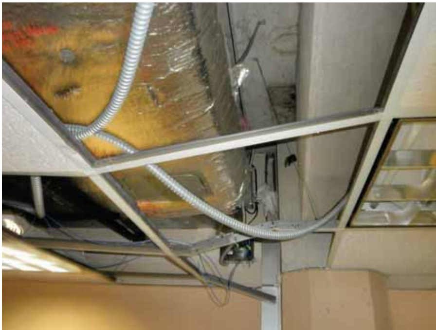
Figure 4-43 Ceiling damage at seismic joint.
