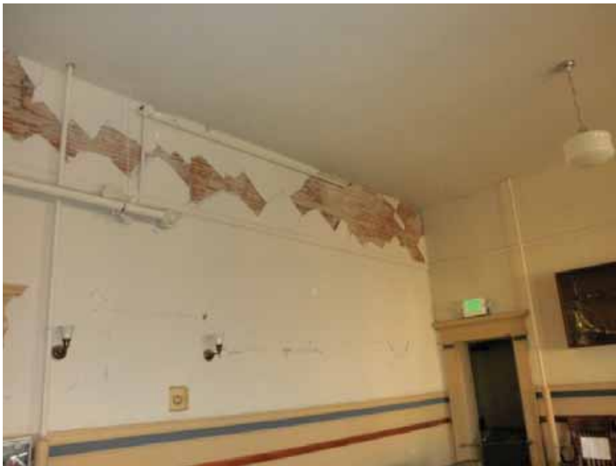
Figure 10-10 Cracked and spalled plaster on lath and plaster wall.
