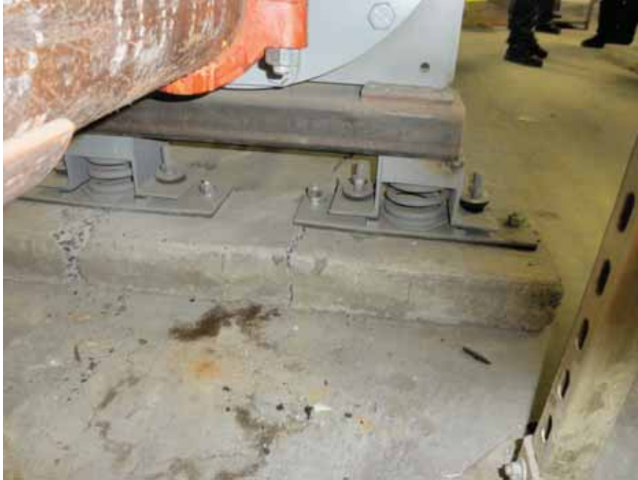
Figure 4-42 Housekeeping slab failure, chiller in 1974 wing penthouse.
