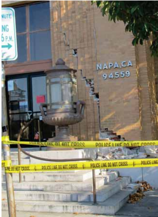
Figure 4-24 Damage to corner pier.
