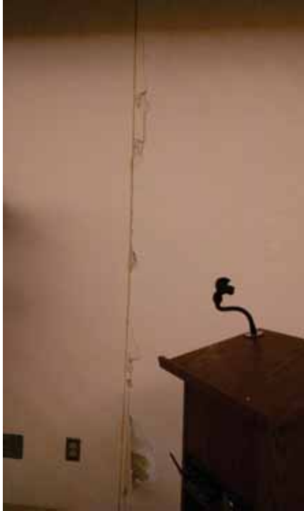
Figure 5-5 Cracked precast concrete panel in BLD-01653.
