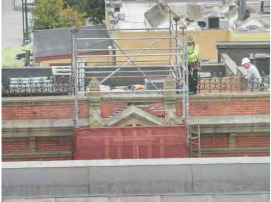
Figure 4-86 Damage to stonework above main entrance.
