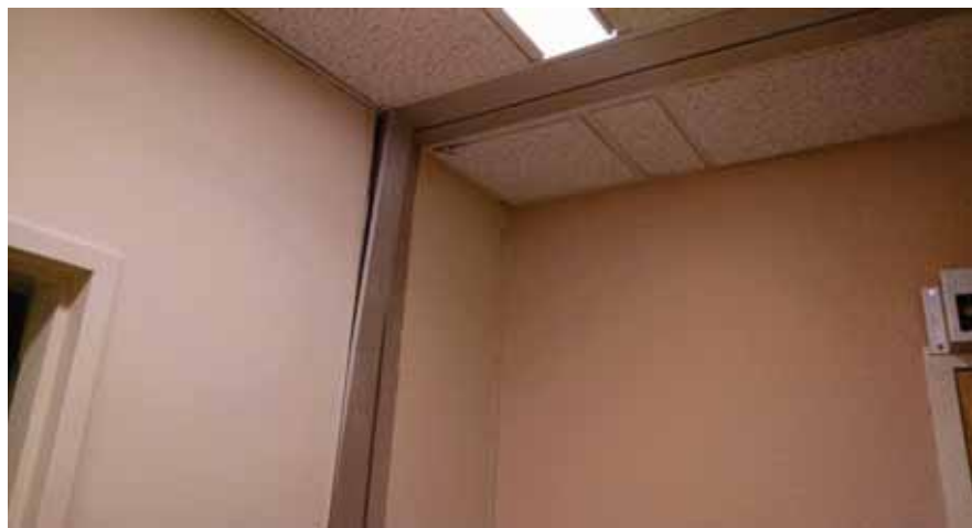
Figure 5-14 Damage to seismic joint cover at second floor of BLD-01659.
