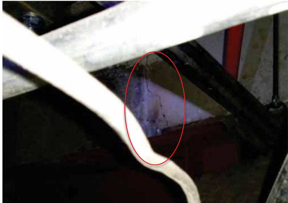
Figure 5-3 Damaged concrete beam at the third floor of BLD-01650.
