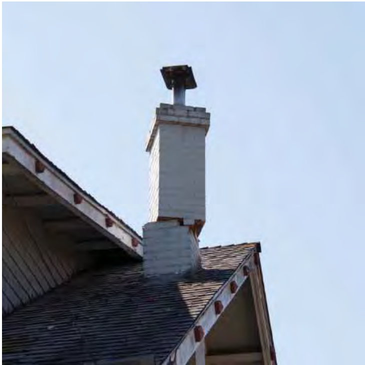
Figure 7-22 Dislodged unreinforced masonry chimney (photo from Janiele Maffei).
