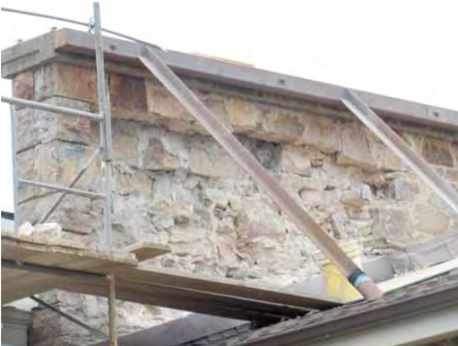
Figure 4-75 Close up of dislodged stone on inside face of parapet.
