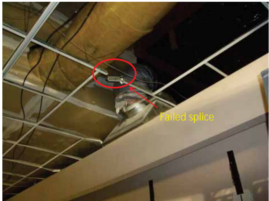
Figure 10-15 Failure of a splice of acoustical tile ceiling grid in a two-story retail store in downtown Napa.
