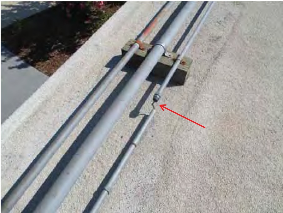
Figure 6-33 Broken low voltage conduit coupling at Redwood Middle School (photo by Quattrocchi Kwok Architects).
