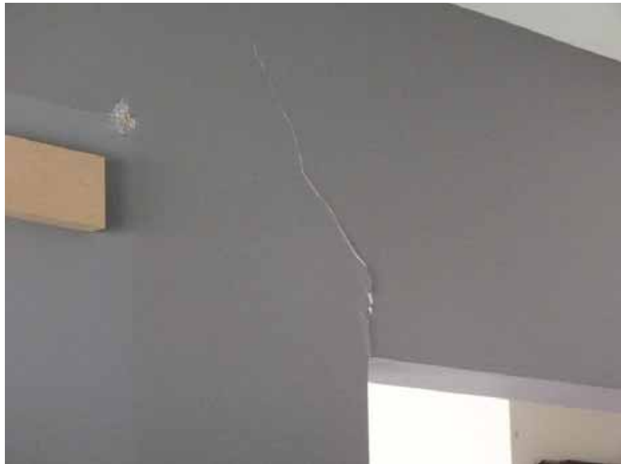
Figure 10-8 Typical damage to gypsum wallboard.
