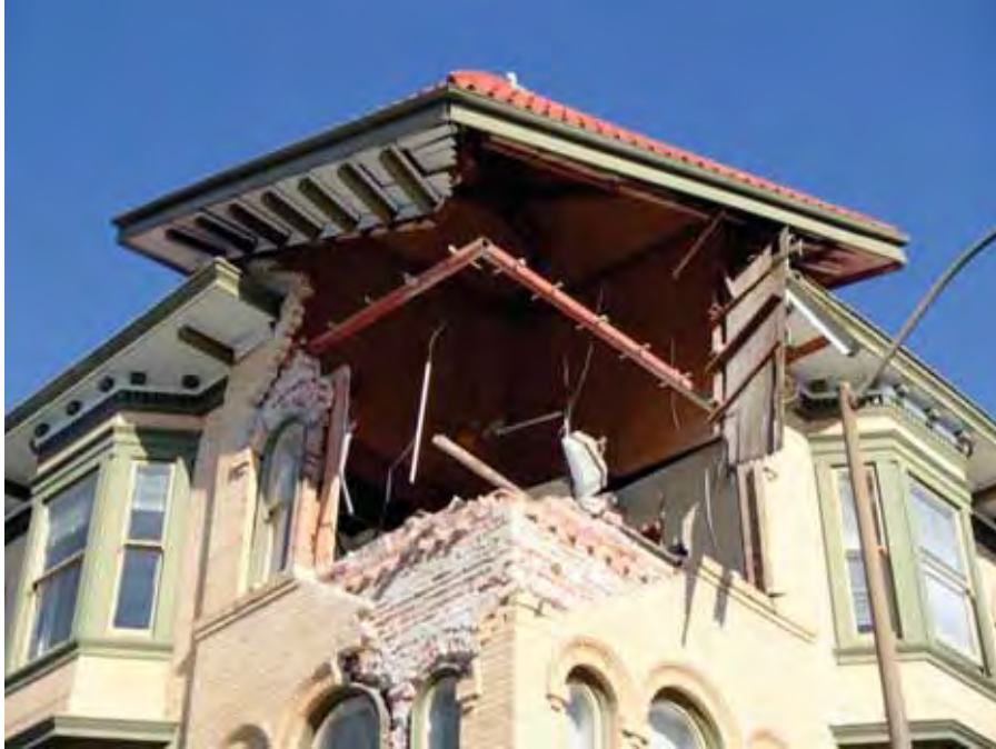
Figure 4-56 Collapse of URM walls supporting a corner cupola.
