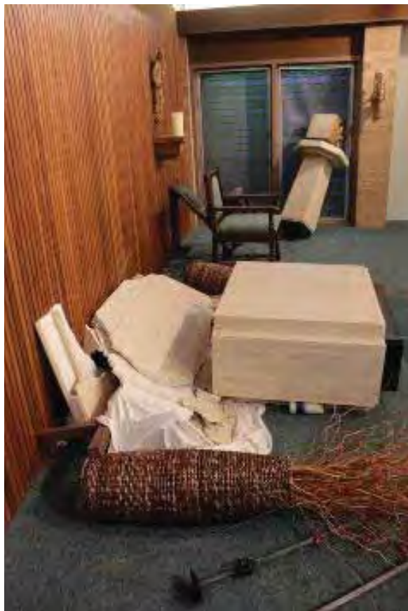
Figure 6-39 Toppled altar and statuary (photo by Quattrocchi Kwok Architects).
