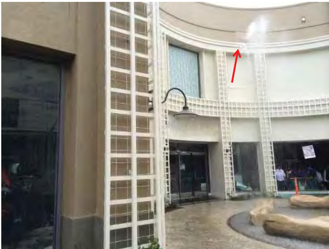
Figure 4-45 Water pressure from broken sprinkler line created a hole in the exterior cladding (photo by KCRA.com).
