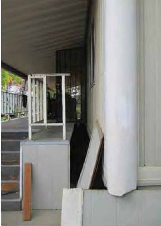
Figure 8-21 Gap between front porch and home on home with ERBS that slid a significant distance.
