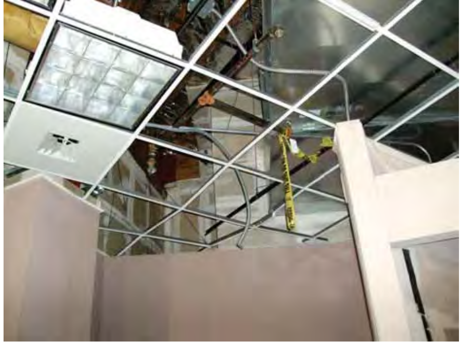
Figure 4-46 Damaged sprinkler pipe. Damage believed to have been caused by interaction with adjacent air handler.
