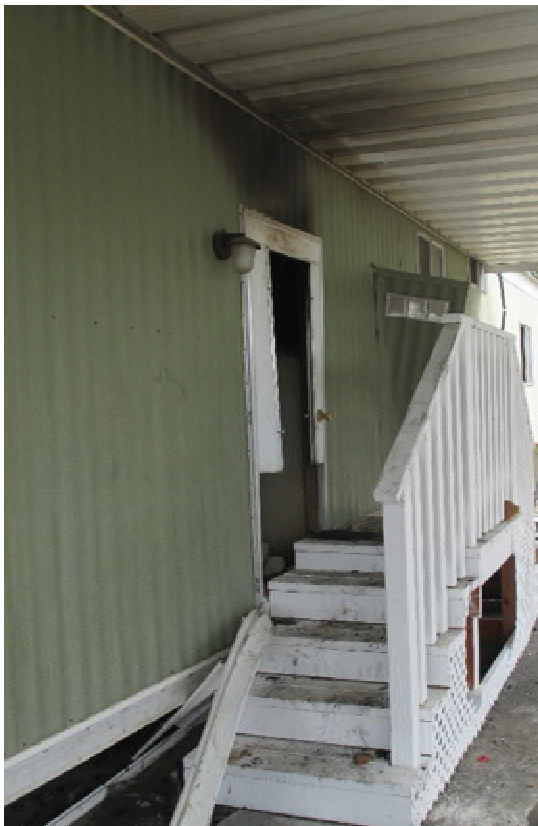
Figure 8-15 This door was blocked when the home dropped off of the gravity supports and had to be broken open by fire fighters.
