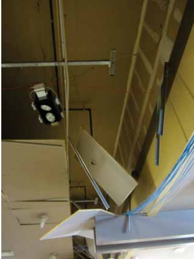
Figure 4-30 Suspended ceiling damage.
