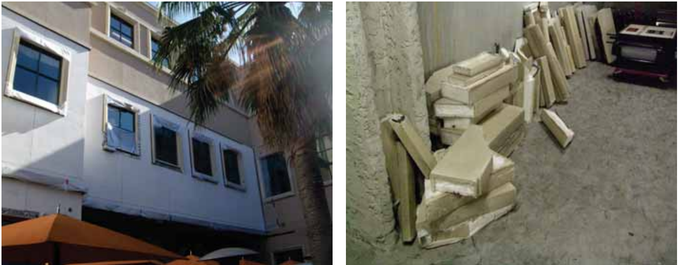
Figure 4-12 Dislodged adhered veneer.
