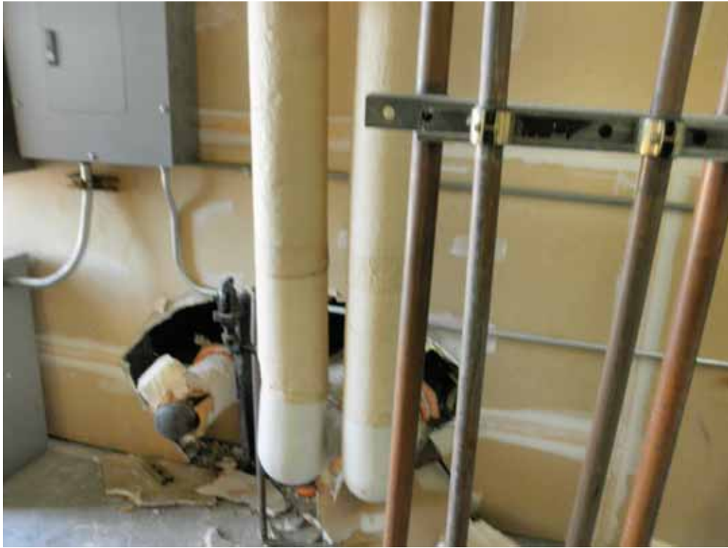
Figure 4-32 Evidence of pipe motion in penthouse partition wall.
