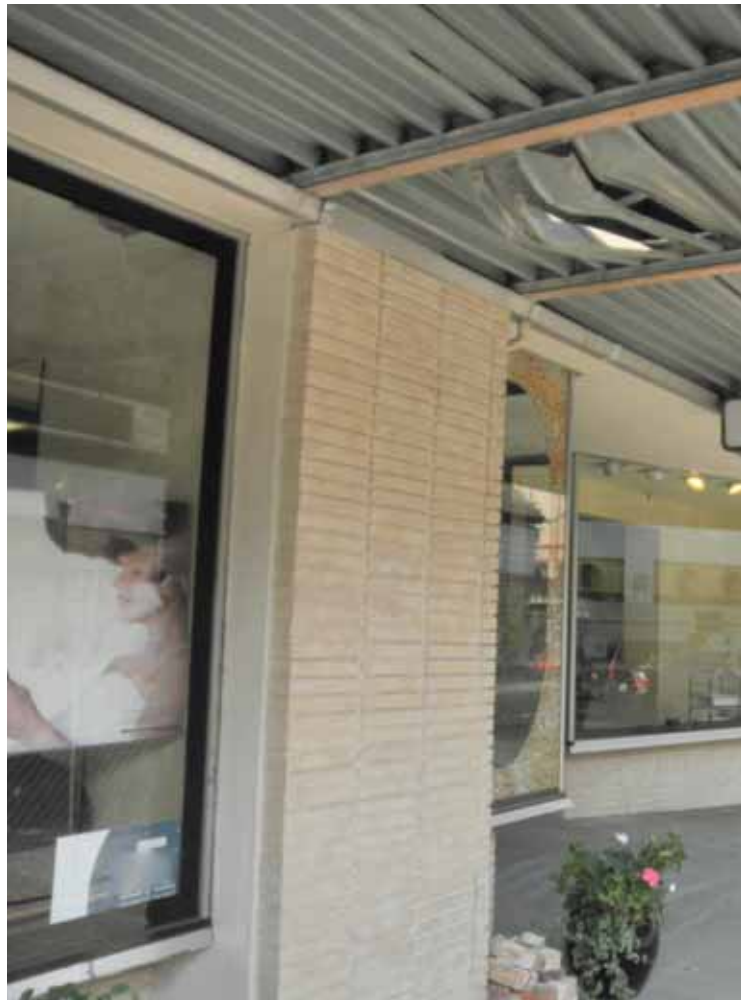
Figure 4-20 Damage to canopy due to falling brick.
