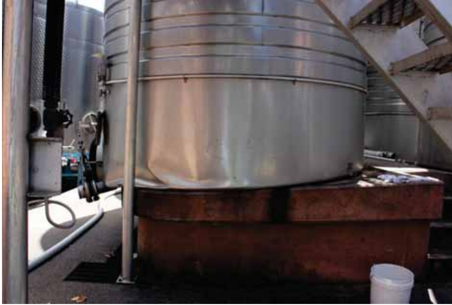
Figure 9-2 Anchorage failure allowed tank to shift on pedestal.
