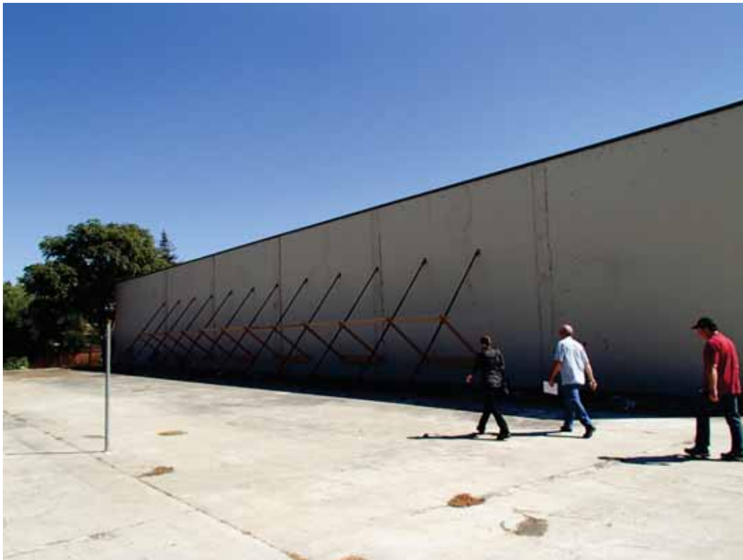
Figure 4-27 Shoring of wall with damaged pilasters.
