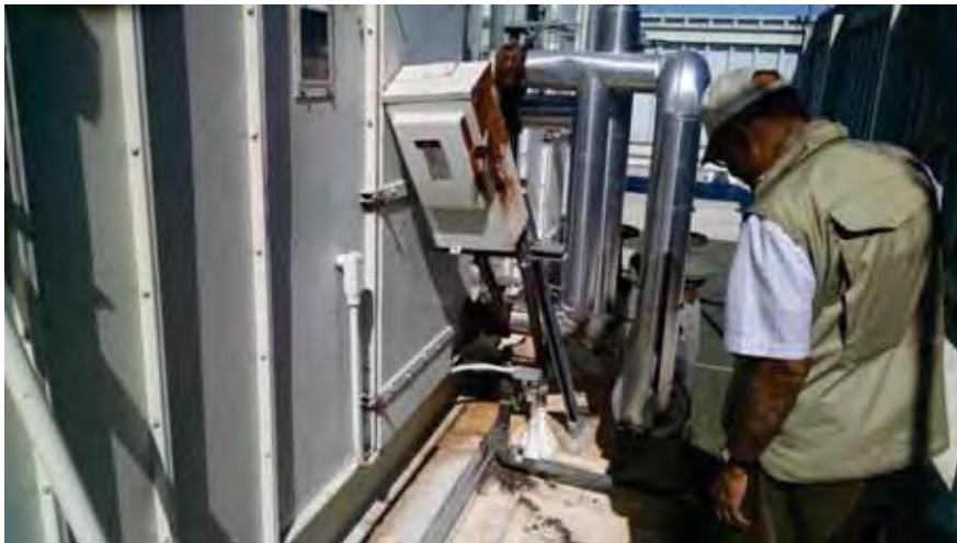
Figure 5-16 Electrical panel on cantilevered supports damaged at roof of BLD-01656.
