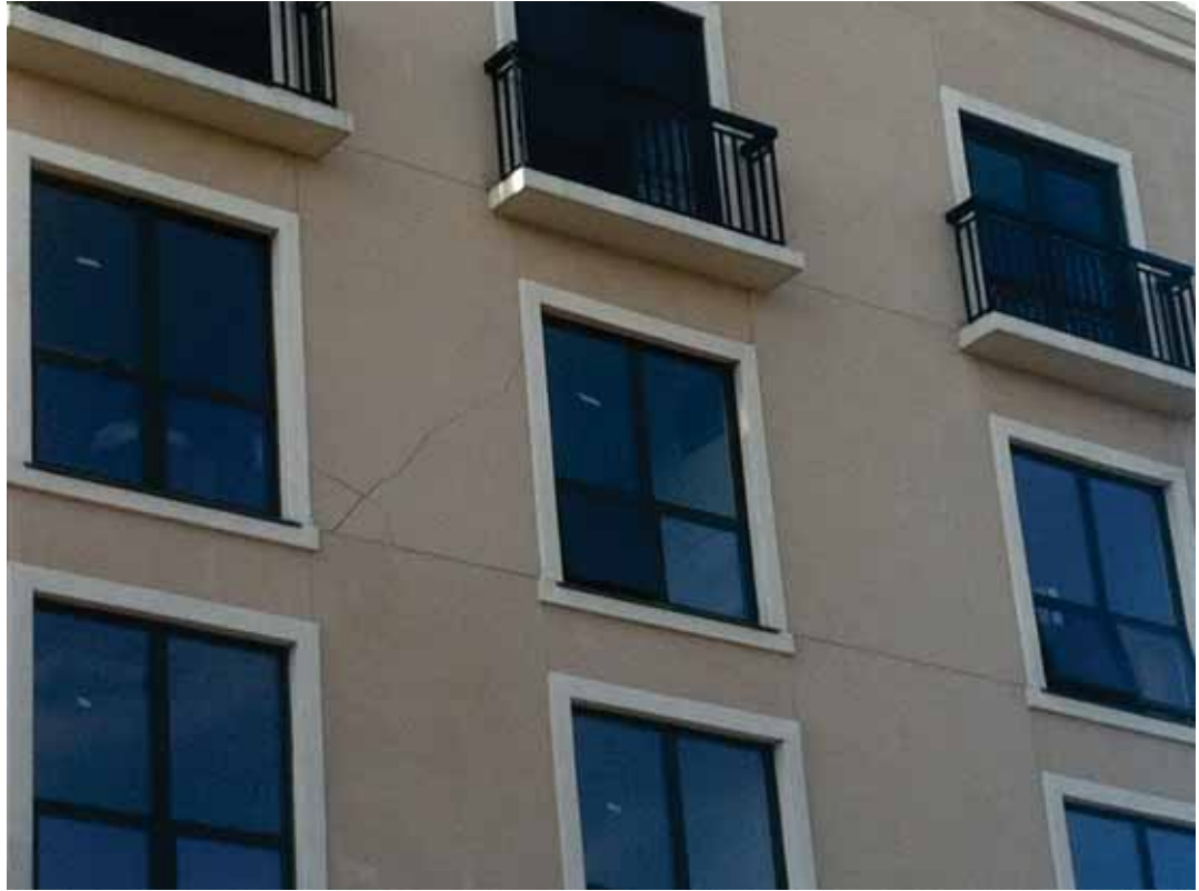
Figure 4-11 Exterior wall, cracked plaster.
