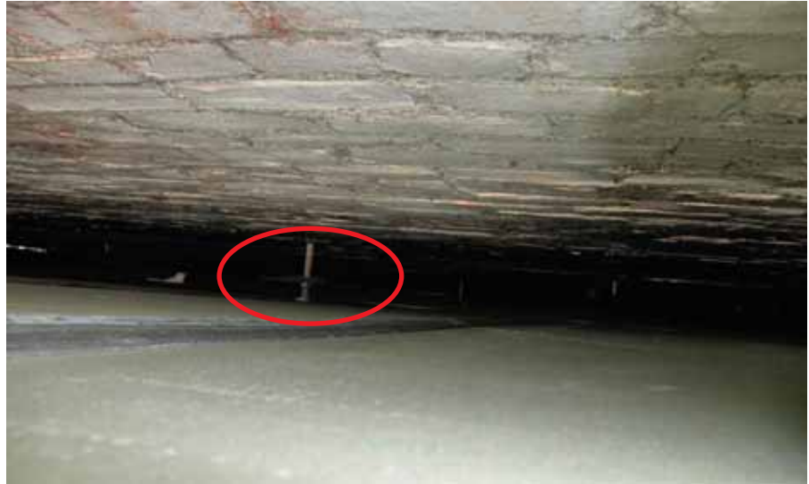
Figure 4-70 Loosened wall anchors on south wall, looking down.
