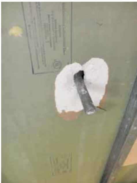
Figure 4-5 Out-of-plane wall anchor of adjacent building penetrated drywall.
