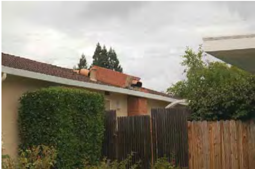
Figure 7-5 Brick chimney collapse on to the roof.
