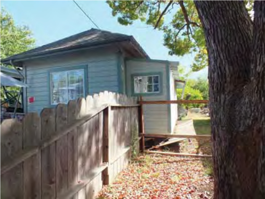
Figure 7-13 Building fell into adjoining property.
