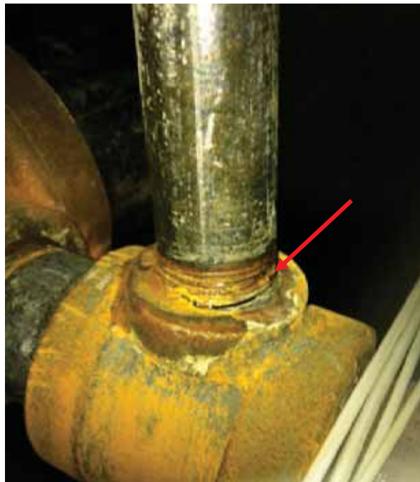
Figure 4-29 Cracked sprinkler pipe.
