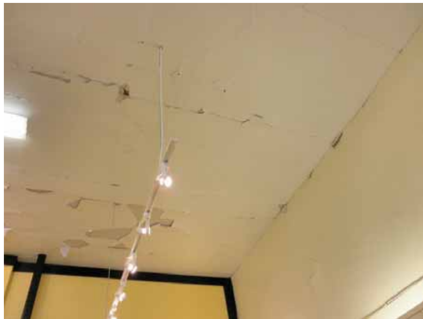
Figure 10-12 Cracking and spalling of a plaster ceiling in an older masonry building in downtown Napa.
