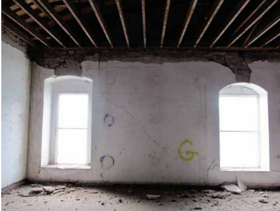
Figure 4-79 Diagonal cracking at inside face of second story pier at front façade.
