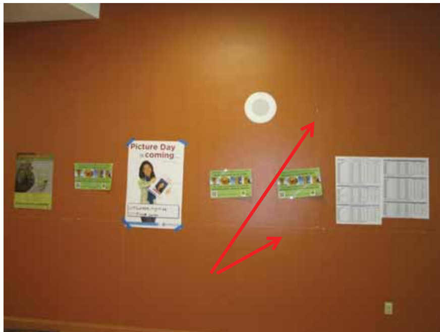
Figure 6-20 Gypsum wallboard cracking in New Technology High School (photo by Quattrocchi Kwok Architects).
