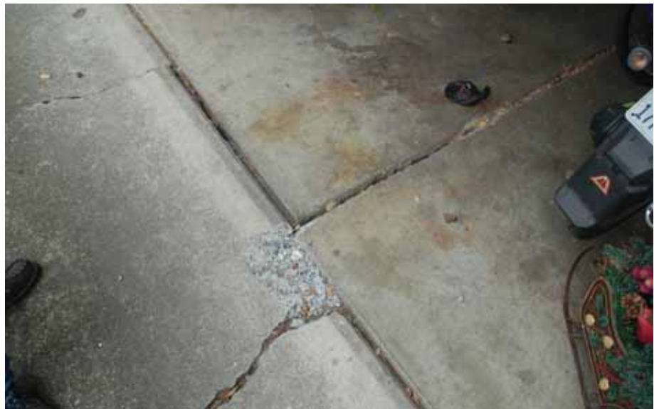
Figure 7-8 Damage caused due to differential movement of floor slabs in garage and driveway pavement.
