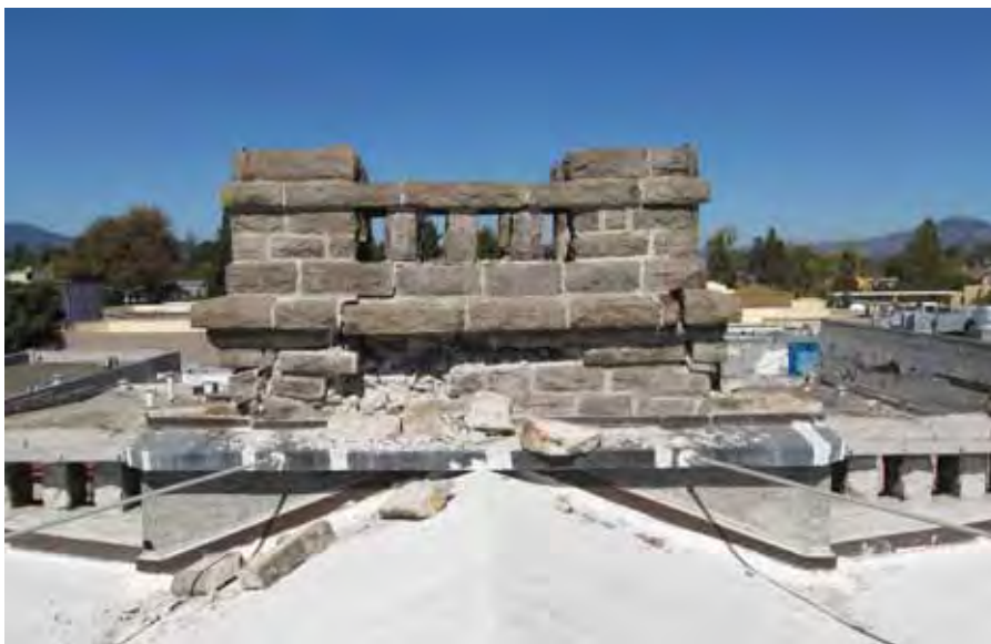
Figure 4-61 Top of concrete shear wall at roof level behind the tower feature.
