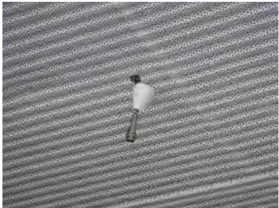
Figure 6-3 Aircraft cable slipped out of the cable gripping support fixture at Pueblo Vista Elementary School (photo by Quattrocchi Kwok Architects).
