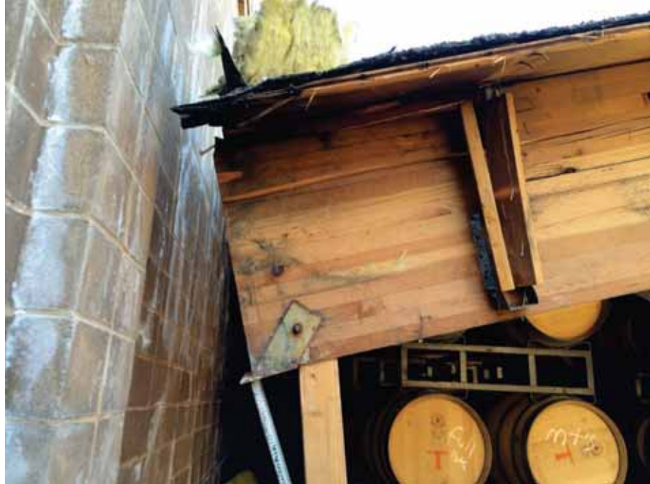
Figure 9-5 Failure of glulam beam to wall connection resulted in roof collapse.
