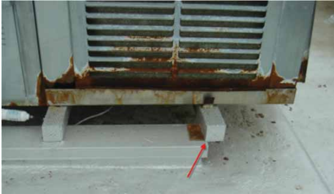
Figure 6-26 Shifted rooftop make-up air unit at Napa High School (photo by Quattrocchi Kwok Architects).
