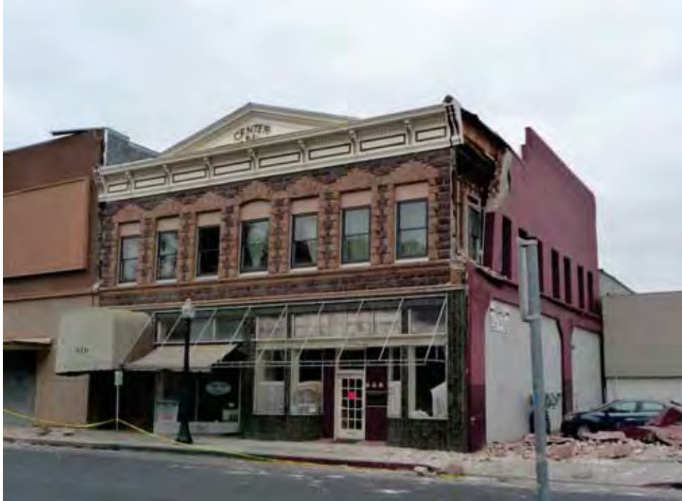
Figure 4-49 Failure of URM south wall (photo courtesy of Marko Schotanus).
