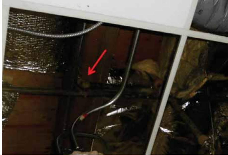
Figure 10-20 Sprinkler head interaction with adjacent components resulted in extensive flooding.
