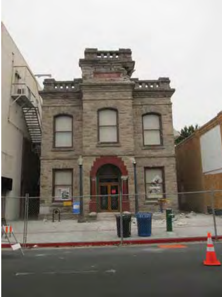
Figure 4-59 Front façade showing damage and UNSAFE placard before scaffolding was installed.
