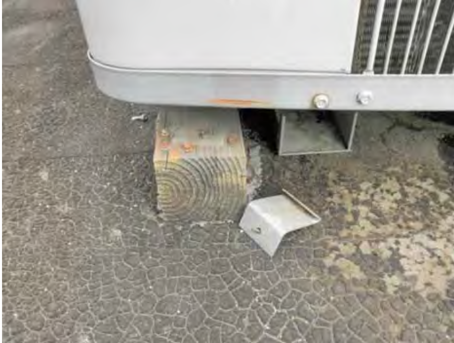
Figure 4-88 Failure of air handler unit anchor, screws pulled out of sleeper.
