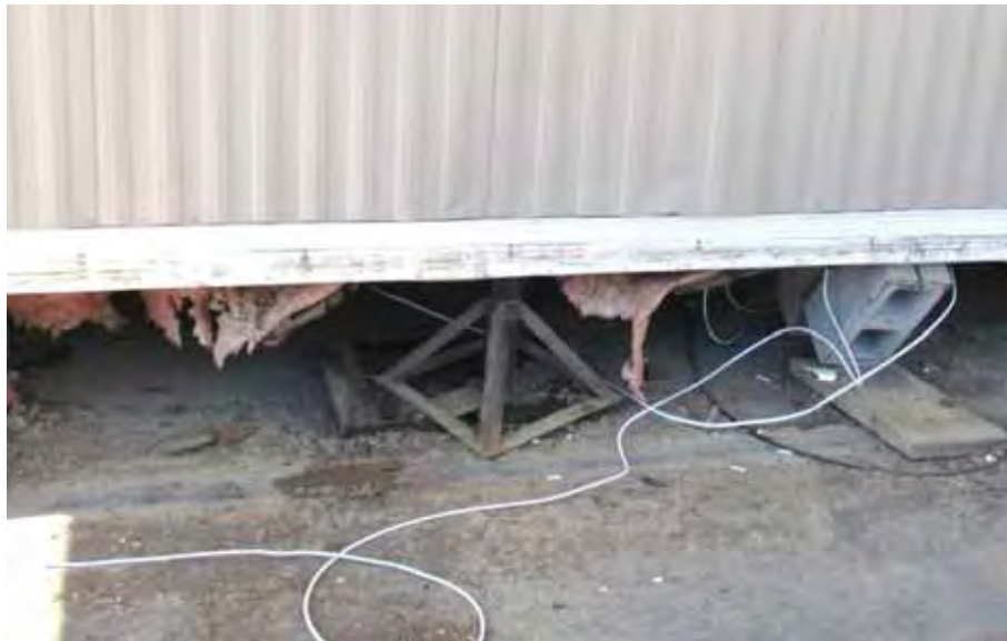
Figure 8-20 “Cantilevered” pier system that slid, adjacent to a masonry pier that has rolled over.
