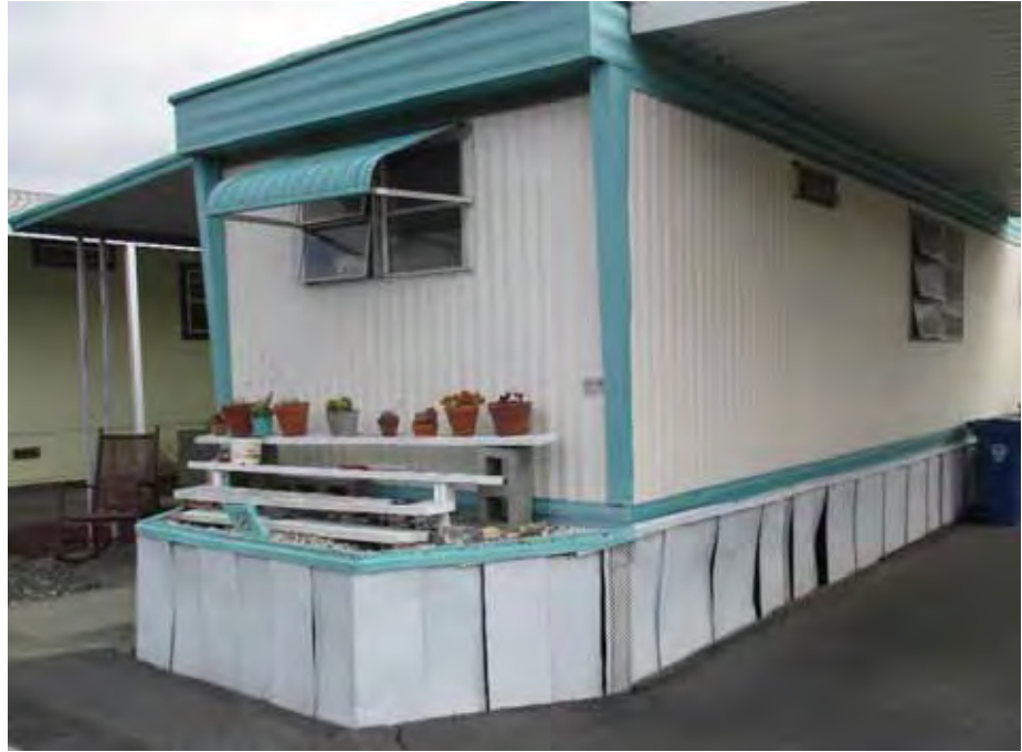
Figure 8-12 Damaged skirt on older home.
