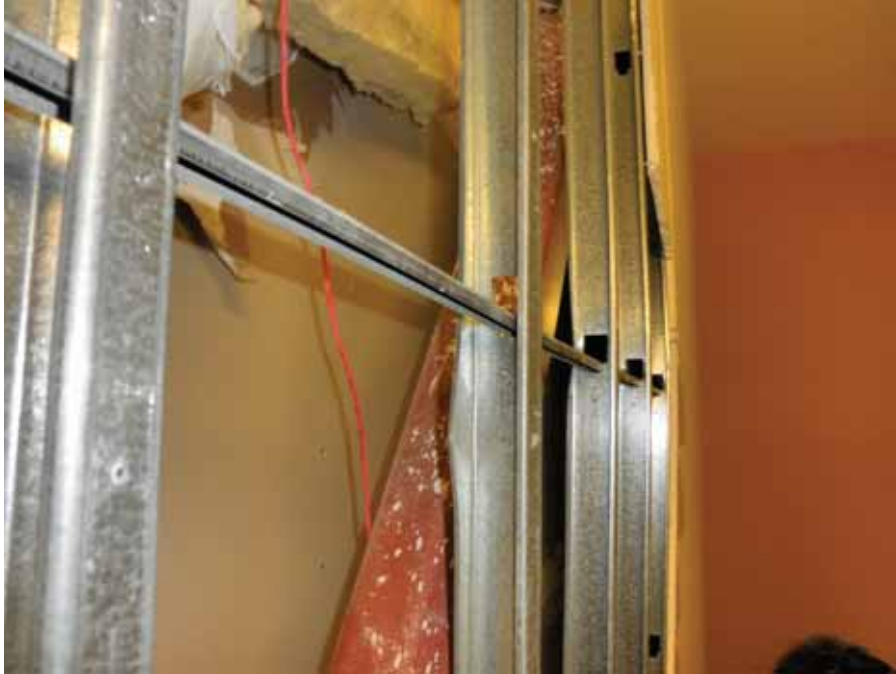
Figure 4-4 Damage to steel studs due to out-of-plane buckling of brace.
