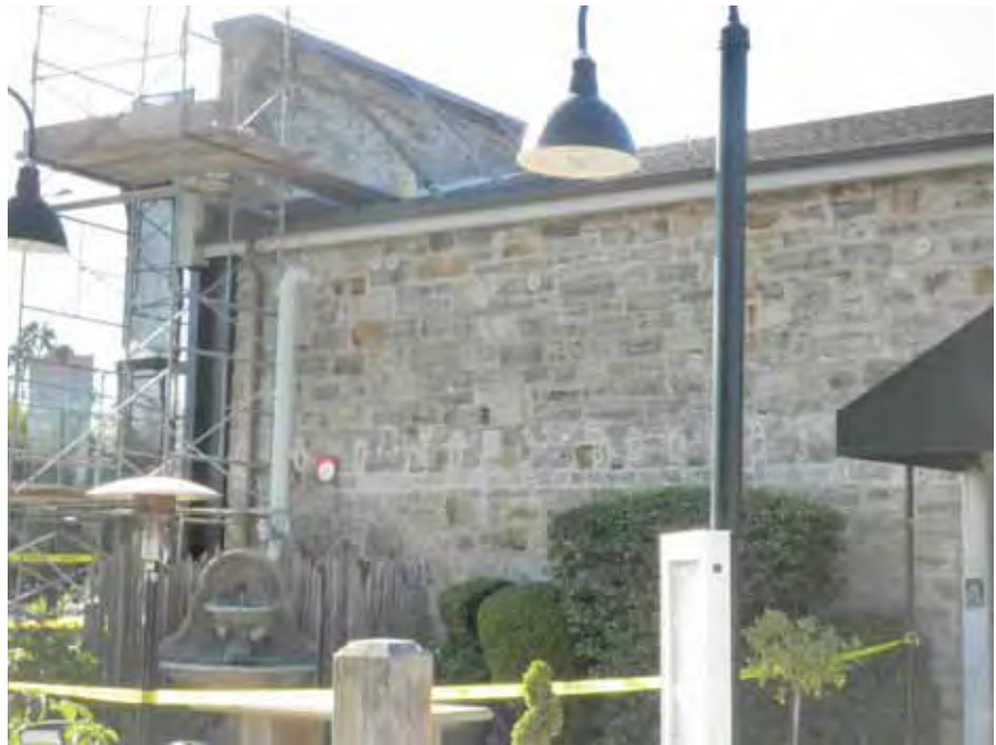
Figure 4-76 URM parapet bracing, loss of stonework.
