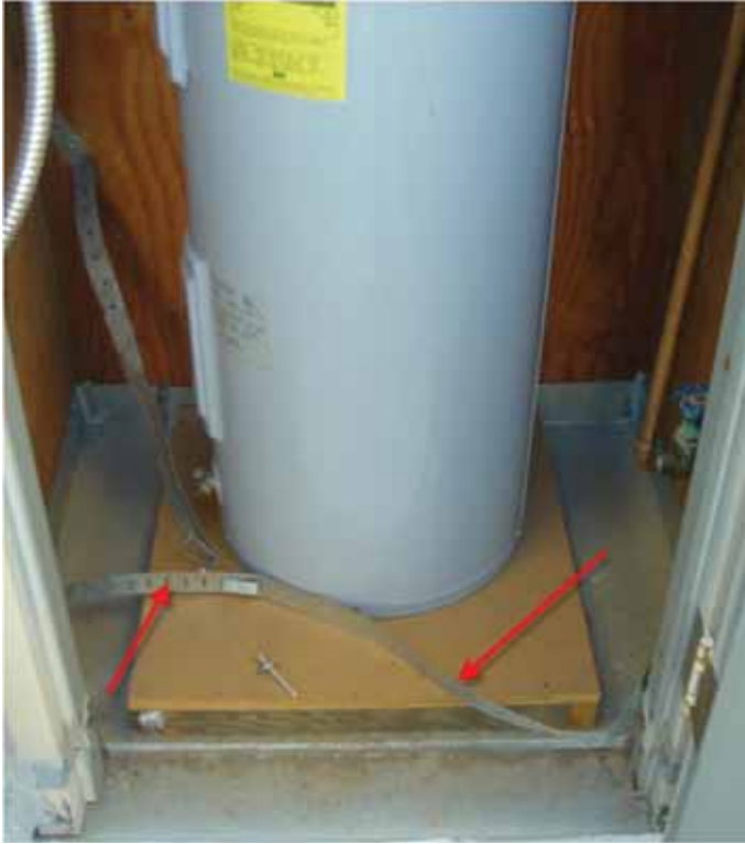
Figure 6-24 Failed earthquake restraining strap at Shearer Elementary School (photo by Quattrocchi Kwok Architects).
