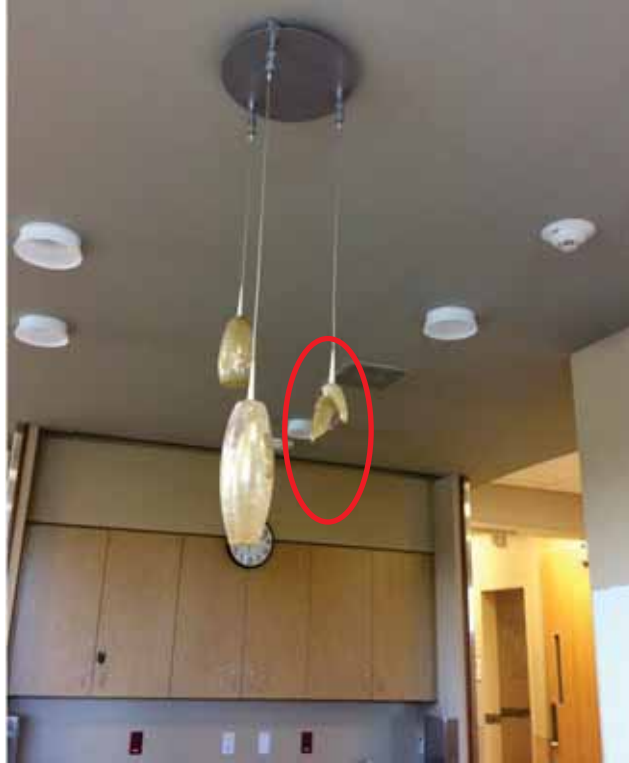
Figure 5-17 Damaged light fixture in BLD-05309.
