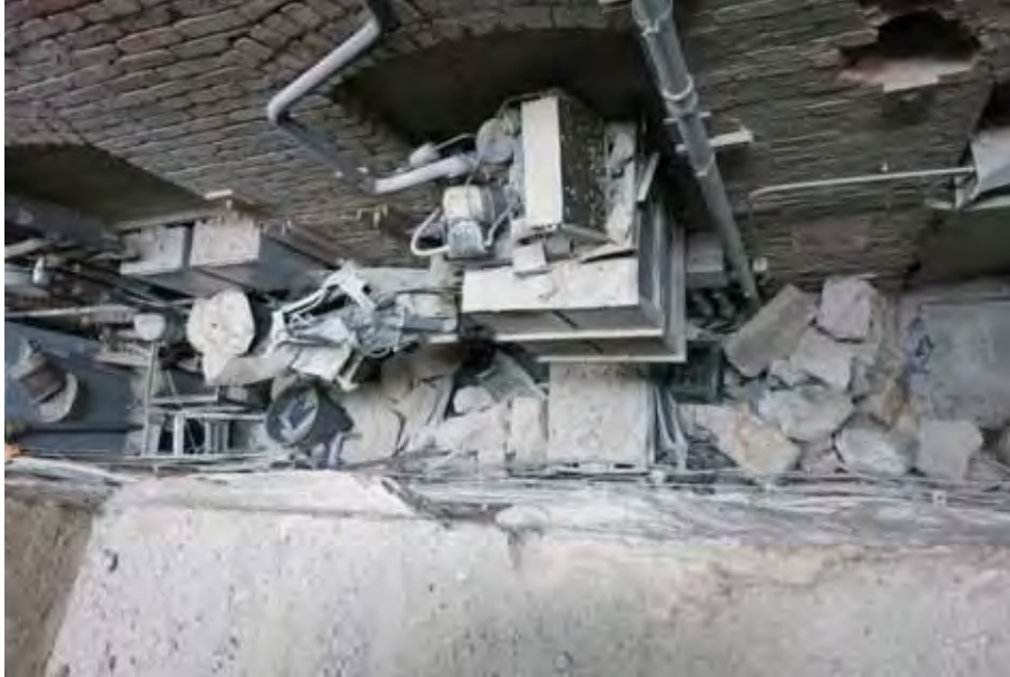
Figure 4-52 HVAC equipment damaged by falling stones.
