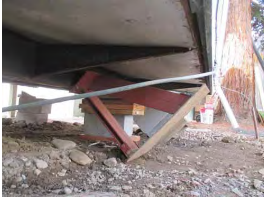
Figure 8-10 “Cantilevered” steel pier on home requiring reinstallation.
