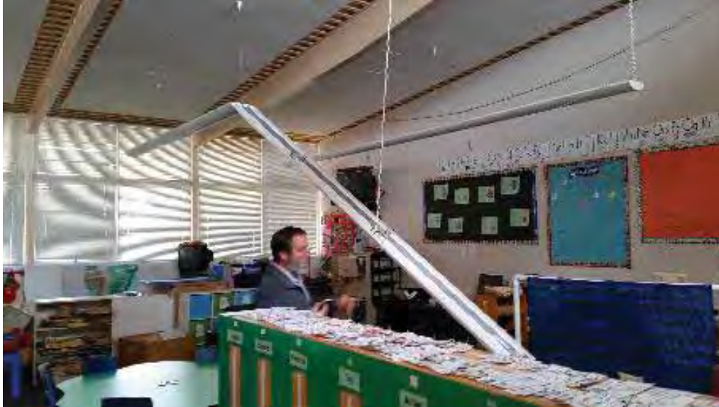
Figure 6-4 Damaged light fixtures in Irene M. Snow Elementary School (photo by Quattrocchi Kwok Architects).
