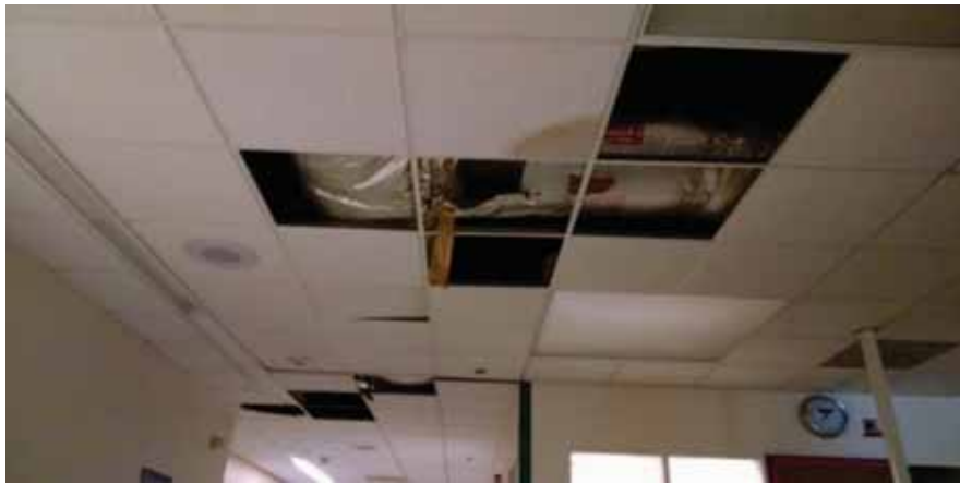
Figure 5-8 Third floor ceiling damage in BLD-01656.
