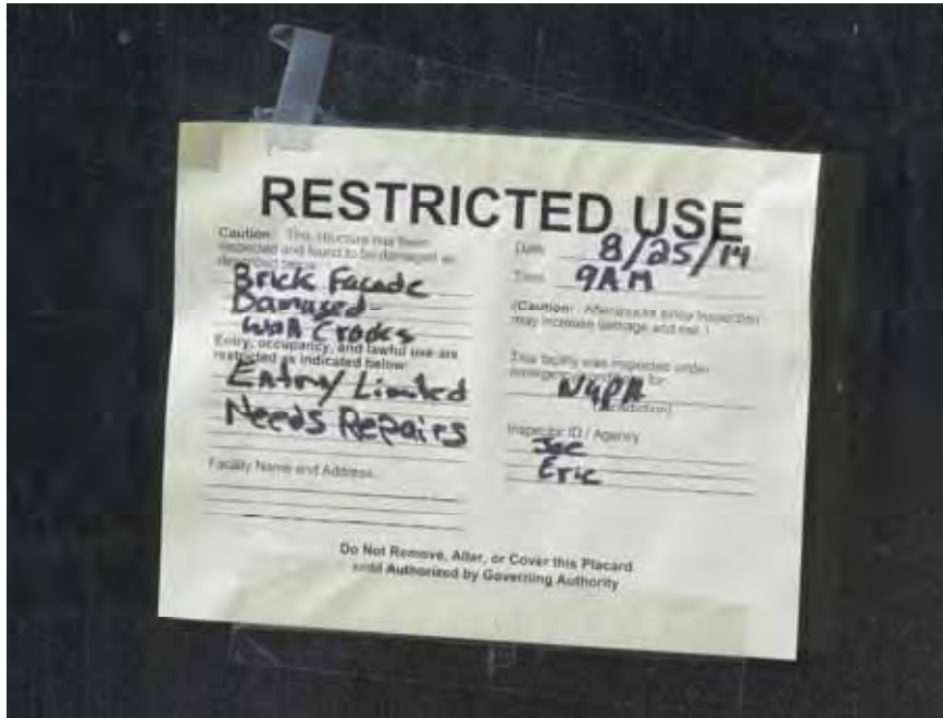
Figure 11-3 A RESTRICTED USE placard with no information on the restrictions.
