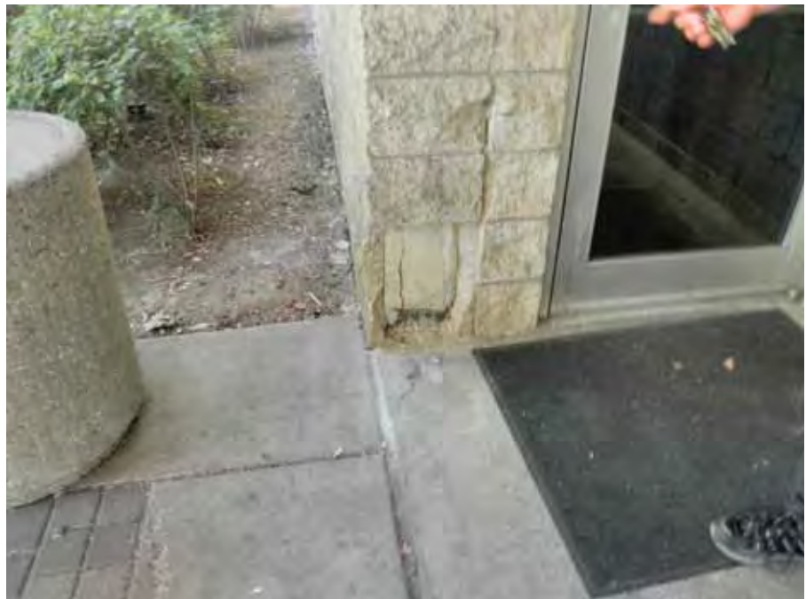
Figure 4-38 CMU face shell spalling, typical at base of walls.
