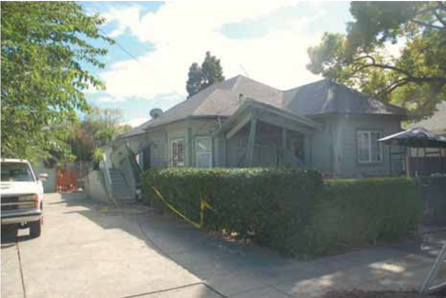
Figure 7-12 Home with collapsed cripple wall.
