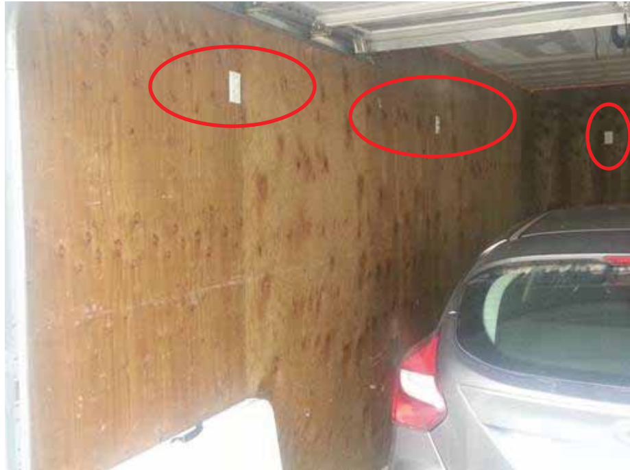
Figure 7-21 Braced wood cripple walls on the first story of elevated duplex homes. The height of the electrical outlets indicated the Base Flood Elevation.
