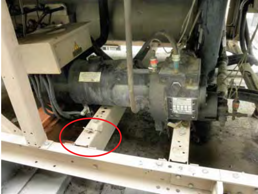
Figure 4-71 Connection failure at compressor.
