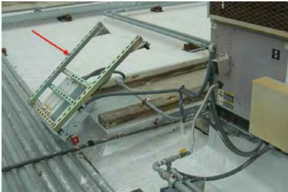
Figure 6-28 Toppled disconnect for rooftop air handler at Napa High School (photo by Quattrocchi Kwok Architects).
