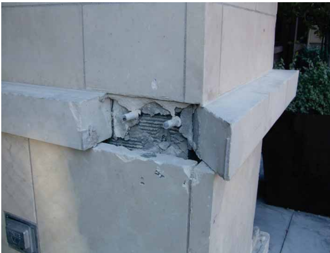
Figure 4-16 Photo showing failed anchored veneer.
