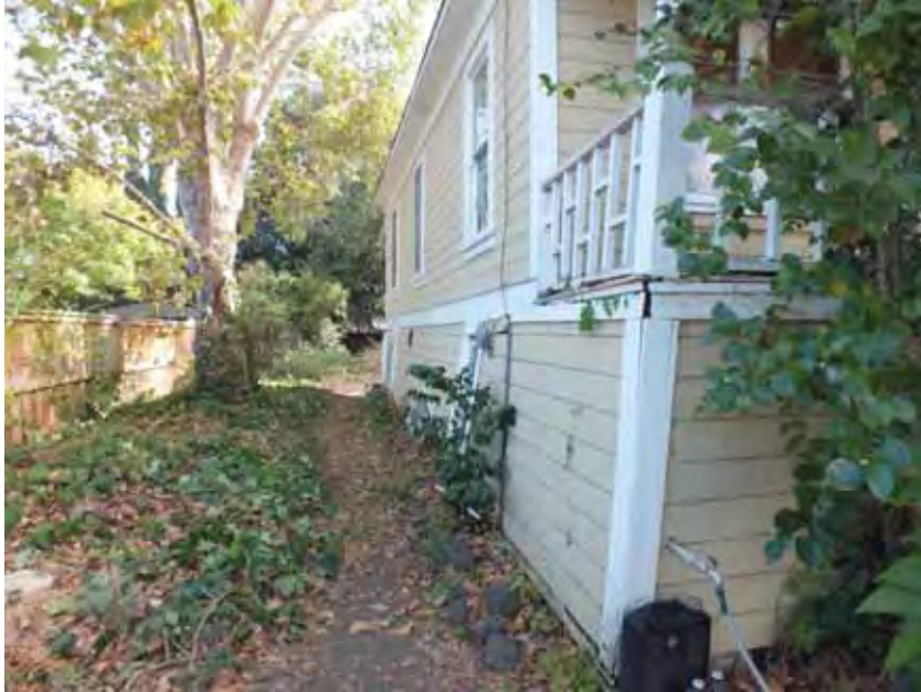
Figure 7-16 House shifted lateral at damaged cripple wall.
