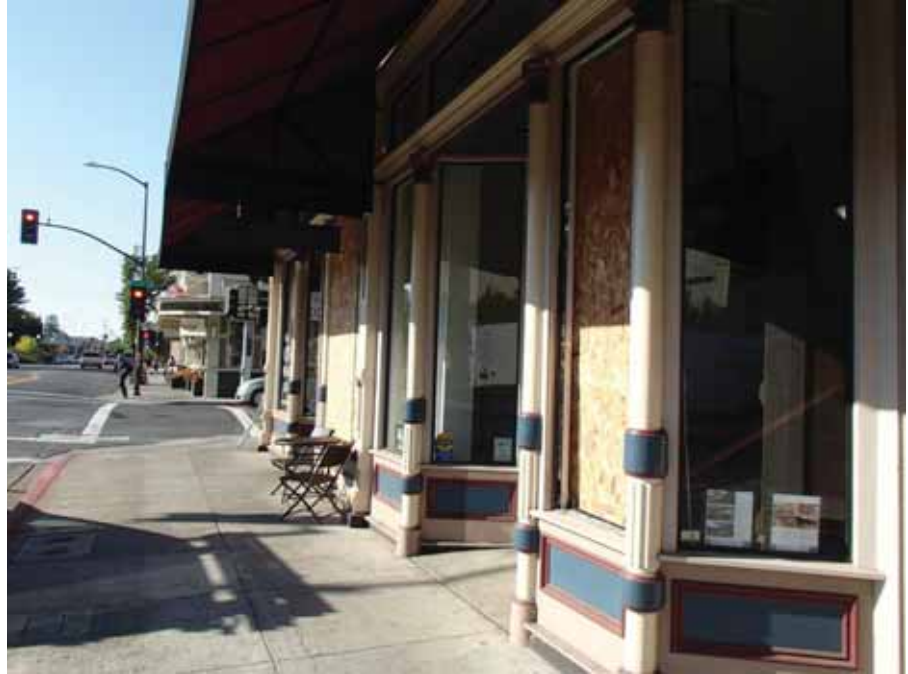
Figure 4-84 Damage to glazing, west elevation.
