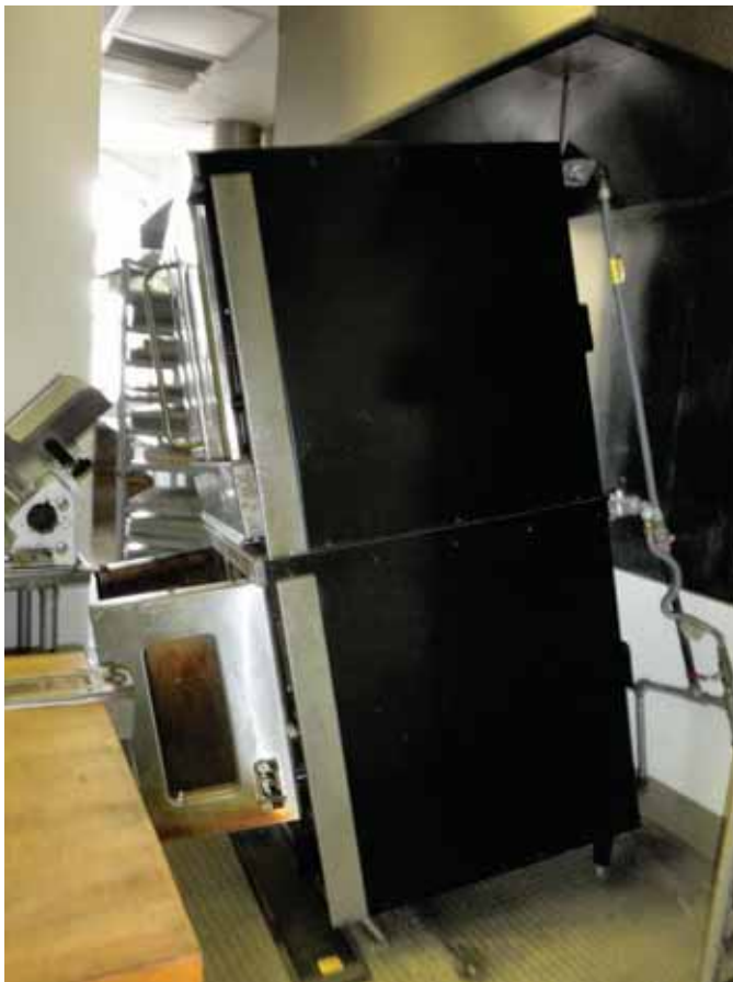
Figure 4-22 Convection oven with failed support leg.
