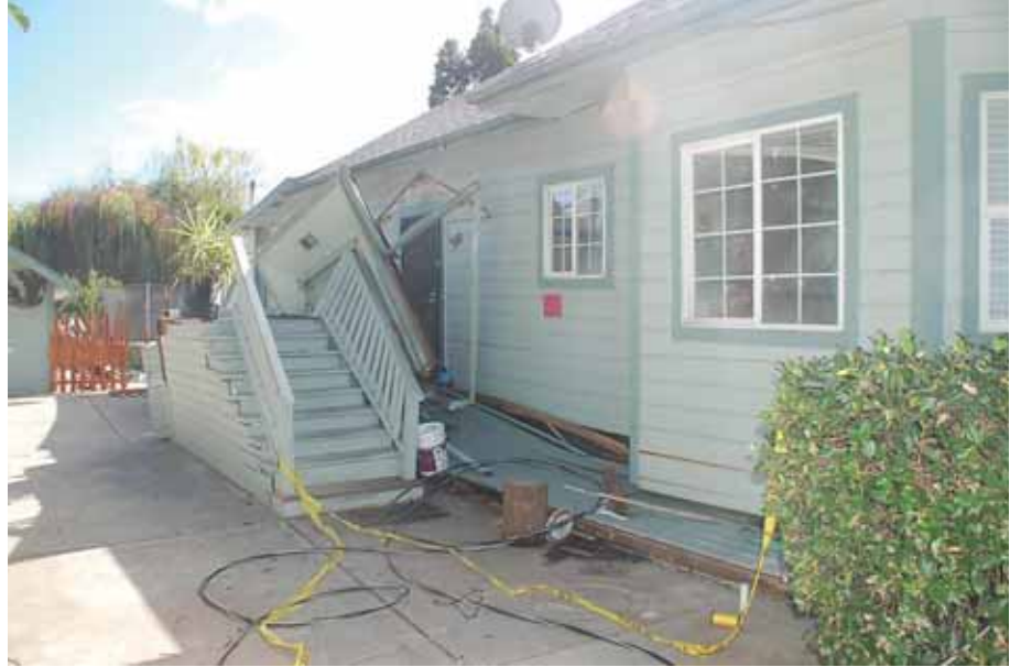
Figure 7-14 Failure of porch due to cripple wall collapse .
