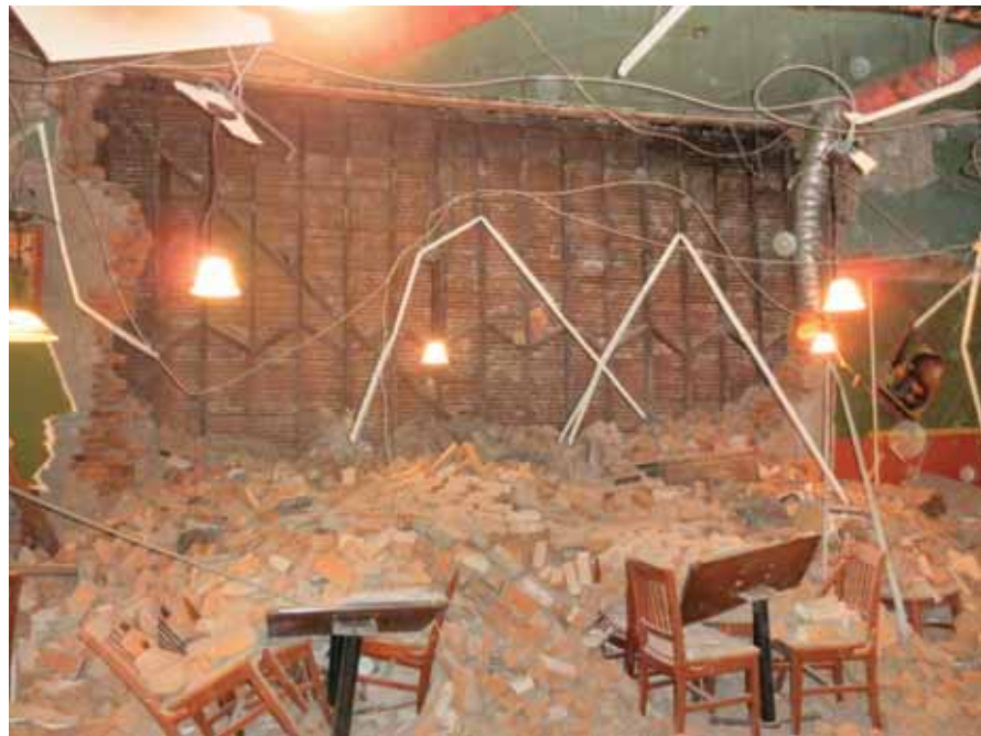
Figure 4-54 Collapsed URM wall and ceiling in dining area.
