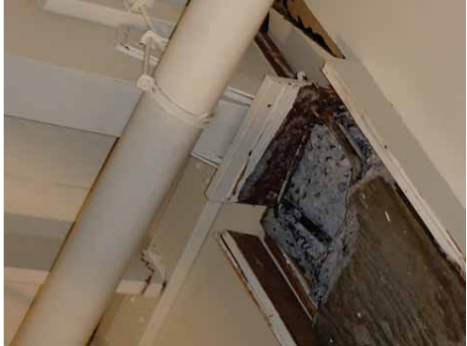
Figure 4-28 Damaged pilaster-to-roof beam connection.
