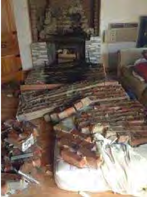
Figure 7-25 Photo of interior chimney collapse (photo from Janiele Maffei).
