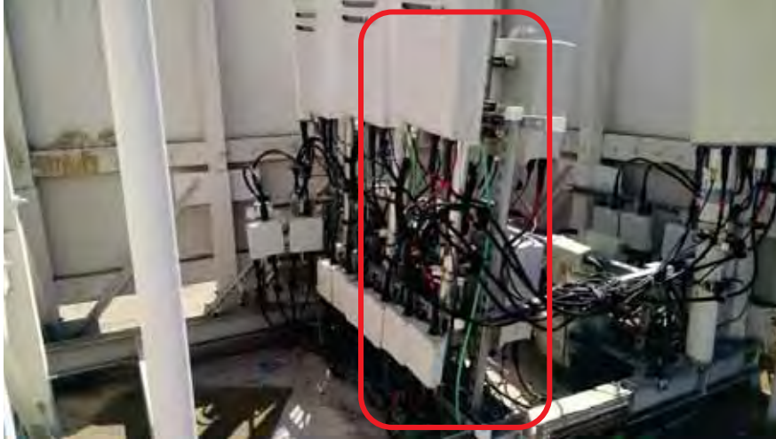
Figure 5-15 Telephone rack on cantilevered supporting frame at roof of BLD-01650 severely out of plumb.
