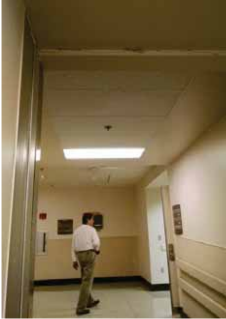
Figure 5-28 Evidence of movement along the separation joint at the fourth floor between BLD-01668 and BLD-01666.
