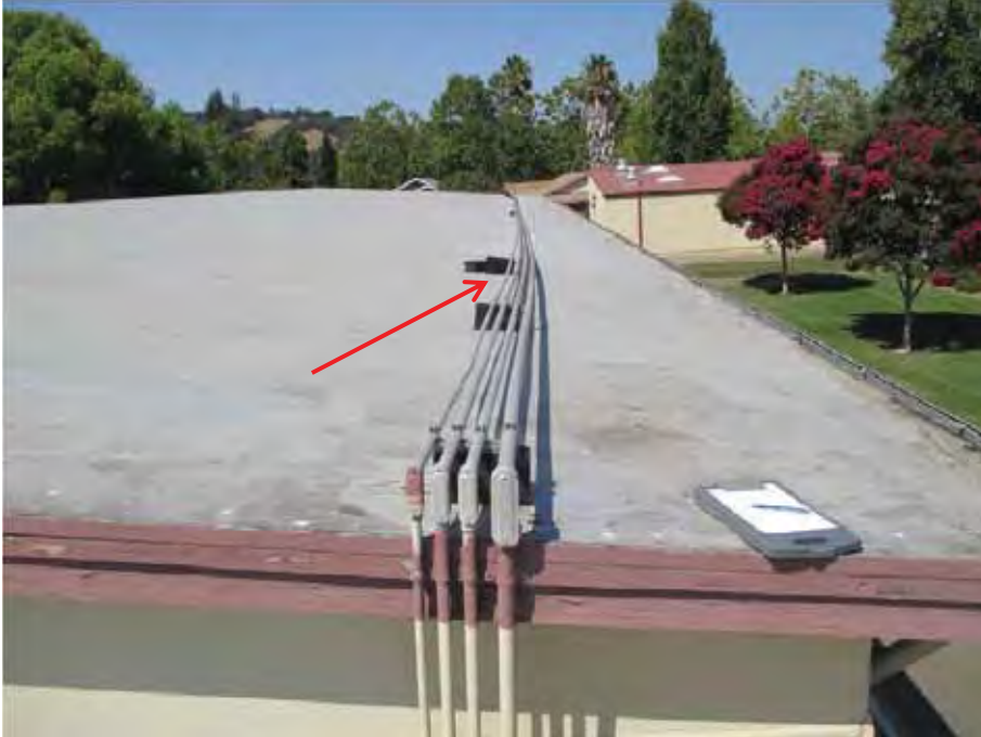
Figure 6-32 Shifted conduit at Napa Valley Language Academy (photo by Quattrocchi Kwok Architects).
