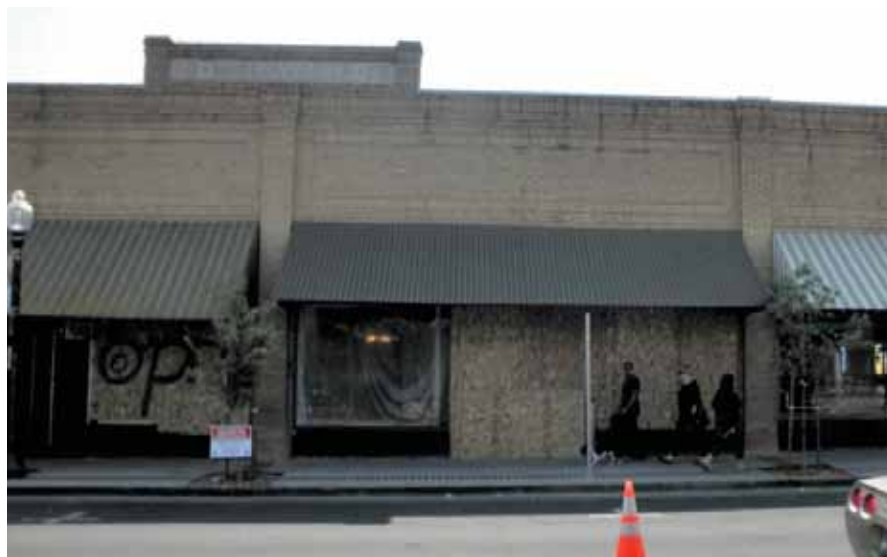
Figure 10-2 Typical condition showing temporary plywood barricades and plastic over openings where storefront glazing was damaged.
