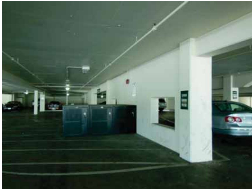
Figure 10-24 Sprinkler installation in parking garage.
