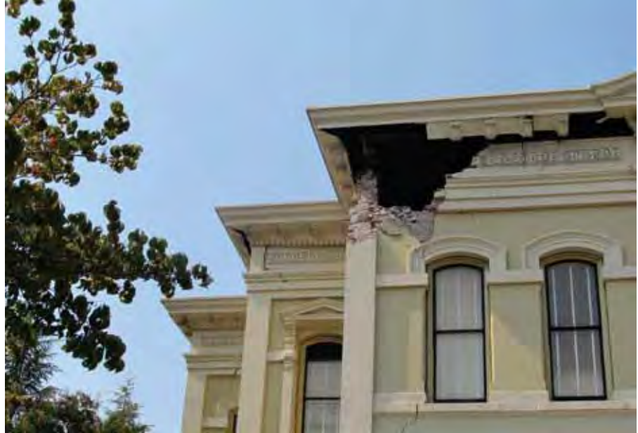
Figure 4-48 Close-up of damage at top of the wall.
