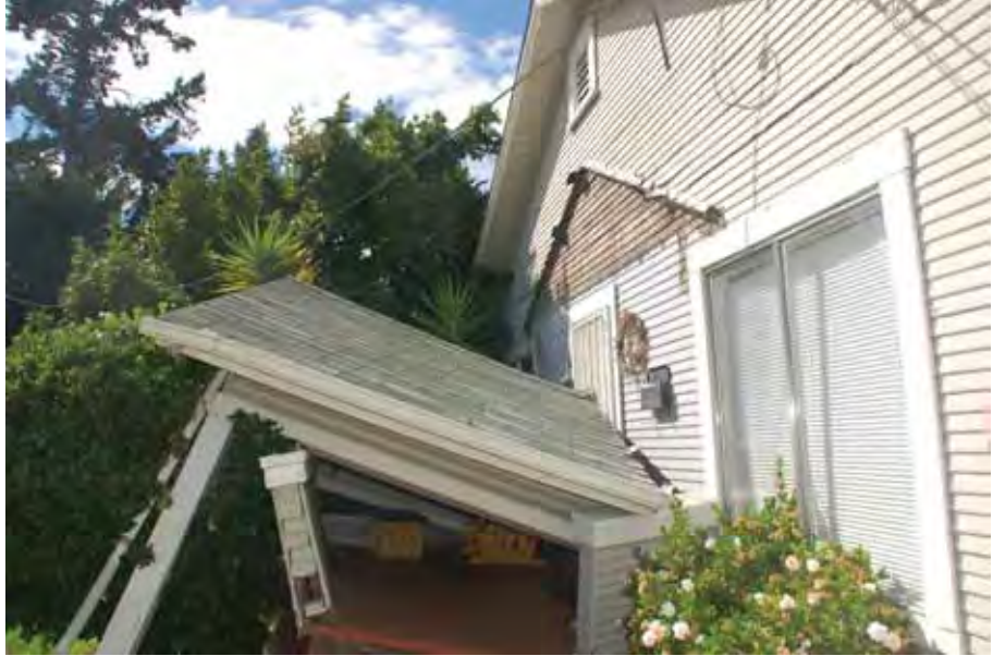
Figure 7-18 Failure of porch due to cripple wall collapse.
