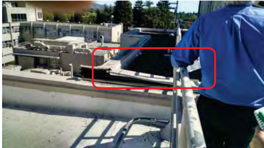
Figure 5-13 Damage to seismic joint flashing between BLD-01654 and BLD-01655.
