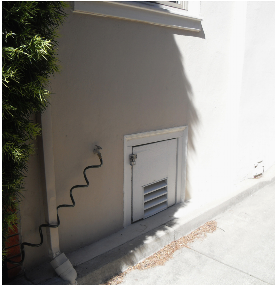
Figure 5-7 Typical crawl space access hatch.
