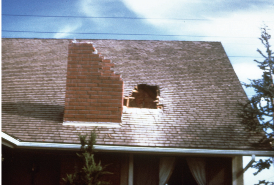
Figure 7-2 Masonry debris from an unreinforced chimney has fallen through the roof into the living spaces (from ATC, 2002).
