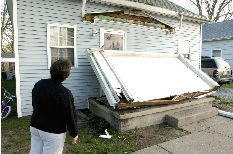
Figure 7-9 Porch roof broken off (and repositioned) in Mt. Carmel, Illinois, by the Richter magnitude 5.2 Mt. Carmel Earthquake in 2008. (Photo credit: Associated Press/Daniel R. Patmore)
