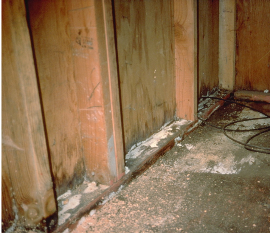
Figure 5-6 Obvious visible decay in a sill plate.
