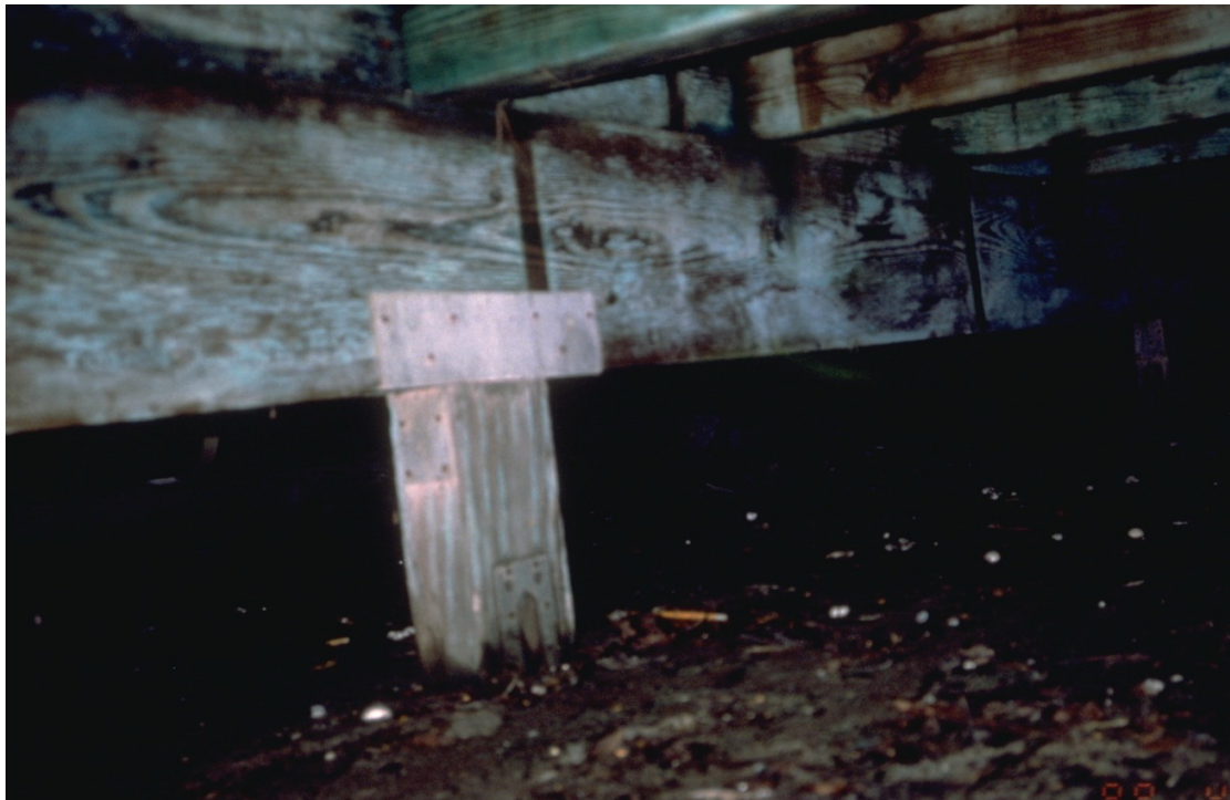
Figure 5-4 Decay of wood framing in damp crawl space.
