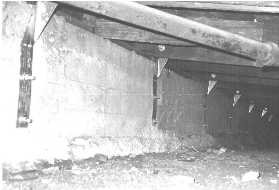
Figure 6-1 A retrofit anchor that is not appropriate for a retrofit to the IEBC Cripple Wall Provisions. Twist strap anchors between the foundation and the floor joists have insufficient strength to resist significant horizontal in-plane shear wall forces.
