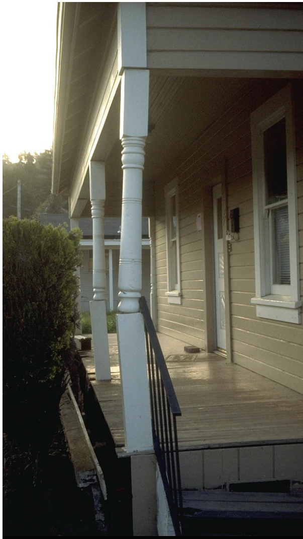
Figure 7-14 Failure of a porch roof support post by hinging at the middle (from ATC, 2002).
