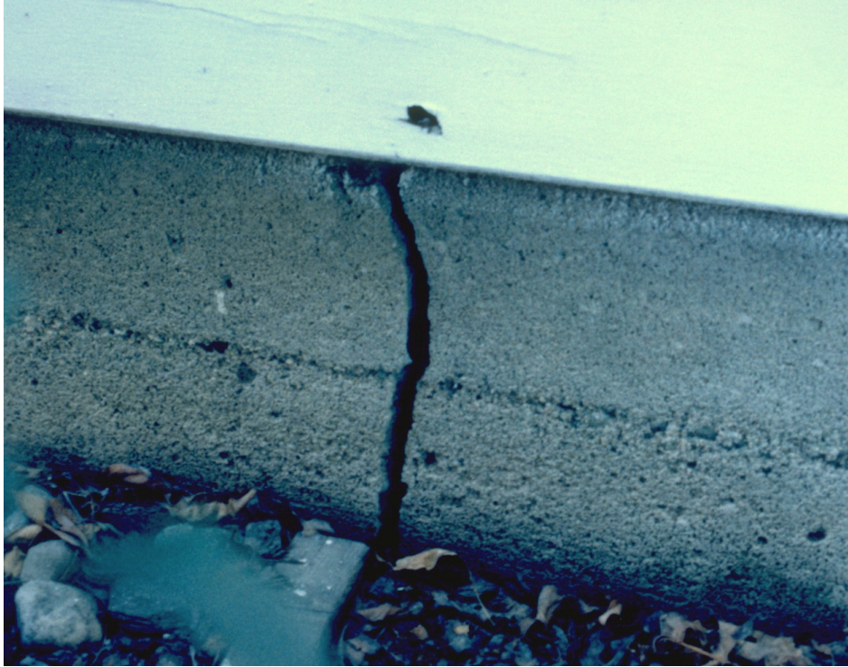
Figure 5-1 Shrinkage crack in unreinforced concrete perimeter footing wall.
