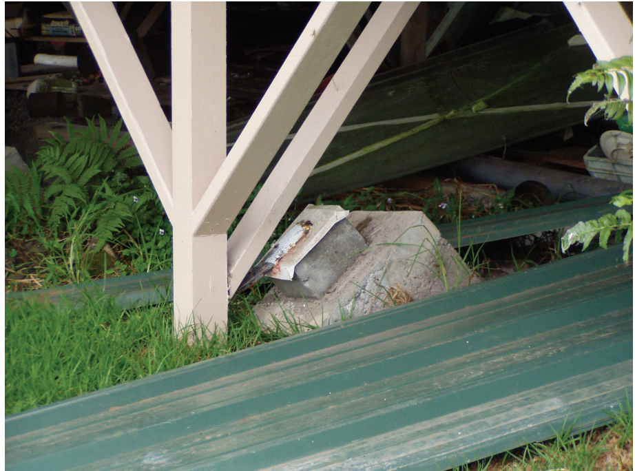
Figure 2-17 Earthquake-damaged perimeter post-and-pier foundation. The diagonally-braced post has overturned the shallow-founded concrete pier footing (from ATC, 2002).
