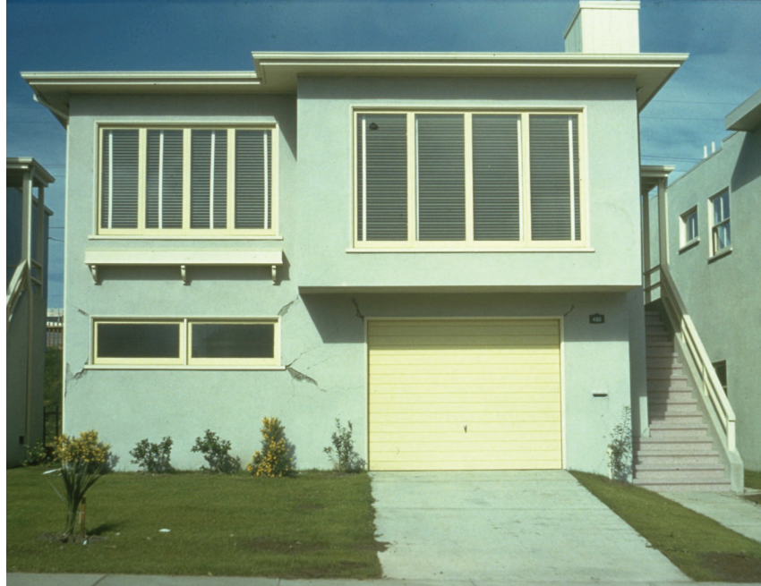
Figure 2-9 Cracking damage at the window to stucco first-floor walls of a two-story slab-on-grade house (from ATC, 2002).
