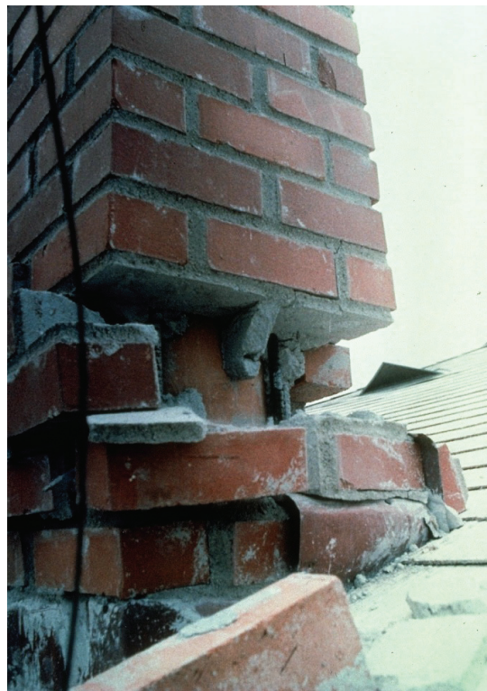
Figure 7-1 Chimney fractured at the roof line, with vertical steel reinforcement visible (from ATC, 2002).
