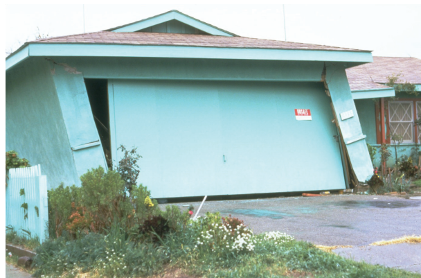
Figure 8-2 Earthquake damage at garage door opening in a one-story house (from ATC, 2002).
