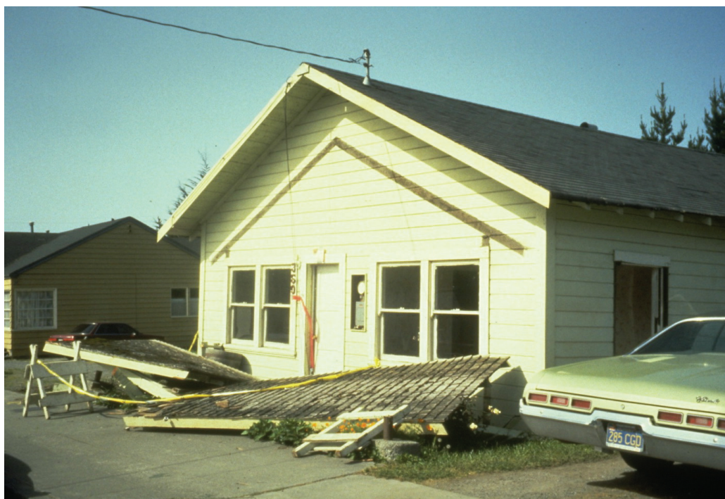
Figure 7-8 Porch roof failure (from ATC, 2002).
