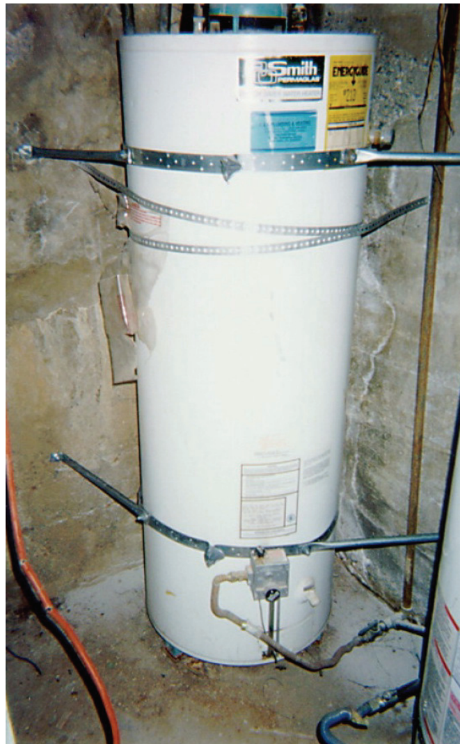
Figure 7-6 Water heater braced with straps and a V-shaped wall-mounted bracket.
