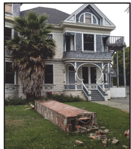
Figure 2: Chimney damaged in the South Napa Earthquake. Photo Credit: Janiele Maffei, CEA
