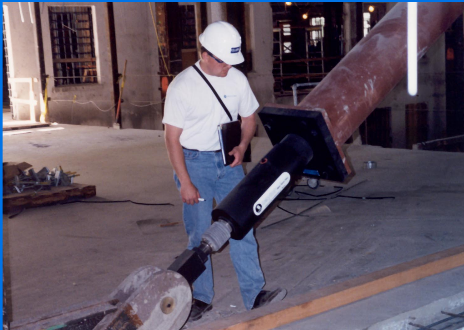
Seismic Damper installed at San Francisco Civic Center Office Building, San Francisco, California Force = 230,000 lbs., Stroke = +/- 4 inches, Production = 292 pieces
