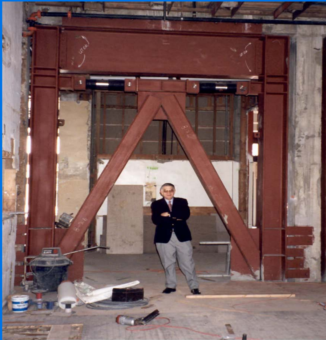
Seismic Dampers installed at the Hotel Woodland, in Woodland, California Force = 100,000 lbs., Stroke = +/- 2 inches Production = 16 pieces
