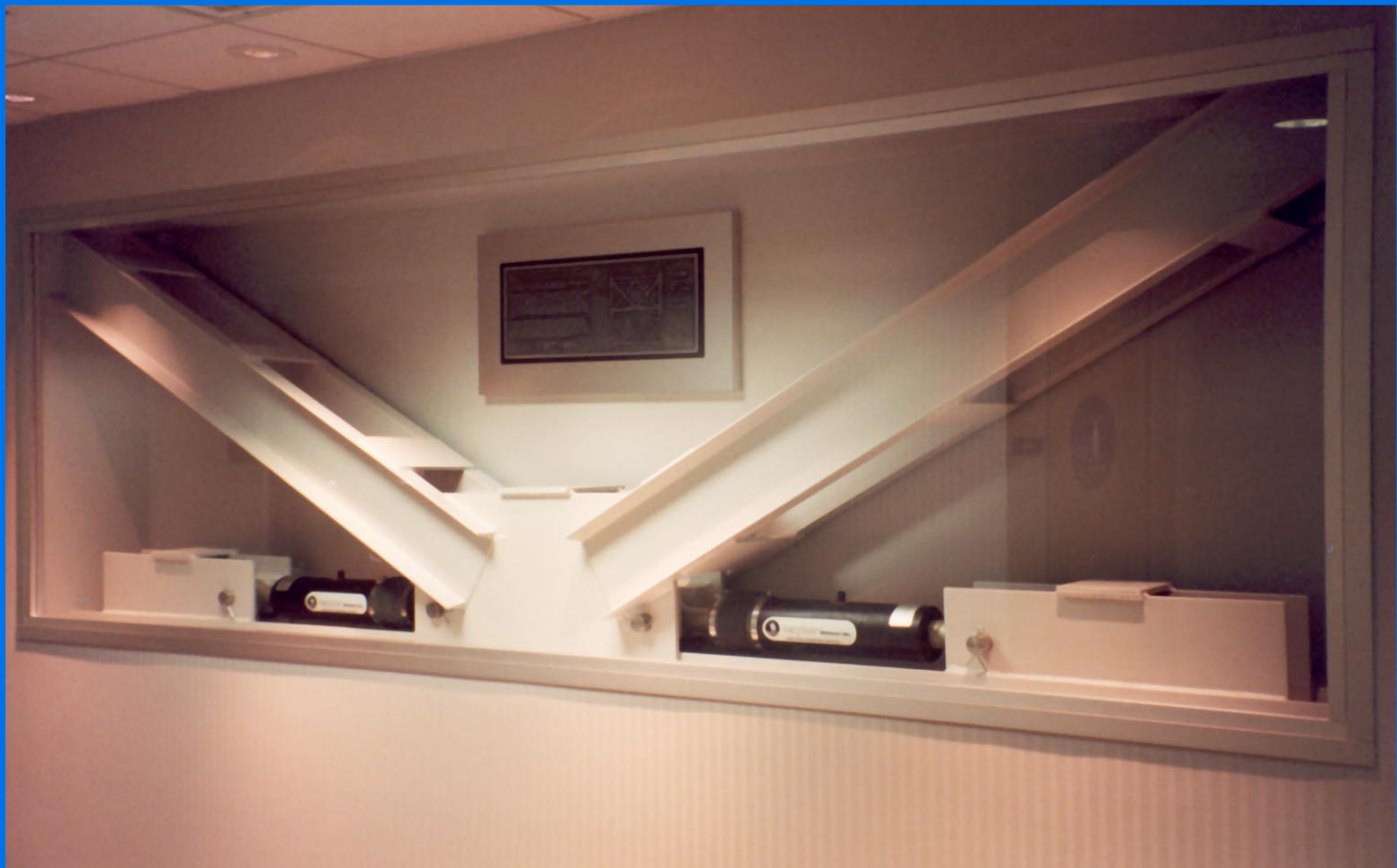
Seismic Dampers installed at Pacific Bell North Area Network Operations Center, Sacramento, California Force = 30,000 lbs., Stroke = +/- 2 inches, Production = 62 Pieces
