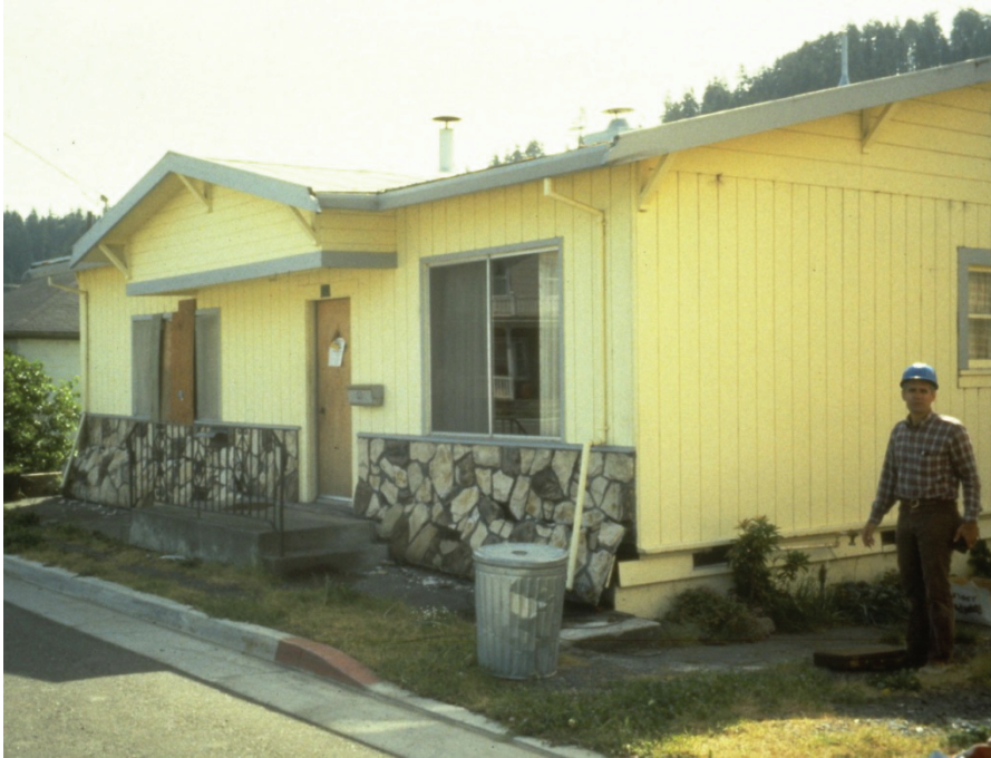
Figure C-10 Damage to a basement-type dwelling where the sill plate slid on the top of the foundation wall (from ATC, 2002a).
