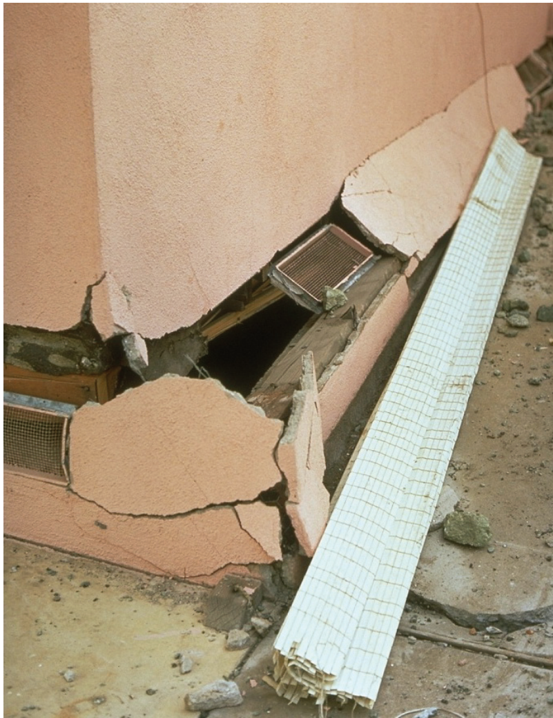
Figure C-5 Typical earthquake damage to a cripple-wall house (from ATC, 2002a).
