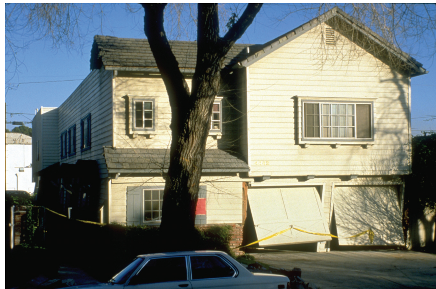
Figure C-16 Damage and racking displacement in the first floor walls (from ATC, 2002a).
