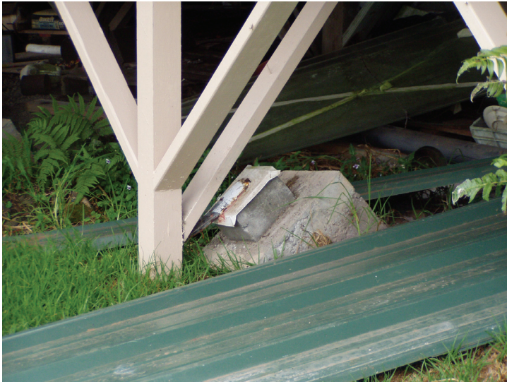
Figure C-13 Earthquake-damaged perimeter post-and-pier foundation (from ATC, 2002a). The diagonally braced post has slid off the pier footing.
