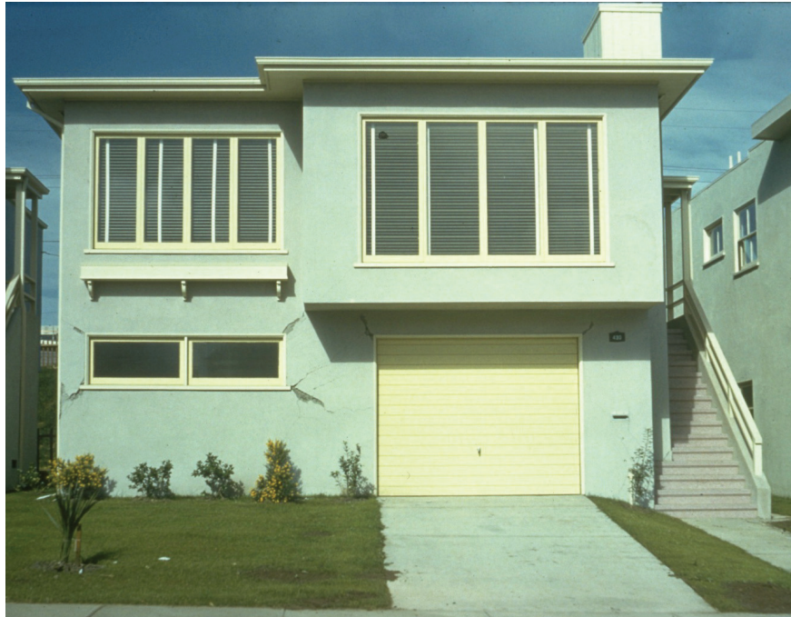
Figure C-15 Cracking damage to stucco first-floor walls (from ATC, 2002a).
