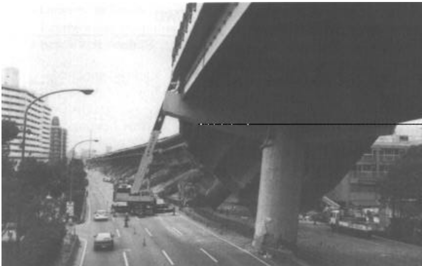
Collapsed portion of Hanshin Expressway, Kobe, Japan. C. Rojahn photo.
