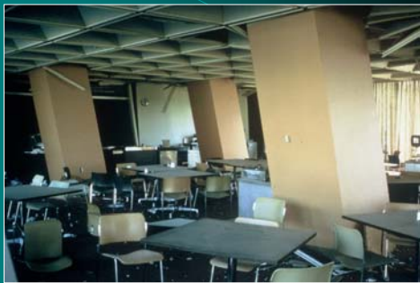
Olive View Hospital 1971 San Fernando Earthquake
