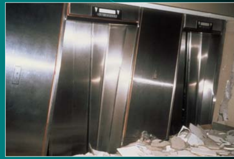
Olive View Hospital 1971 San Fernando Earthquake
