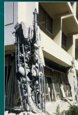
Olive View Hospital 1971 San Fernando Earthquake
