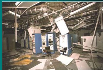
After 1994 Northridge Earthquake
