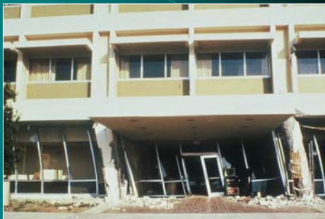
Olive View Hospital 1971 San Fernando Earthquake
