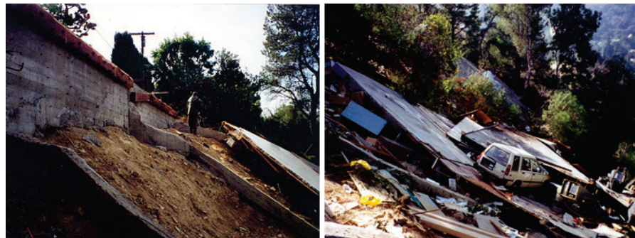
Figure 9-2 Illustrations of hillside dwellings failing by tearing away at the uphill diaphragm connection causing global collapse following the 1994 Northridge, California earthquake. (Photo credit City of Los Angeles.)
