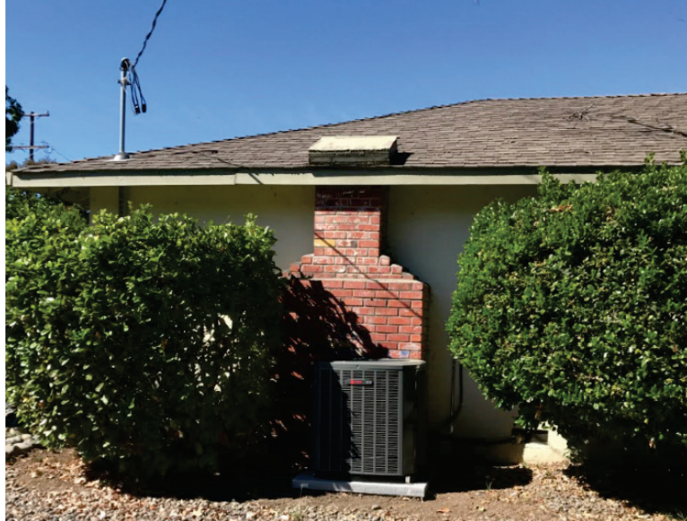
Figure 10-2 Chimney retrofit by removing masonry to the roof level and capped. (Photo by authors).
