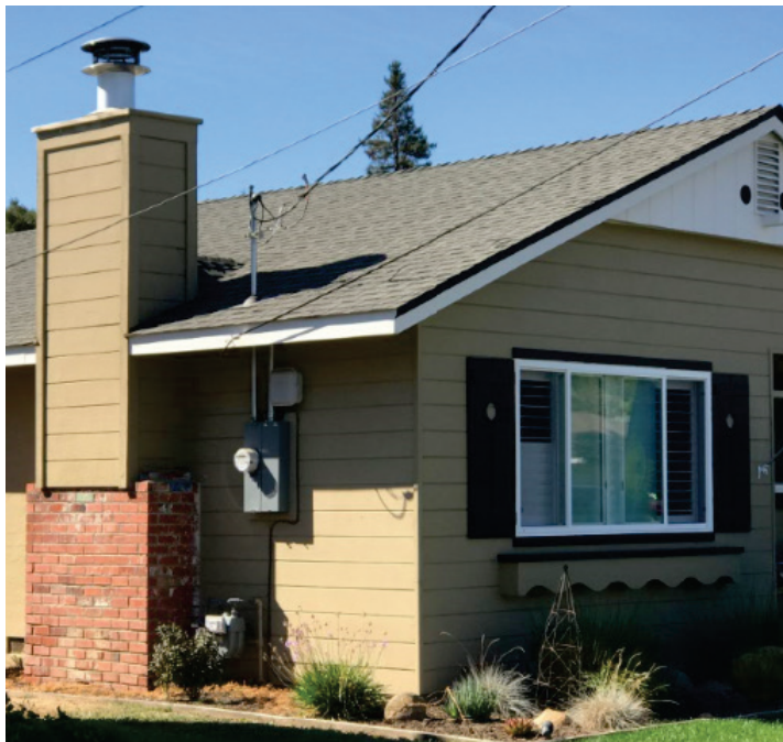
Figure 10-3 Chimney retrofit by removing masonry to the top of the smoke chamber and installing a factory-built metal flue in a light-frame chase. (Photo by authors).
