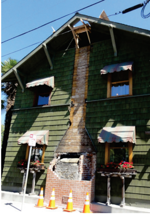
Figure 10-4 Common failure of two-story exterior chimney. (Photo by authors).
