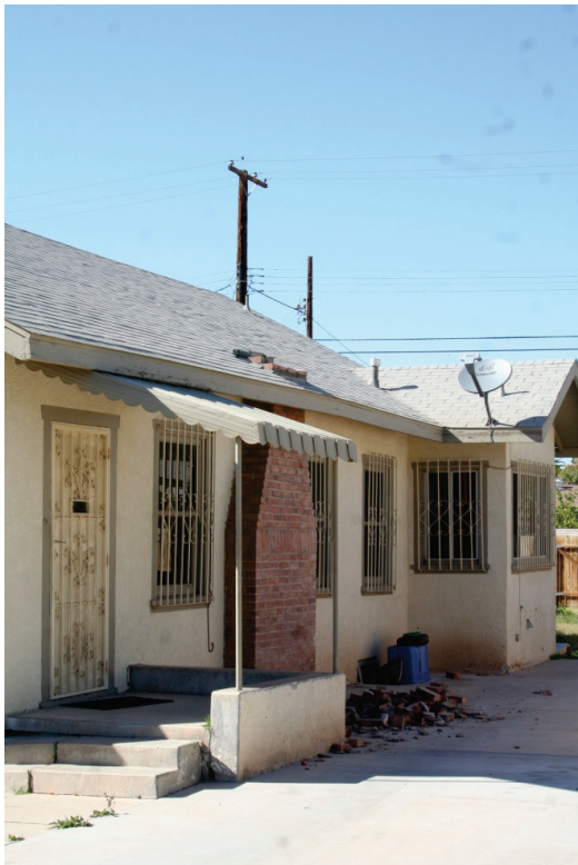
Figure 10-5 Typical failure at roof line. (Photo by authors).
