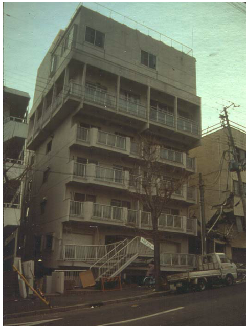
Figure 7: This reinforced concrete building was determined to be stable even though leaning slightly, because of the presence of substantial concrete shear walls on all sides.
