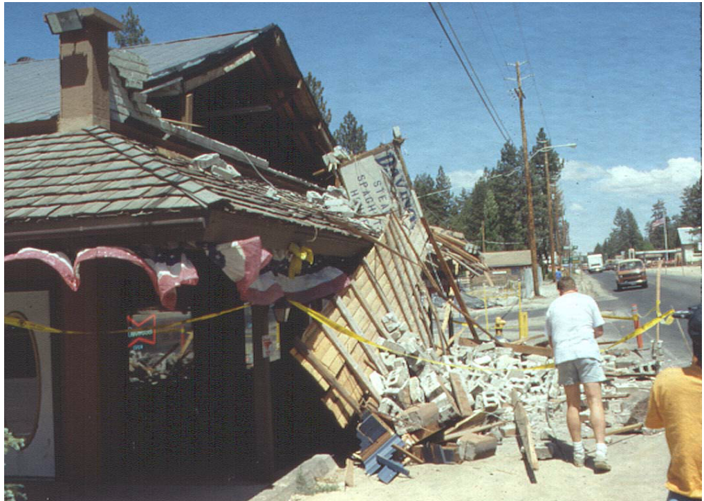
Figure 3: The M 6.2 aftershock of the M 7.5 1992 Landers, California, earthquake caused this gable end wall to collapse.
