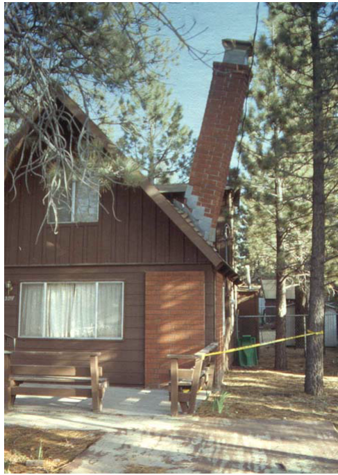
Figure 2: A house with a broken chimney, while posted yellow, RESTRICTED USE, may be entered except for the restricted area.
