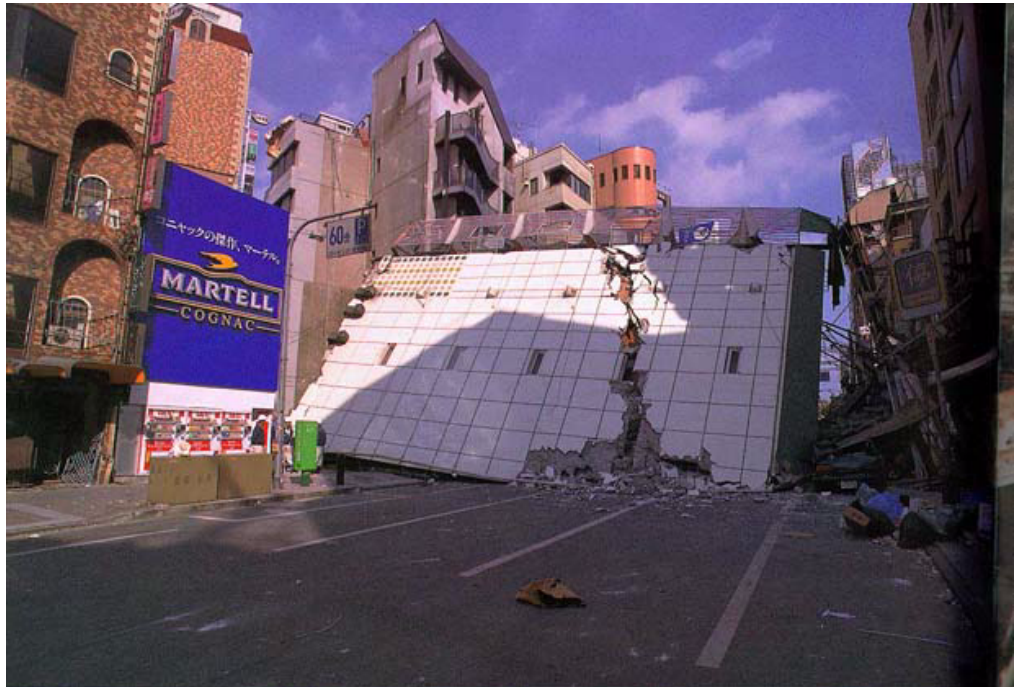
Figure 8: This Kobe office building was unstable after the mainshock and collapsed under its own weight in less than 24 hours.
