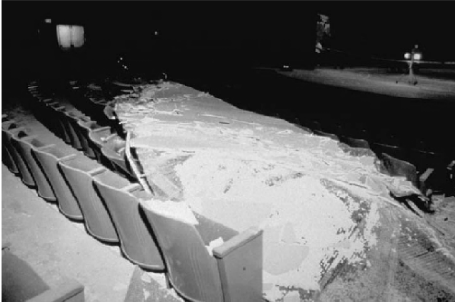
Figure 3. Collapse of heavy plaster ceiling during 1994 Northridge earthquake (EERI photo).
