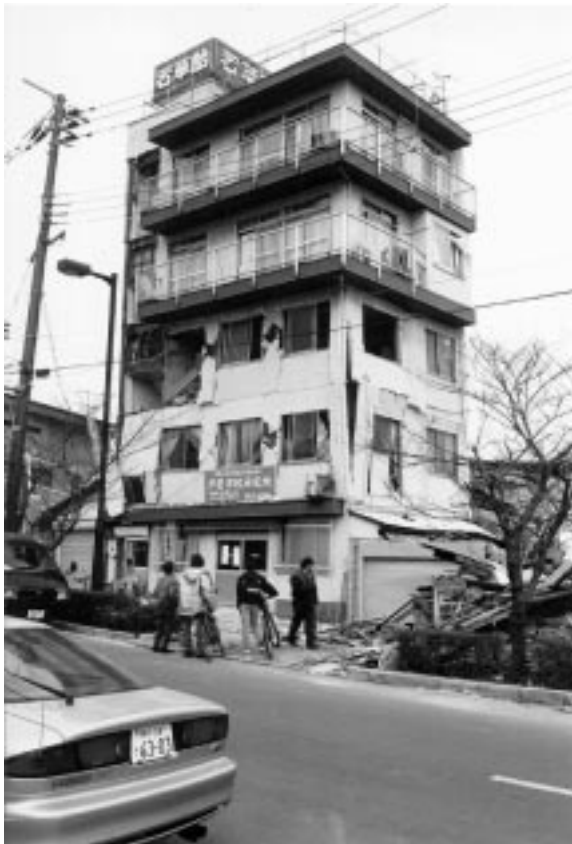
Figure 2. Cladding damage resulting from 1995 Kobe earthquake (C. Rojahn photo).
